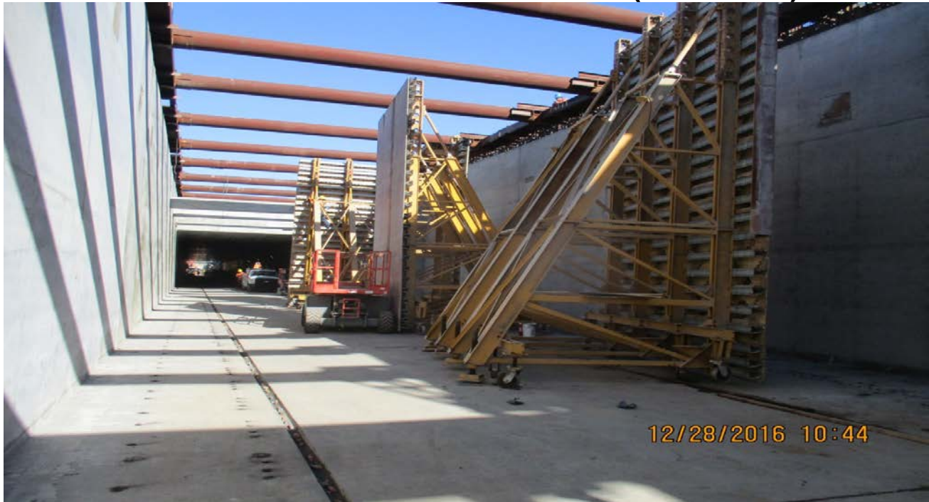
UG#1 – Crew continues with sequential construction at Underground Guide way progressing from South to North. Open cut at strutted U-wall.
