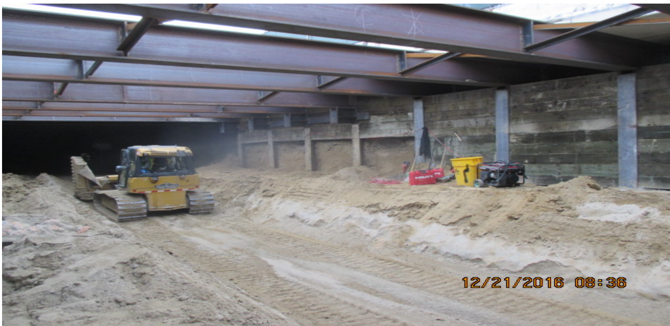
UG#3 – Lagging and excavation activities at 63rd St. UG#3 - Trenching activities for OCS conduits at north portal.
