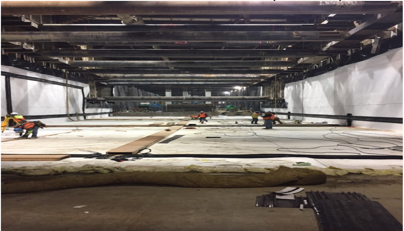
UG#4 – Installation of waterproofing and formwork for protection slab at north portal.
