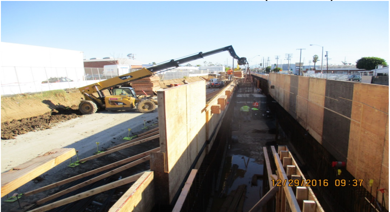
WESTCHESTER STATION – Rebar and formwork for Hindry station north bound platform stem walls.
