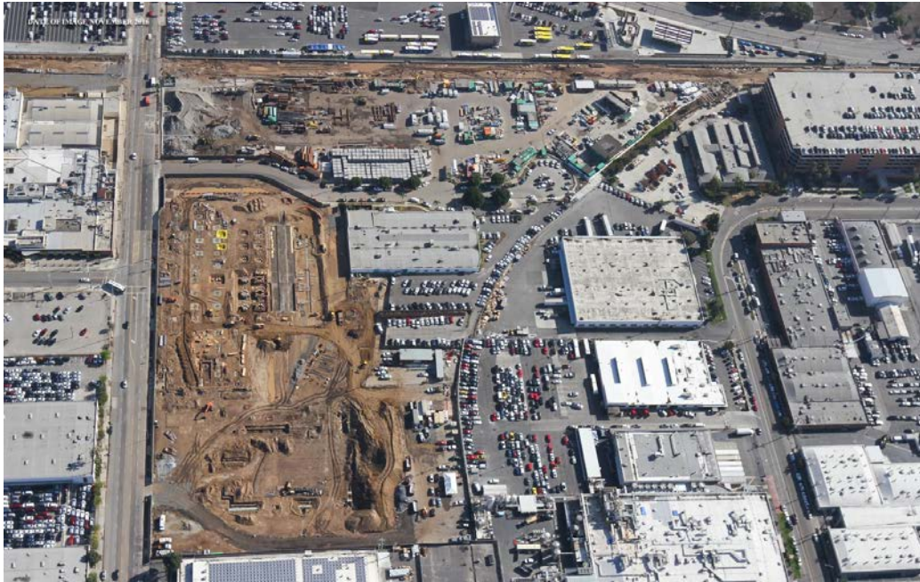
SOUTHWESTERN YARD: DIVISION 16 - Aerial view of construction site on the left and the alignment work at the top.
