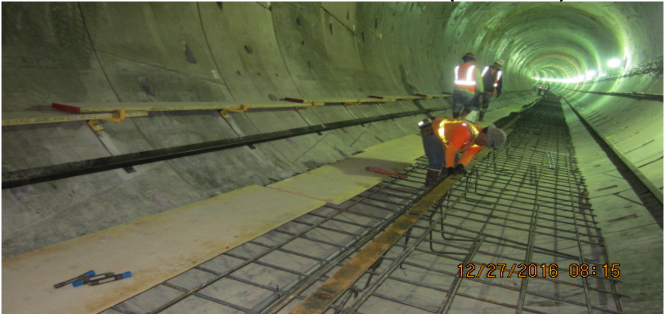
TUNNELING – Installation of gutter drain formwork at SB tunnel to accommodate tunnel invert work.
