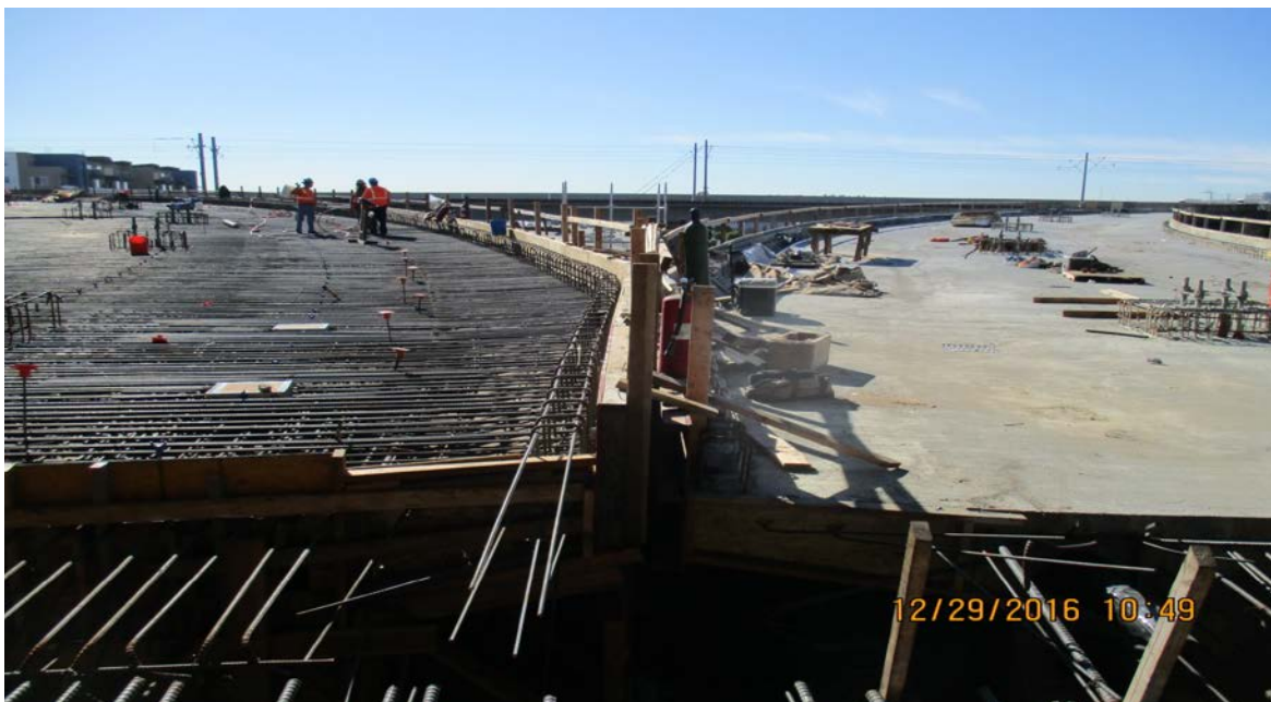
GREENLINE UNDERPASS – Wye junction at Green line: Frame 1 (left) and Frame A.
