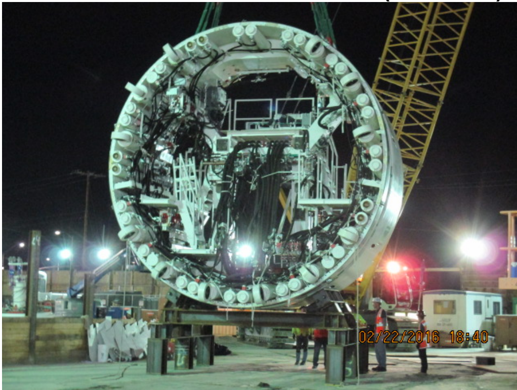
EXPOSITION/CRENSHAW STATION – Lowering of mid-shield of Tunnel Boring Machine (TBM) into Expo station
