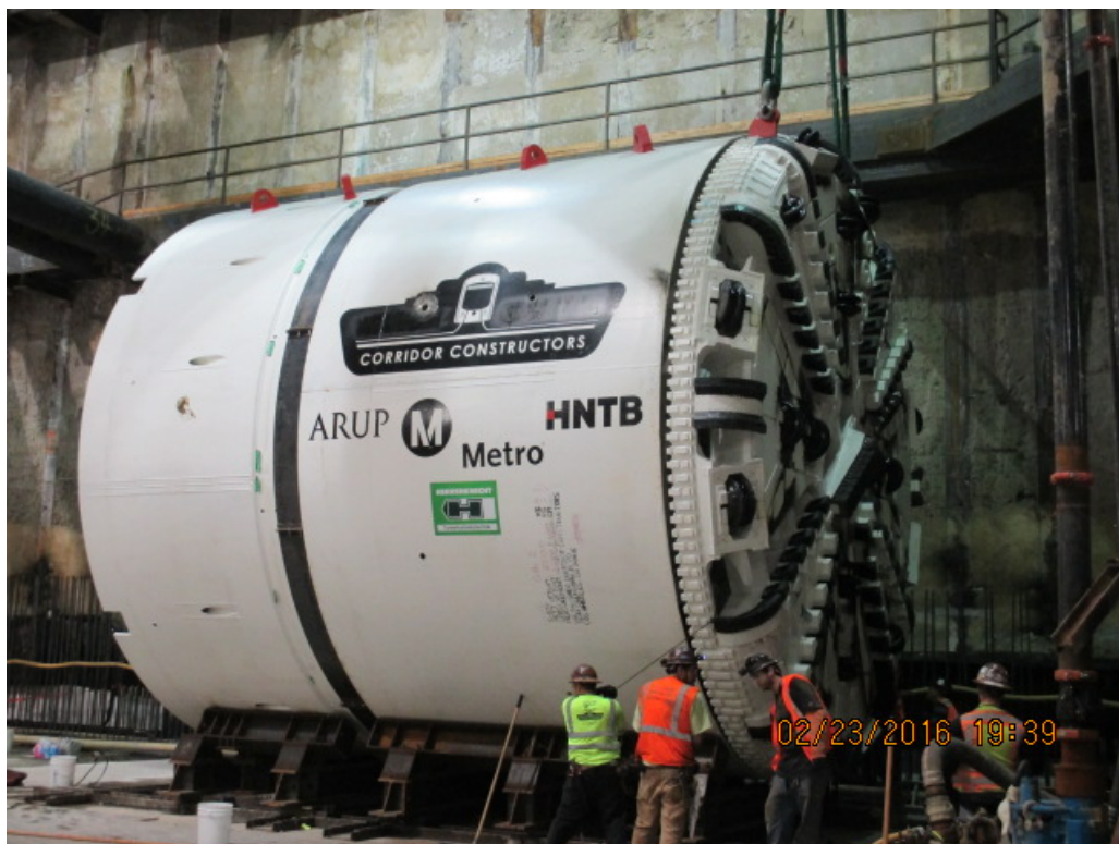
EXPOSITION/CRENSHAW STATION – Attaching Tunnel Boring Machine (TBM) cutter head to the front shield.
