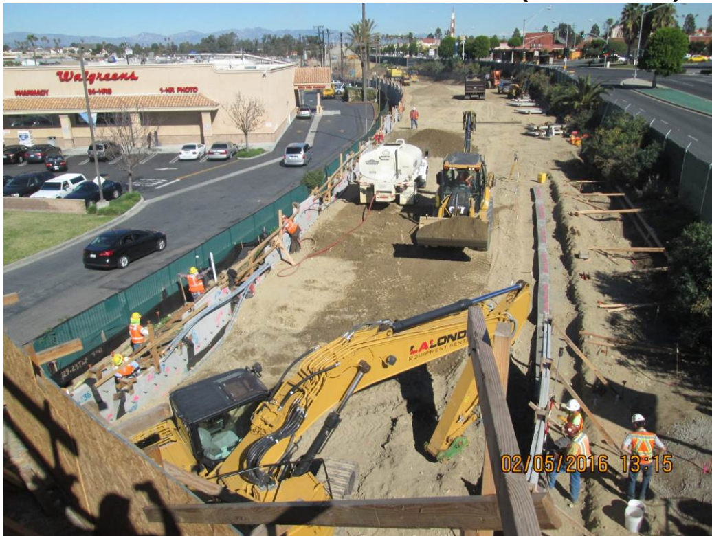
MSE WALL 202L&R - Crews continue to work on subgrade preparation, leveling pads, precast panel erection, strap placement and embankment backfill.
