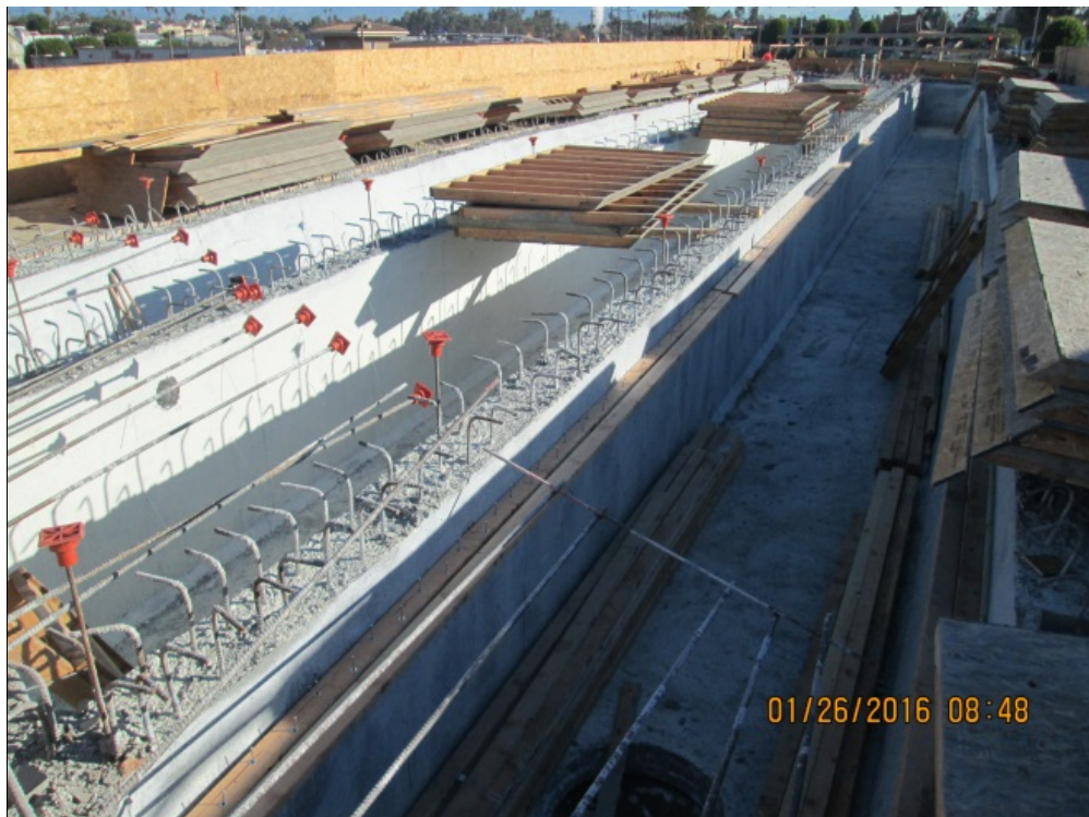
LA BREA BRIDGE: Stem and soffit pour complete. Deck pour scheduled to take place in two weeks followed by post-tensioning.
