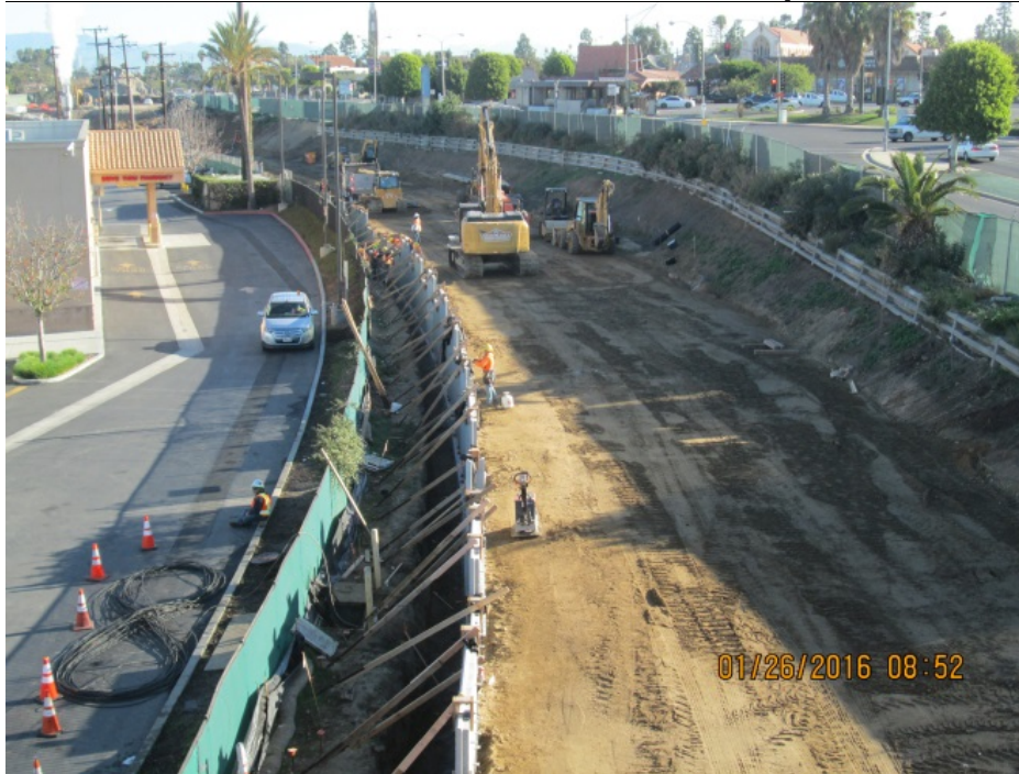
MSE WALL 202L&R: Crews continue to work on subgrade preparation and leveling pads for MSE 202L&R. Crews have begun to work on precast panel erection and strap placement/backfill for 202L.
