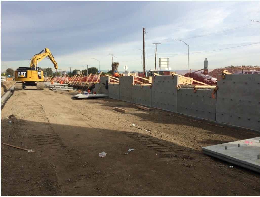
MSE Wall 17L&R (Mechanically Stabilized Embankment): Precast Panel placement begins. Leveling pads and subgrade preparation nearly complete.
