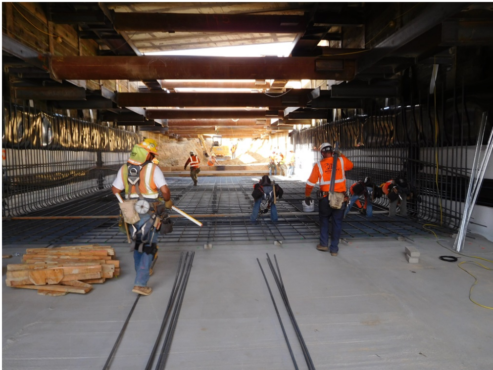
UG#1- Finished installing bracing and lagging beneath 104 th Street temporary deck bridge.
