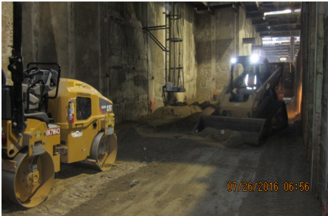
MARTIN LUTHER KING JR. STATION - Backfill and compaction of west bump out wall.
