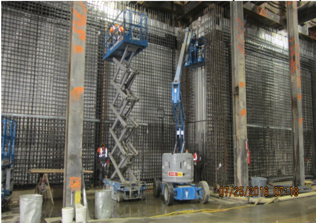
EXPOSITION/CRENSHAW STATION - Installation of rebar for east lower wall D-29 thru D-31.
