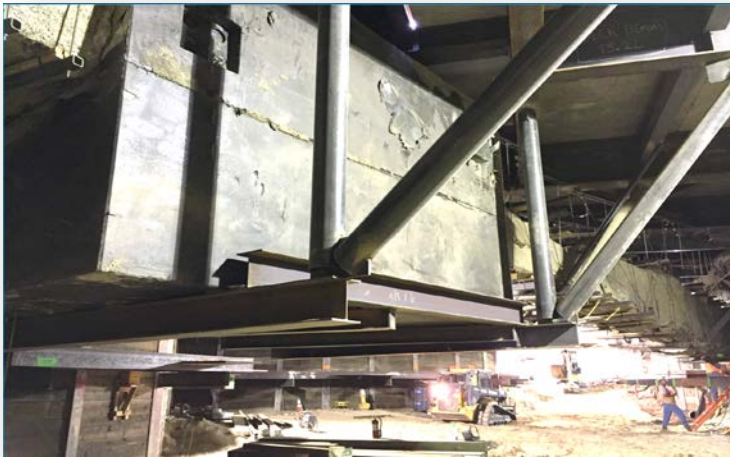
Hanging Utilities under Wye
