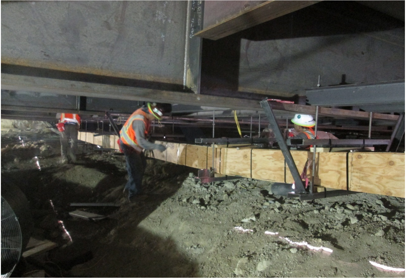
C1045 Contractor Hanging in Place Telecommunications Duct Bank under the Street Decking at Wilshire/La Brea Station
