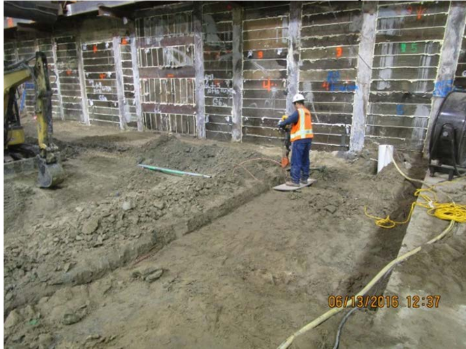
LEIMERT PARK STATION – Installation of grounding grid in preparation for mudslab placement.
