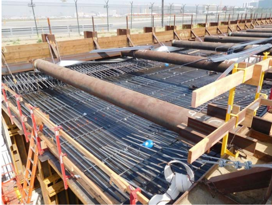
UG#1 – Roof slab rebar installation for the cut and cover tunnel section.
