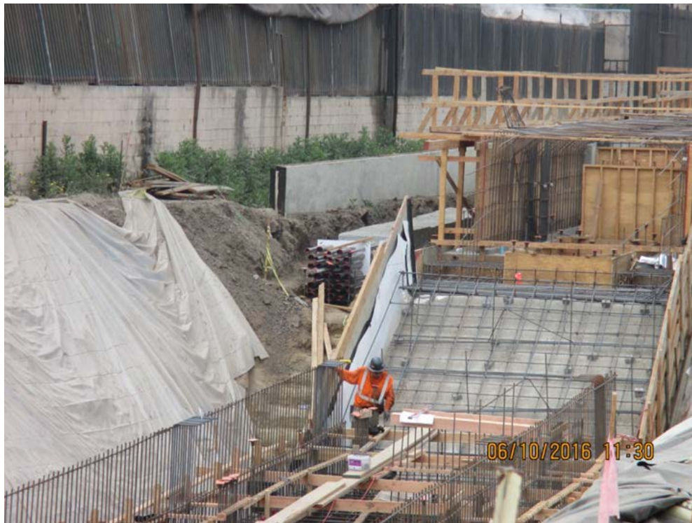
FAIRVIEW HEIGHTS STATION – Crews continue with MEP embed installation for the TC&C room invert. Poured the station platform footing and stem walls.
