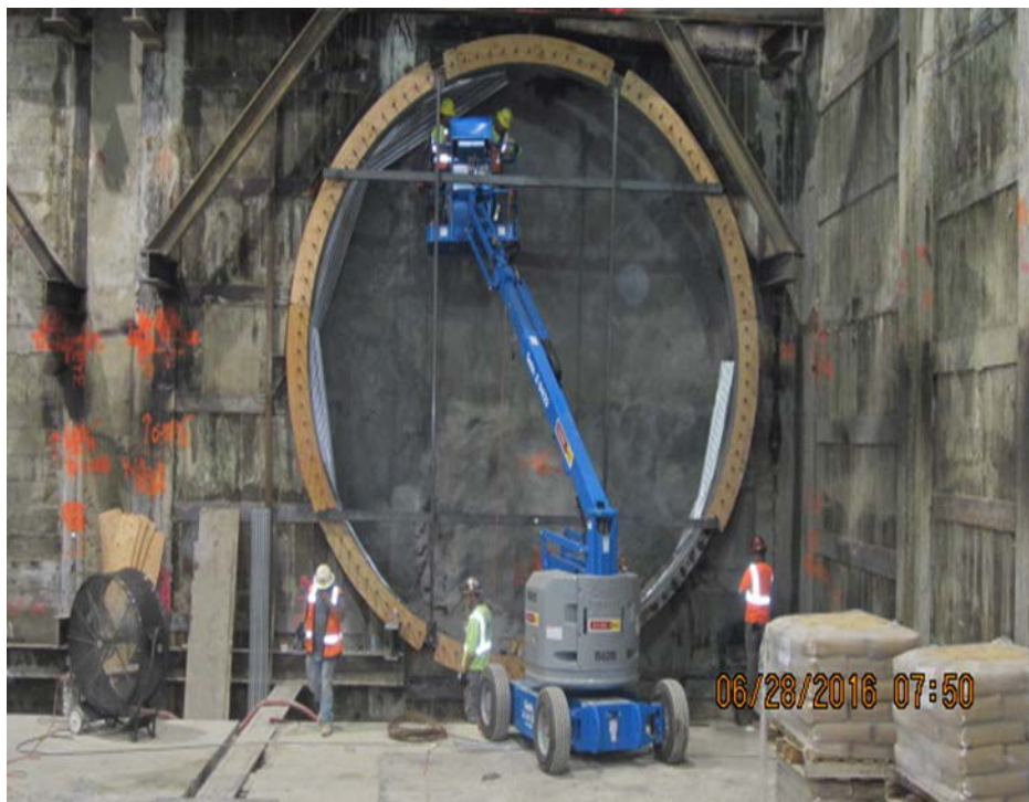
MARTIN LUTHER KING JR. STATION – Installation of southbound tunnel portal seal at south hammerhead.
