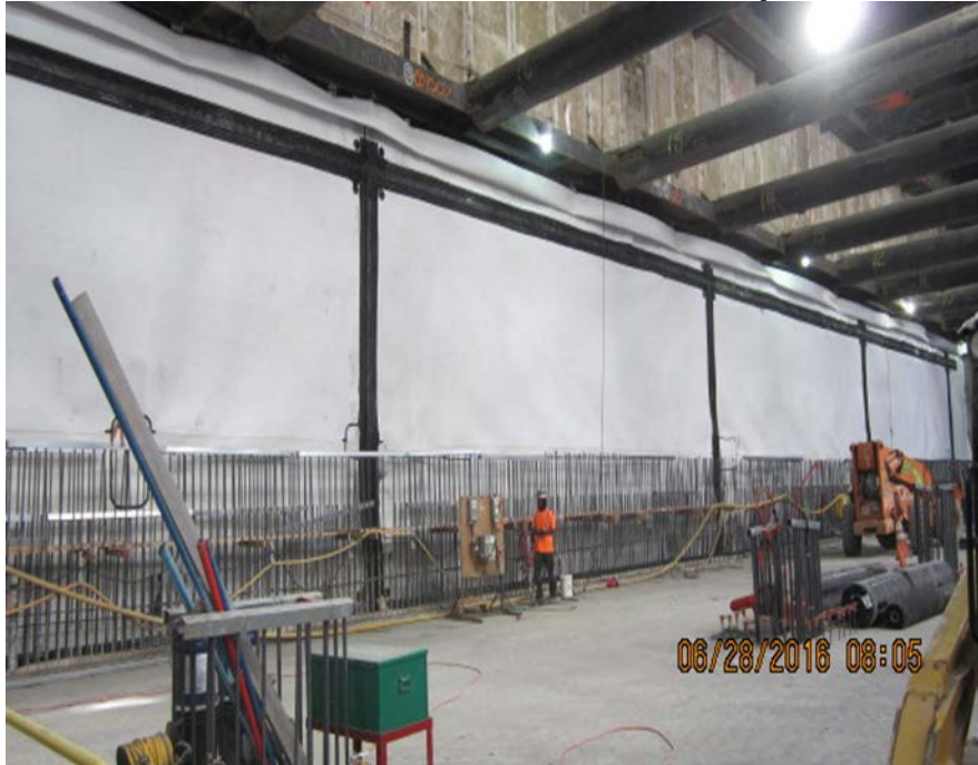
MARTIN LUTHER KING JR. STATION – Installation of geotextile membrane at the station.
