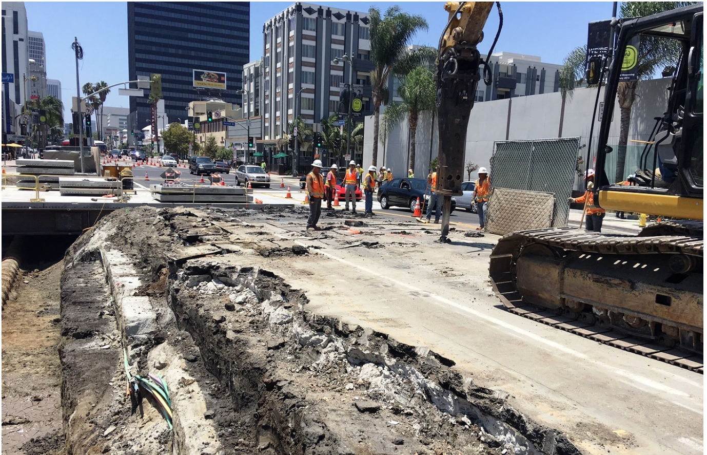
C1045 Contractor Preparing for 3 rd Weekend Closure at Wilshire/La Brea Station to Install Deck Beams and Street Decking
