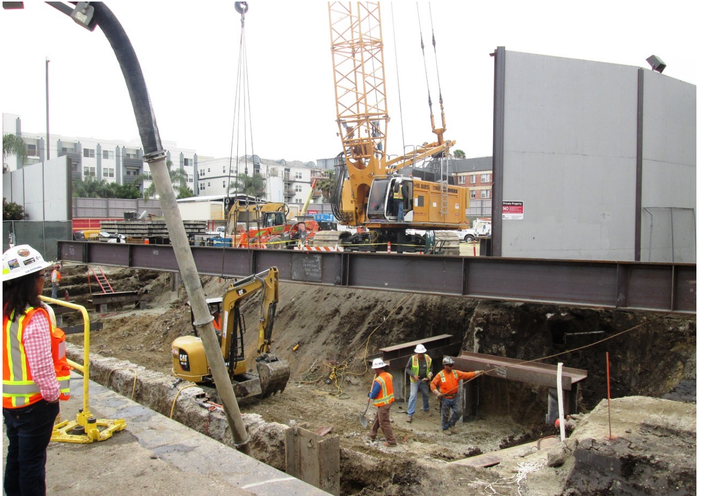
C1045 Contractor Installing Deck Beam during the 1 st of 22 Weekend Closures at Wilshire/La Brea Station
