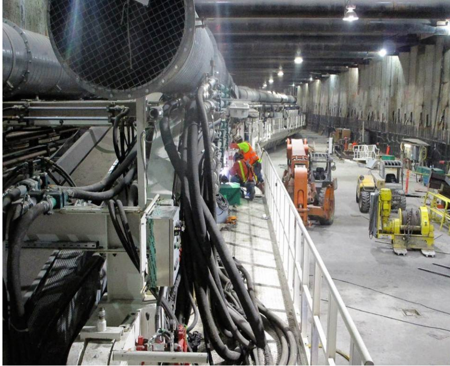
EXPOSITION STATION – Looking north from the TBM toward the trailing gear gantries
