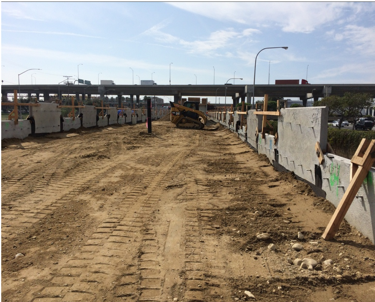
MSE WALL 17L&R (Mechanically Stabilized Embankment) - Precast Panel erection, galvanized strap placement, embankment backfill and compaction testing continue.
