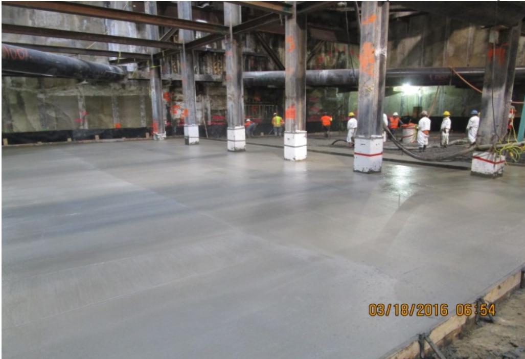
MARTIN LUTHER KING JR. STATION – Placement of mudslab at the north end of station box
