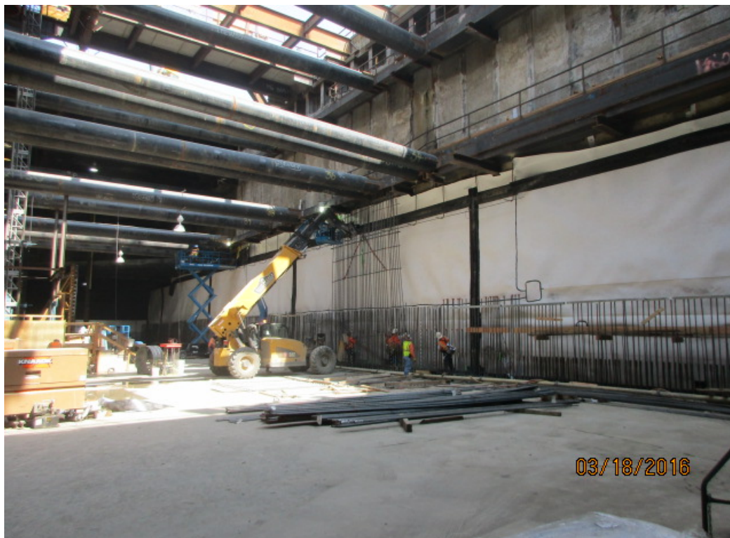
EXPOSITION STATION – Installation of rebar for lower wall placement along the east wall
