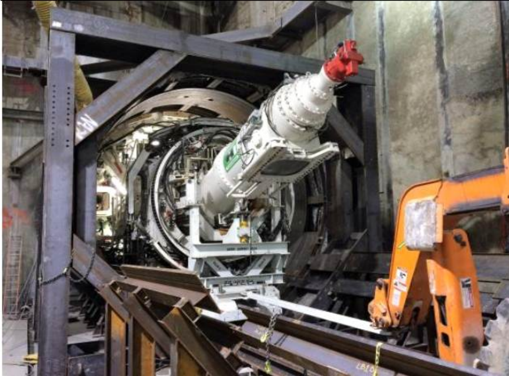
EXPOSITION STATION – Screw conveyor and ring erector in place at the southbound tunnel
