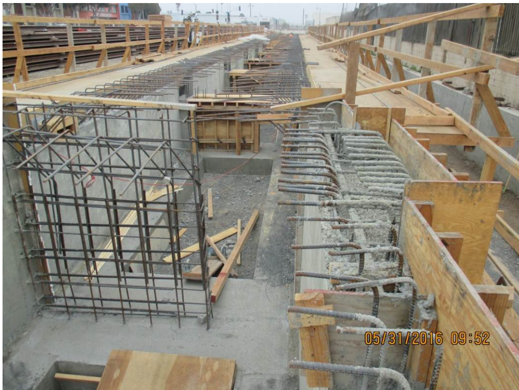
FAIRVIEW HEIGHTS STATION - Crews installed MEP embeds for the TC&C room invert. Crews poured the station platform footing and stem walls.
