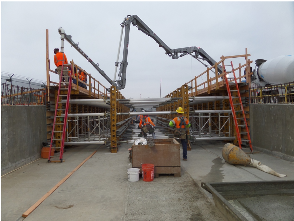
UNDERGROUND GUIDEWAY 1 - Crews continue with sequential construction at Underground Guideway 1, progressing from south to north.
