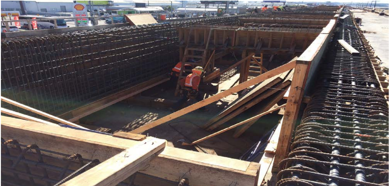
AVIATION/CENTURY BRIDGE – Formwork and rebar installations ongoing for the girders and beams of the aerial station platform.
