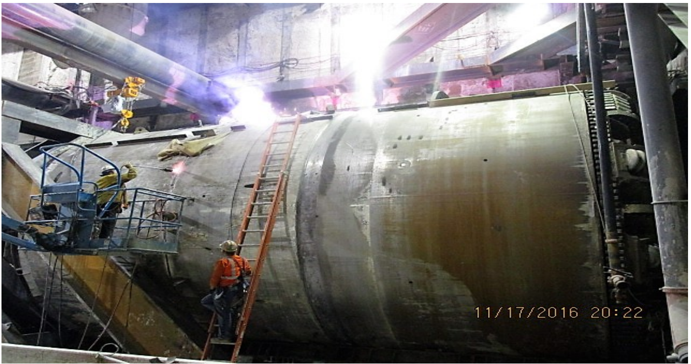
TUNNELING – Welding of the TBM mid-shield/tail shield joint at NB tunnel portal.
