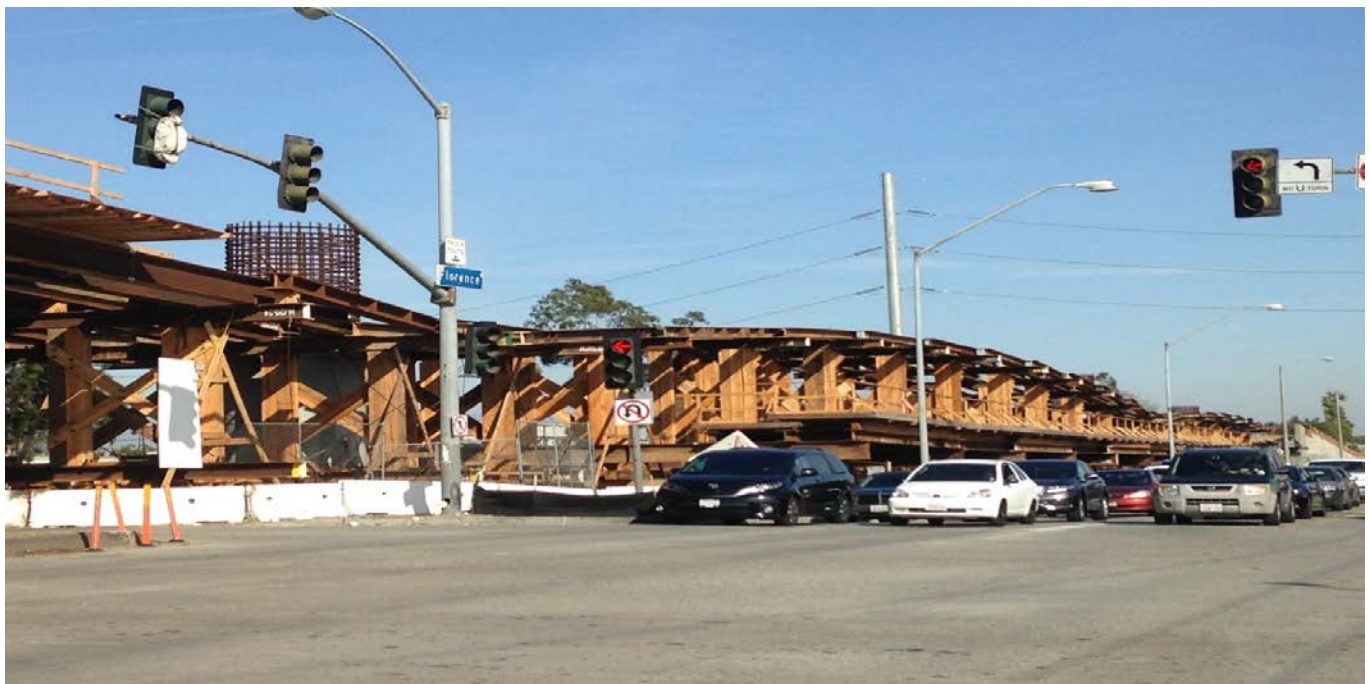
(AG-5) I-405 Bridge – Bridge superstructure falsework erection 90% complete. Crews commenced rolling soffit construction in frame 1.
