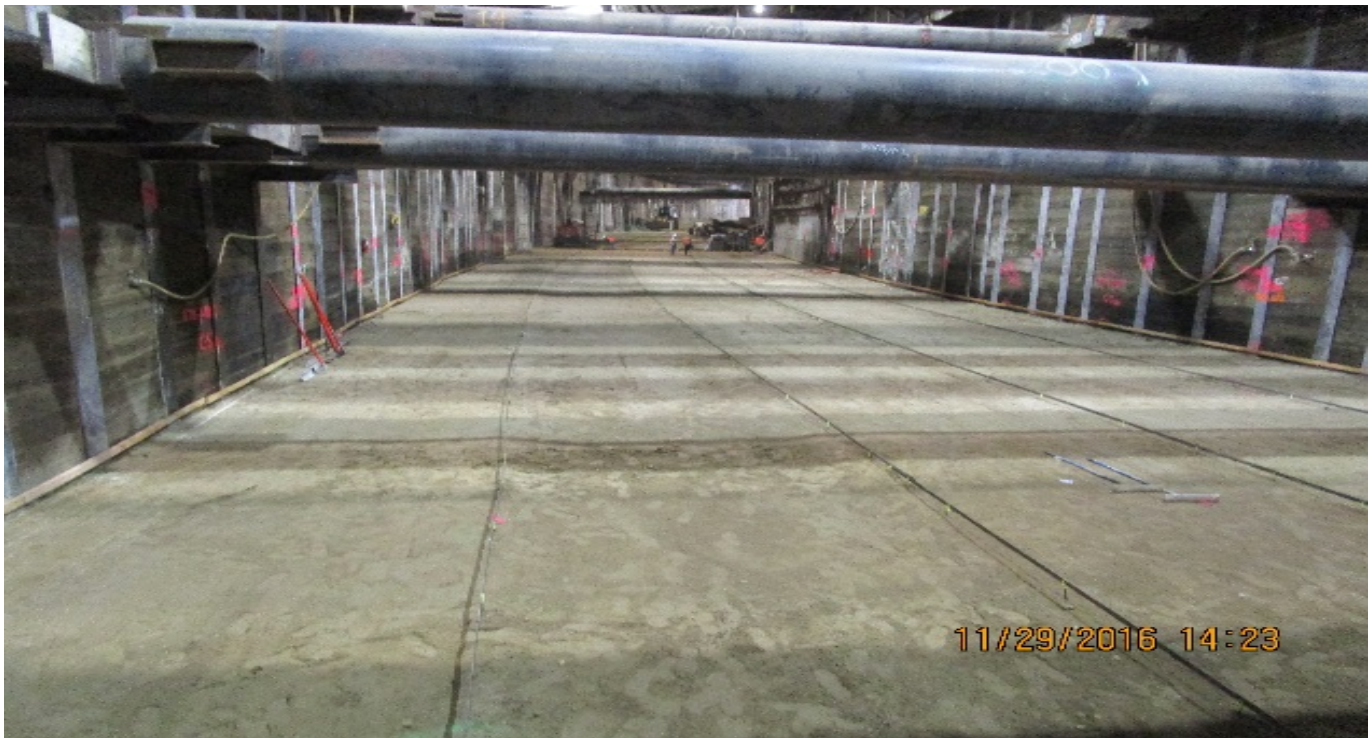
UG#4 – Preparing grade for mud slab placement at north end of UG4.
