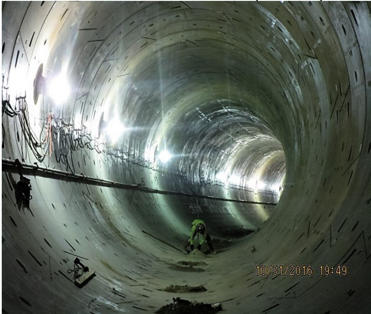
TUNNELING – Removed temporary rail and vent lines to prepare for invert pour of completed tunnel.
