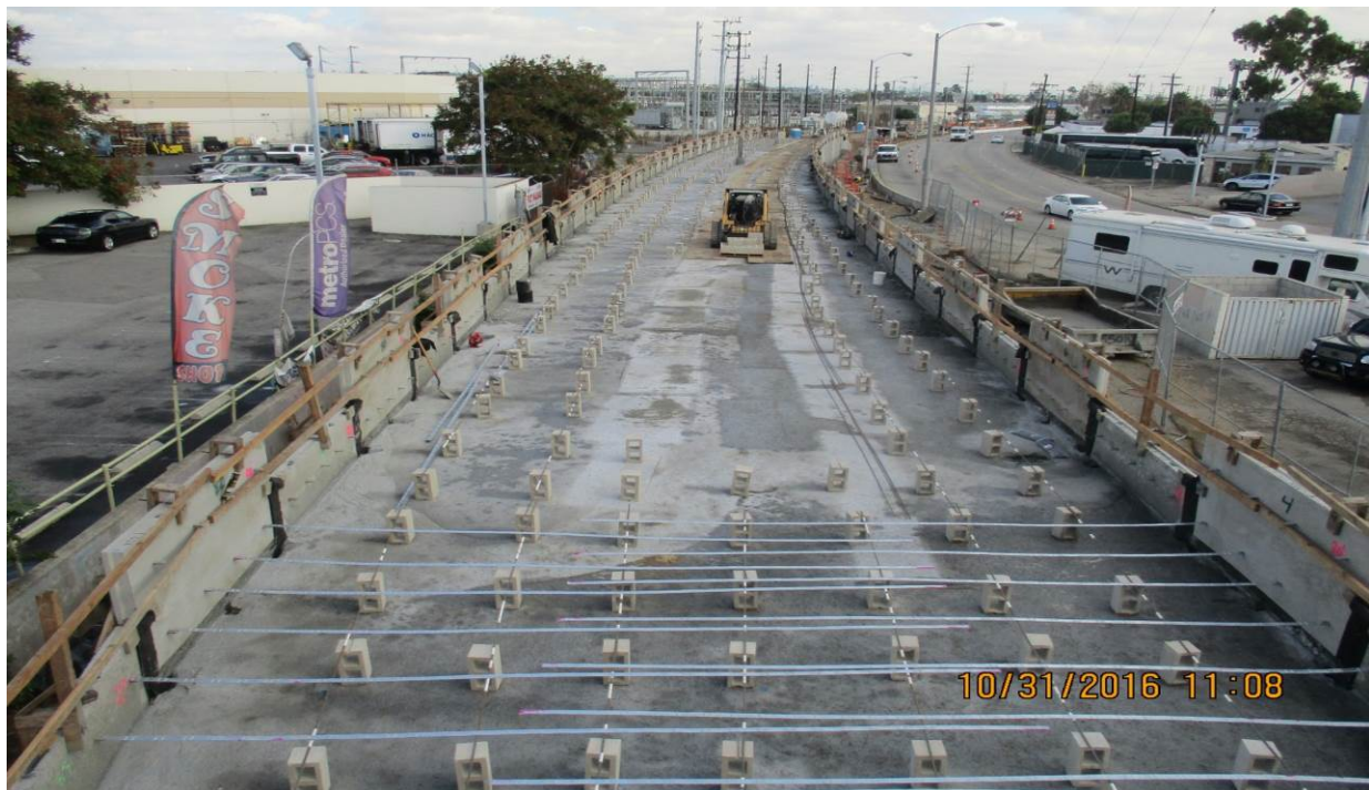
MSE 122 L & R (North of Manchester Blvd.) – Crews continued with sequential construction of the LCC MSE wall erecting precast panels and setting/anchoring the galvanized reinforcement straps.
