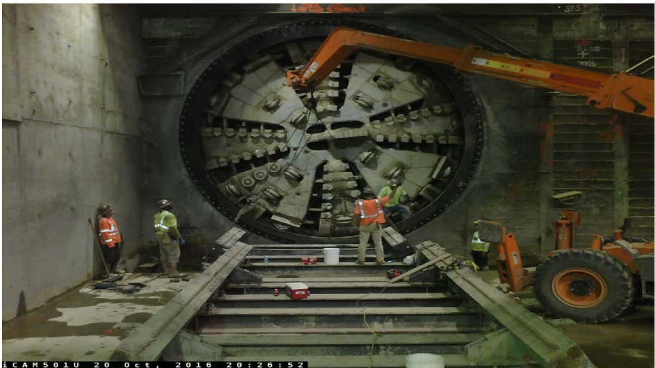
TUNNELING – After TBM breakthrough contractor starting to remove TBM and will reposition back to Exposition/Crenshaw Station for start of 2 nd tunnel leg.
