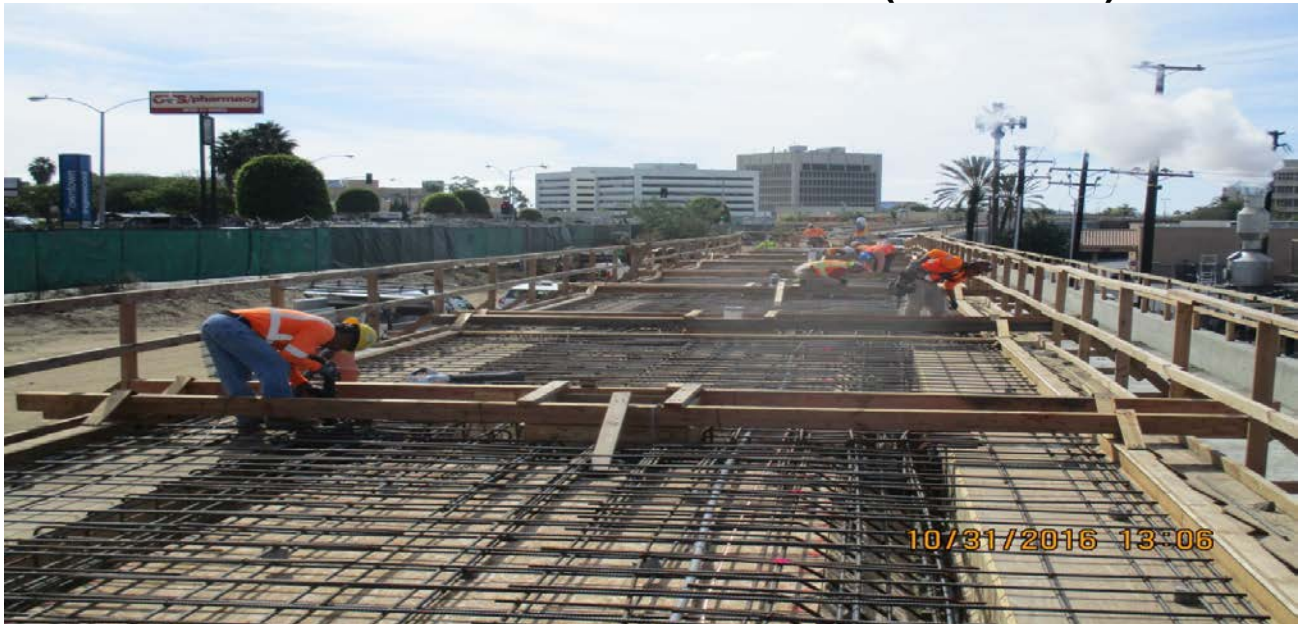
LA BREA BRIDGE -Crews prepped the platform deck and formed bulkheads for the upcoming concrete placements.
