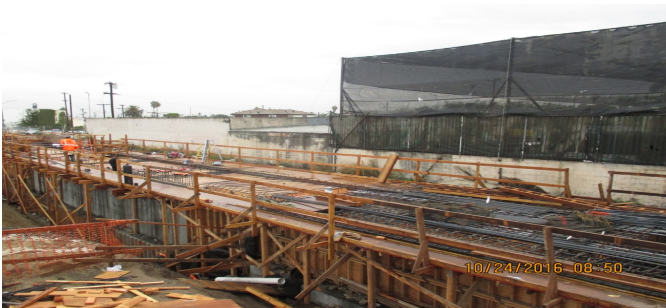
FAIRVIEW HEIGHTS STATION – Crews continued with rebar and formwork installations for the platform deck and through-girders as well as deck MEP embeds.
