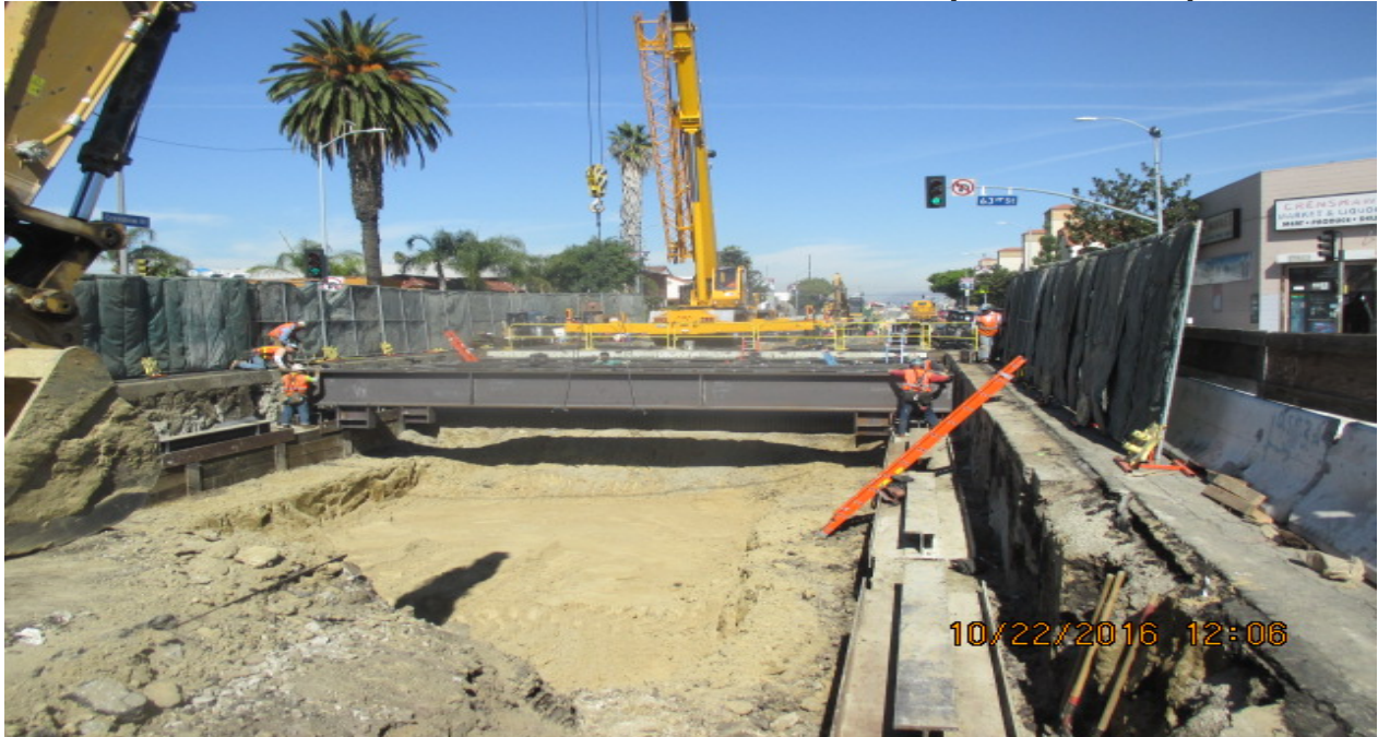
UG#3 – Completed placing deck beams and deck panels south of 63rd Street.
