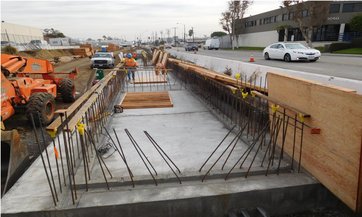
WESTCHESTER STATION – Crews cured the recently placed station footing and continued with rebar and formwork installations for the NB and SB station platform stem walls.
