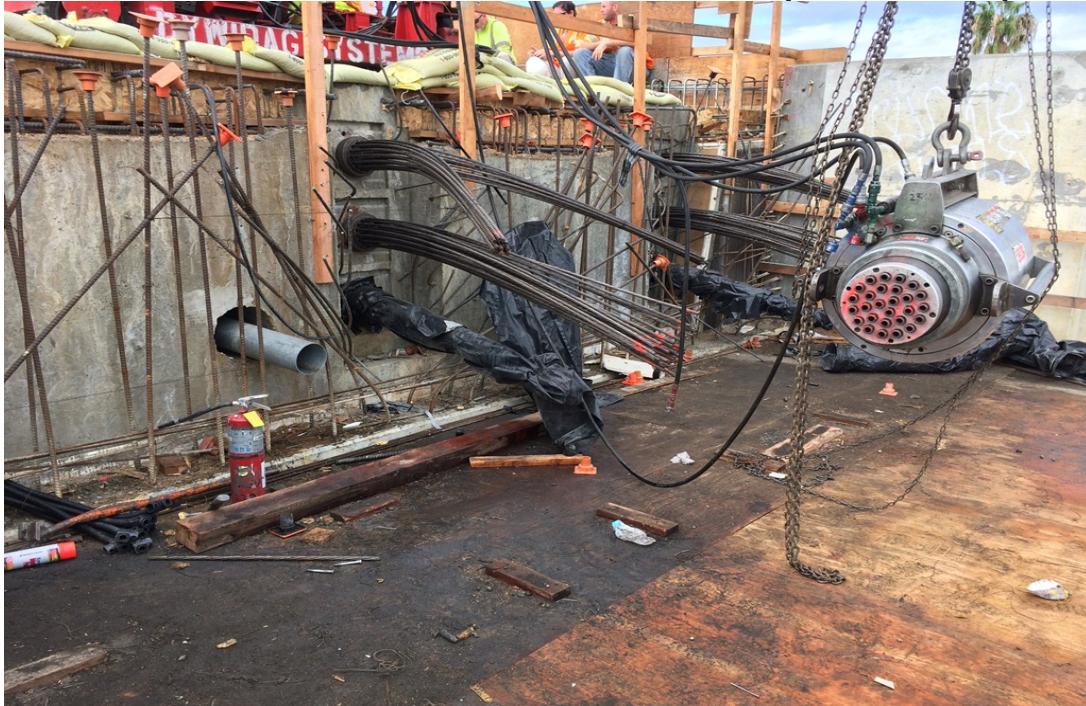
MANCHESTER BRIDGE – Bridge deck concrete placement complete. Subcontractor completed post tensioning stressing operations.
