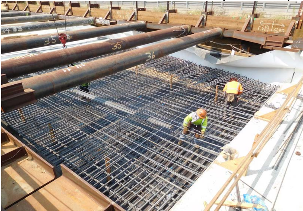
104 th STREET – Rebar installation for a portion of the cut and cover tunnel roof slab.
