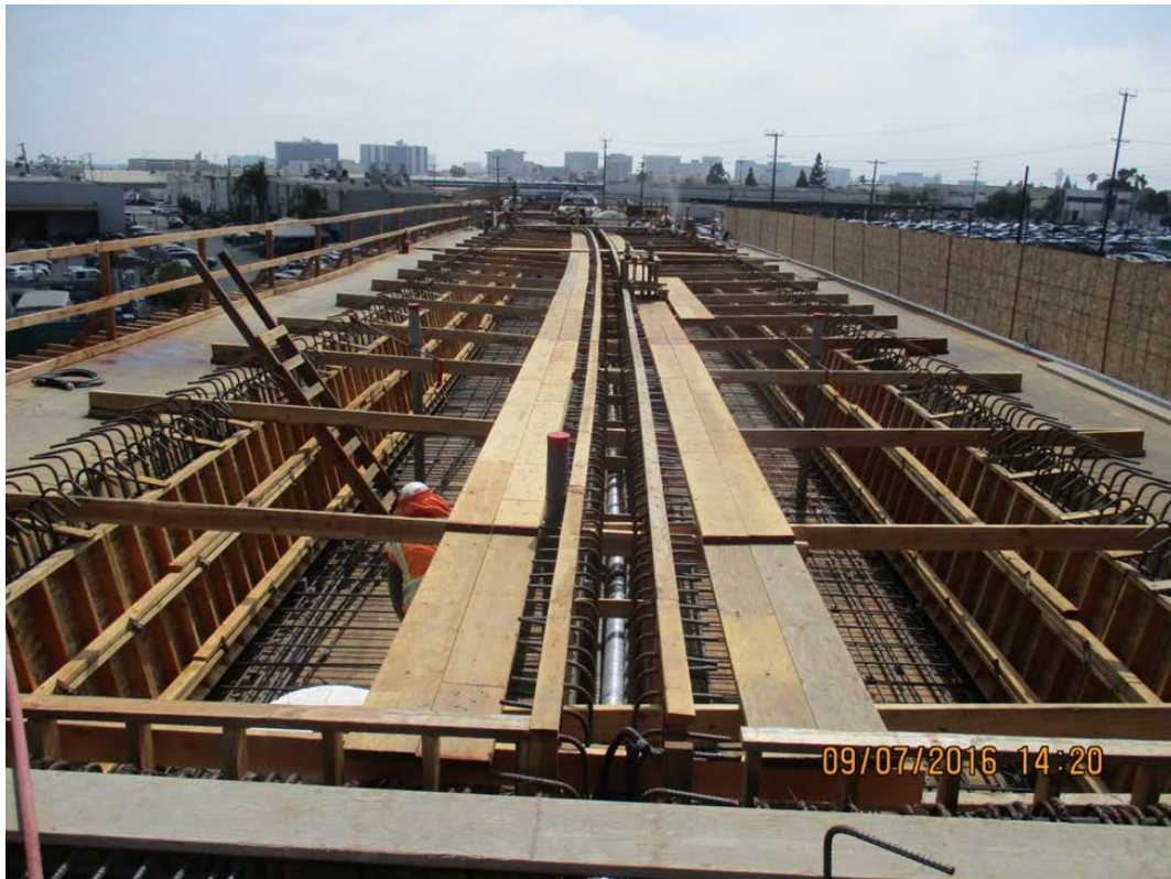
MANCHESTER BRIDGE – Finished formwork, placed and cured concrete for the stems and soffit.
