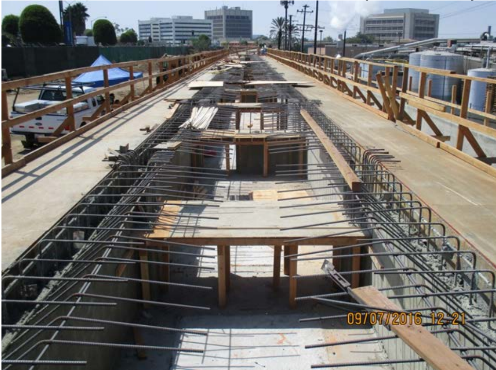
DOWNTOWN INGLEWOOD STATION – Deck formwork starts for the Downtown Inglewood Station platform.
