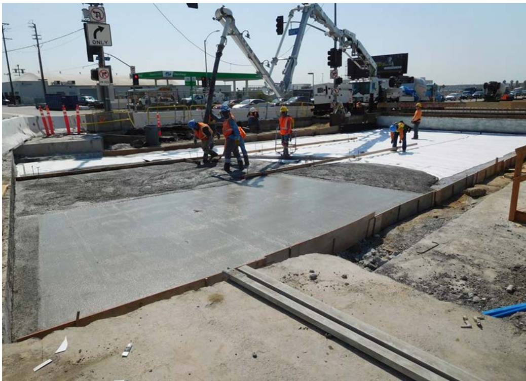
104 th STREET – Finished cut and cover tunnel including waterproofing protection slab and street restoration.
