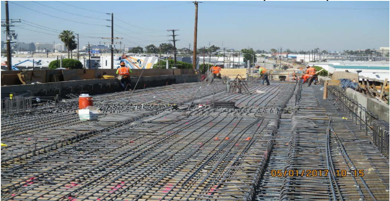
(AG-5) I-405 BRIDGE- Crews finished lost deck construction. Subcontractor IRP continued installing deck, overhang and parapet curb reinforcement. Deck pour tentatively scheduled for May 13th. (Span 1).
