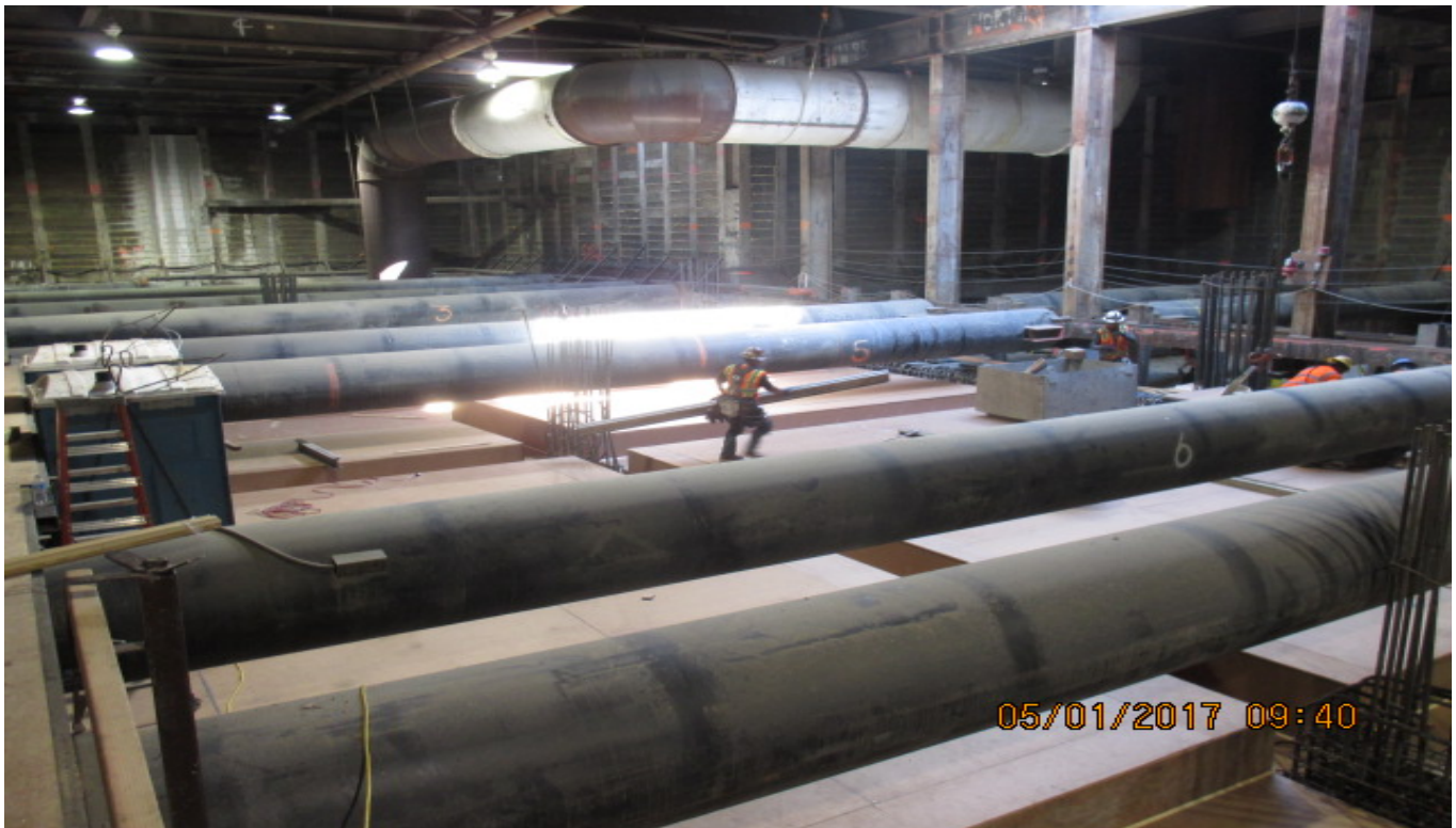
LEIMERT PARK STATION – Installation of formwork and rebar for concourse level slab.
