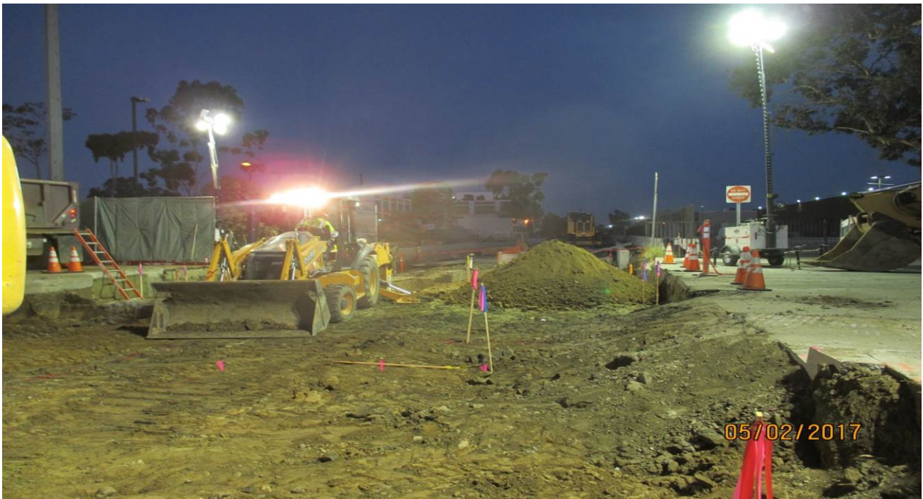
EUCALYPTUS GRADE CROSSING - AC paving of the approach and departure to match the existing elevation of Centinela Ave.
