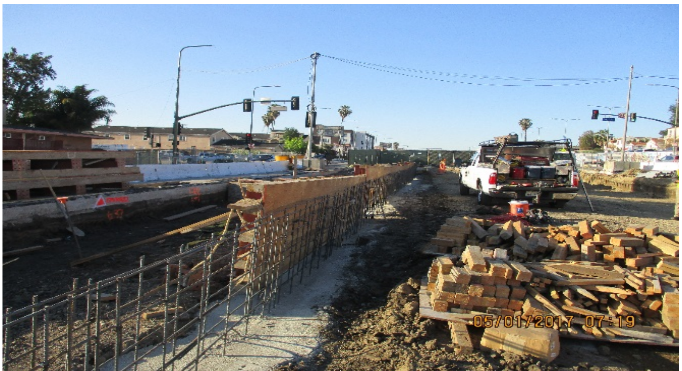
PARK MESA – Installation of formwork for ballast wall south of 50th St.
