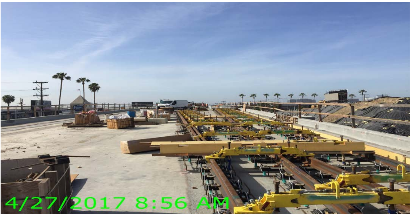
4/27/2017 8:56 AM AVIATION/CENTURY BRIDGE – Iron horse assembly in preparation for top-down construction of the 10K1 and 10K2 crossover.
