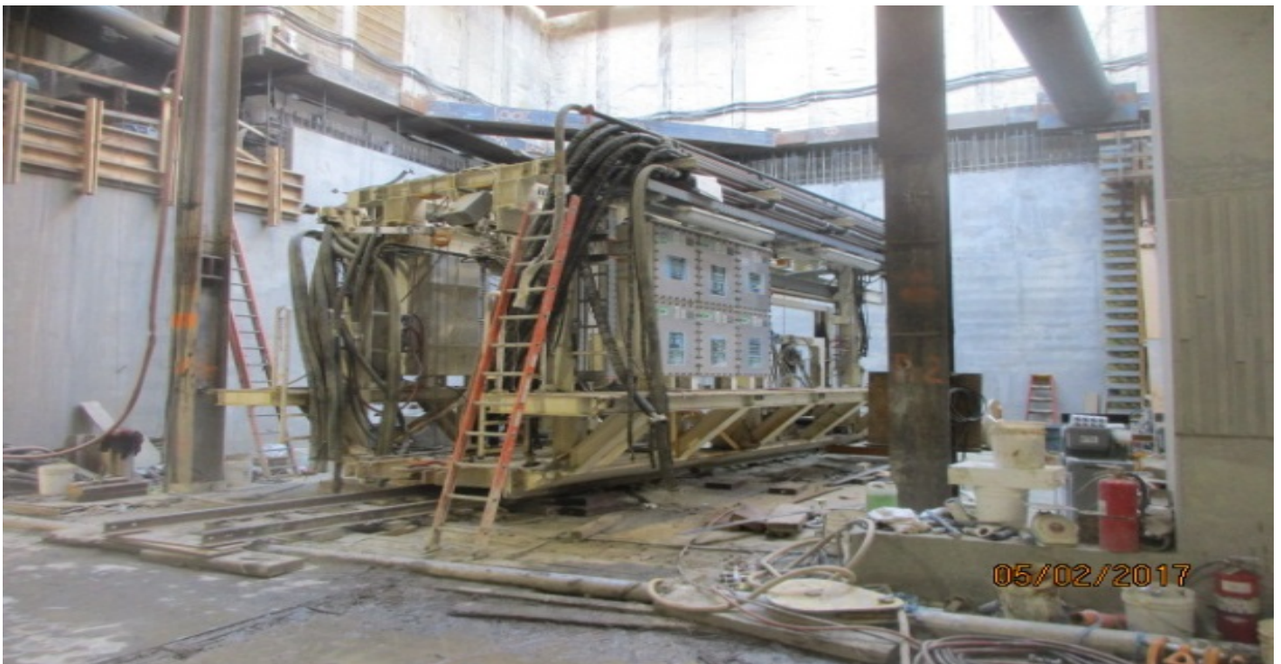
TUNNELING – Disassembling TBM trailing gear car #2 and preparing to hoist out of MLK Station.
