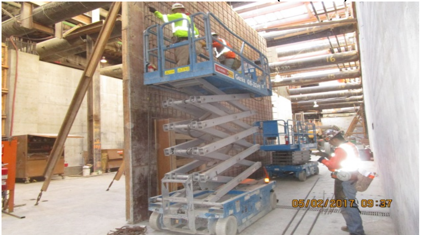
MARTIN LUTHER KING JR. STATION – Installation of formwork for interior wall section LW-28.
