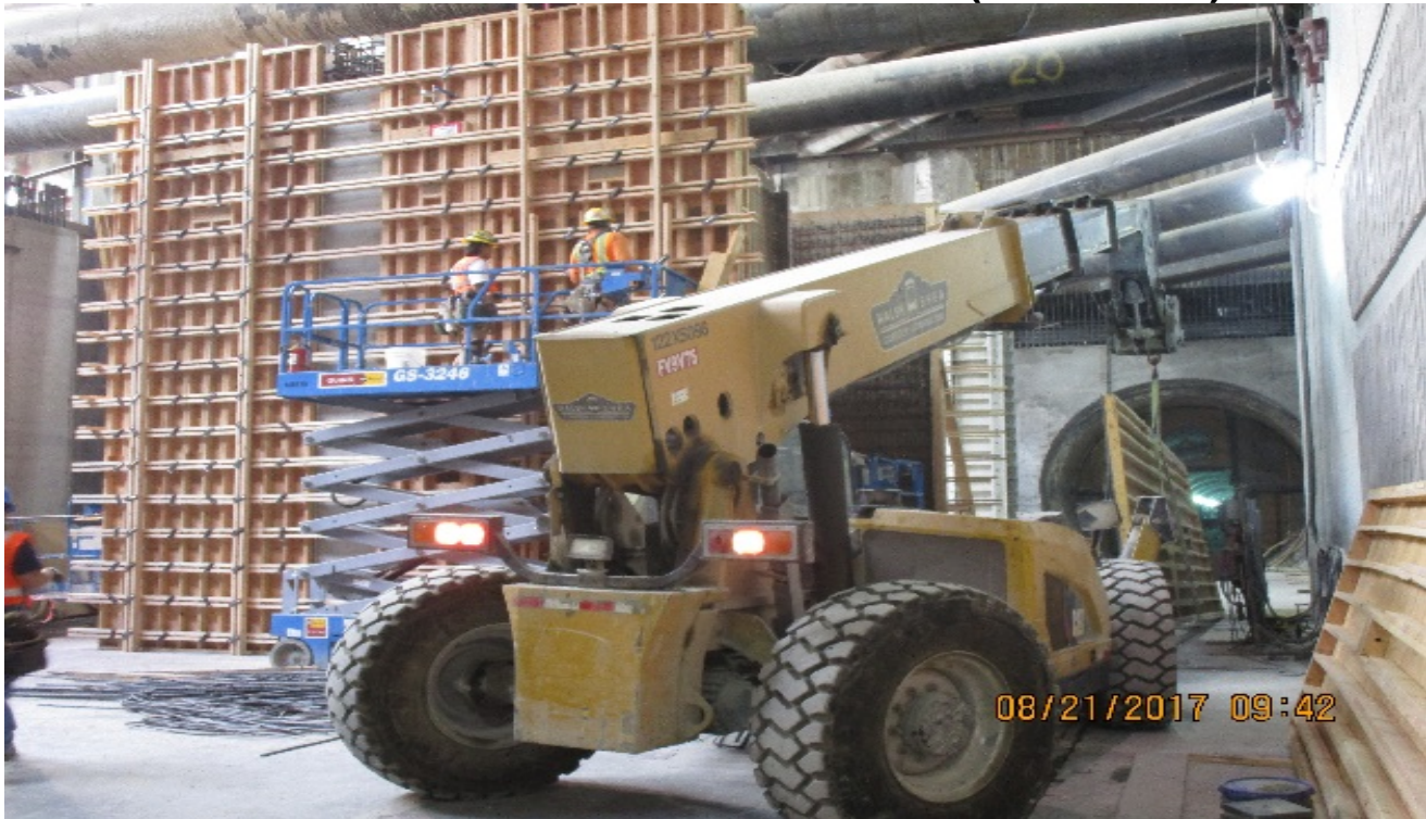
MARTIN LUTHER KING JR. STATION – Installation of formwork for north emergency stairs interior walls.
