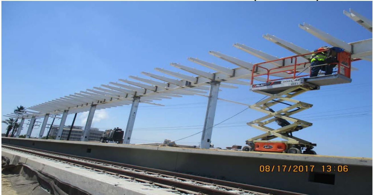
LA BREA AT GRADE STATION - Canopy frame erection complete. Crews worked on welding mounting brackets and electrical and plumbing installations.
