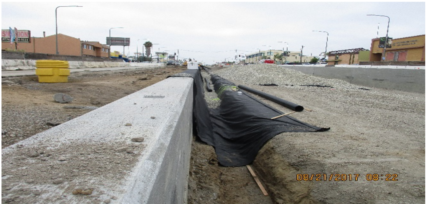
PARK MESA —Backfill activities along the northbound ballast walls between 50th and 52nd St.
