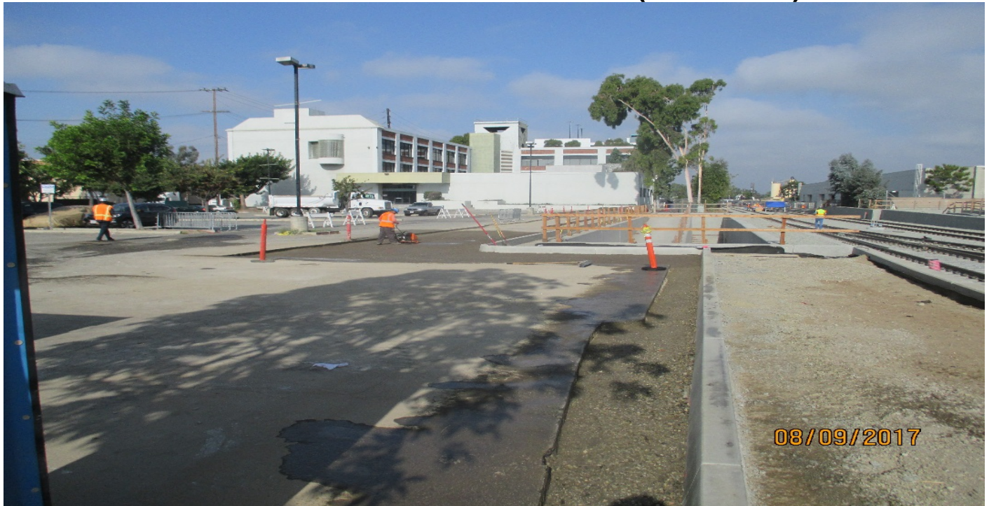
(AG-7) FCBC PED UP - Crews continued work on the FCBC parking lot extension/reconstruction.
