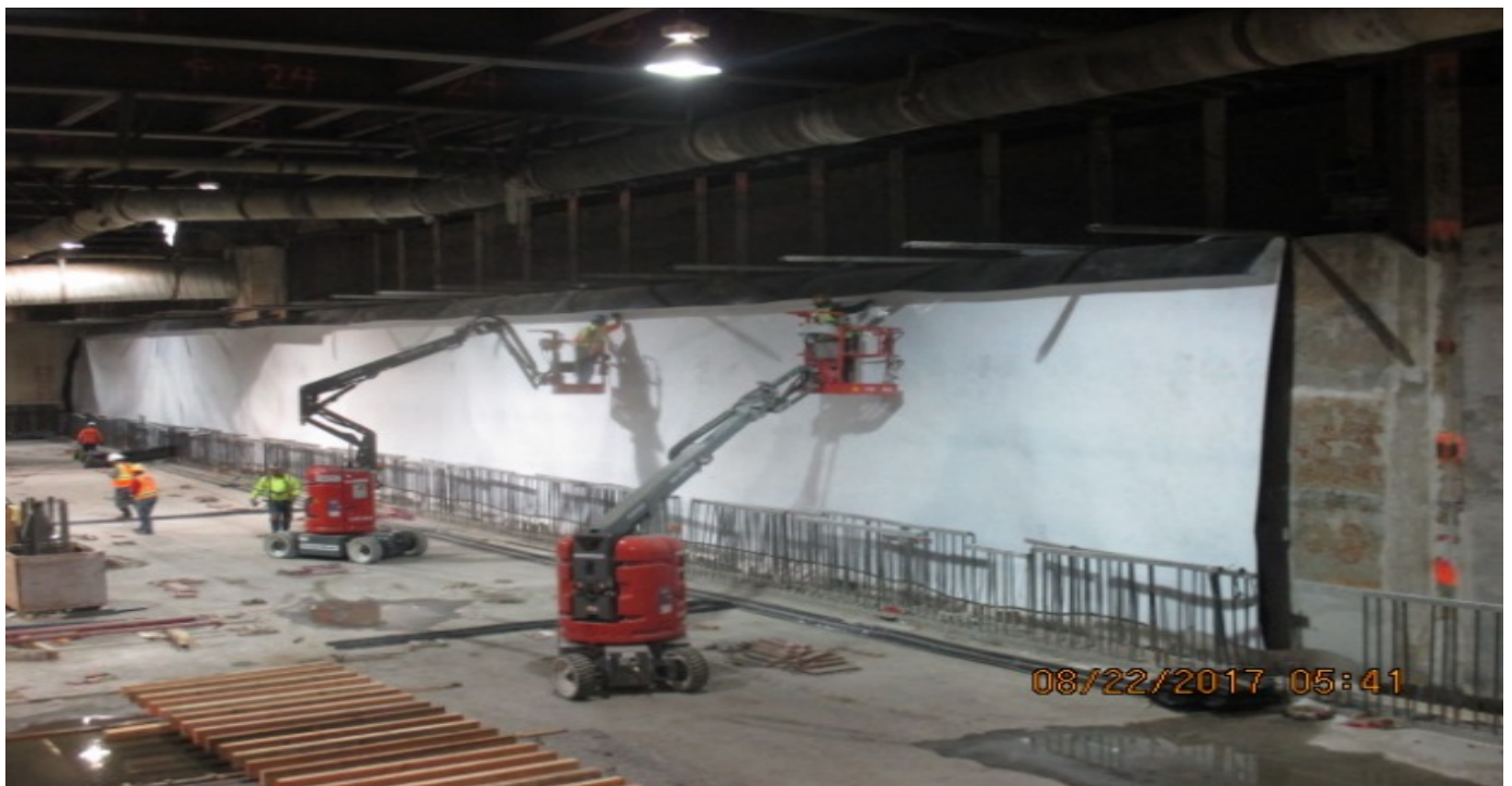
LEIMERT PARK STATION - Installing waterproofing along concourse level wall sections UW-1 thru UW-4.
