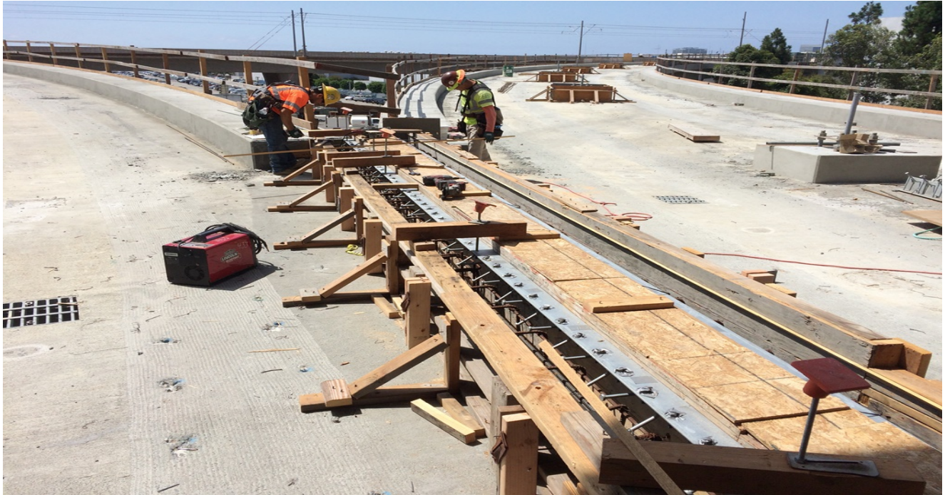
GREENLINE UNDERPASS Remaining portion of parapet curb underway at the wye junction.
