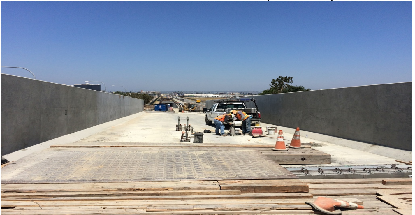
111 th Street – Bridge superstructure complete, DF track plinths to follow. Crews worked on girder wall finish work.
