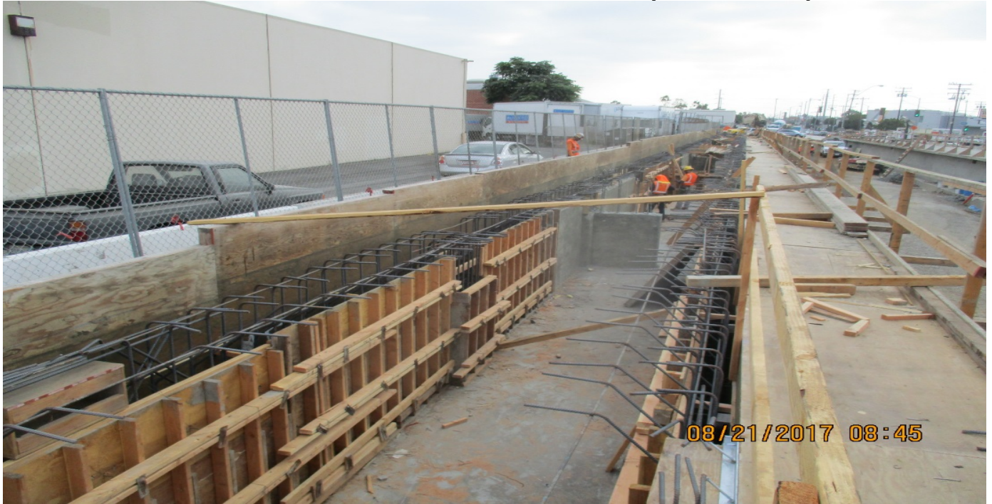
WESTCHESTER STATION – Exterior finish work continued along the NB platform stem walls.
