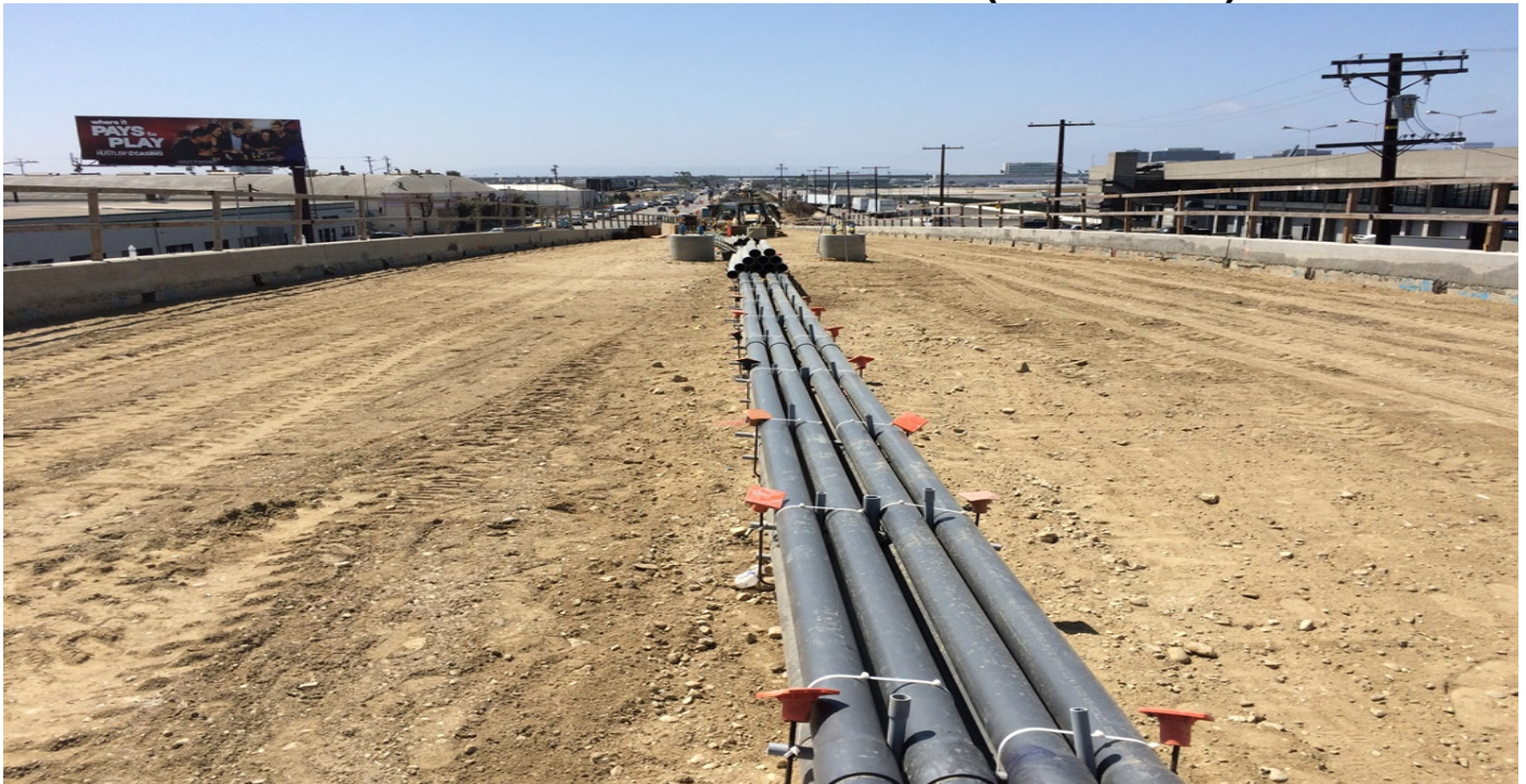
MSE 60L&R –Crews finished fine-grading in preparation for AC cap placement and Neil Electric laid conduit for the combined emergency walkway/ductbank.
