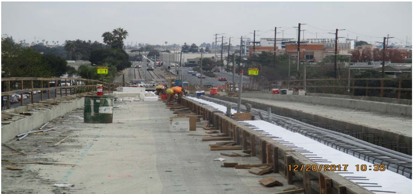
(AG-5) I-405 - Span 4 epoxied reinforcement doweling and bracing the north face of ductbank.
