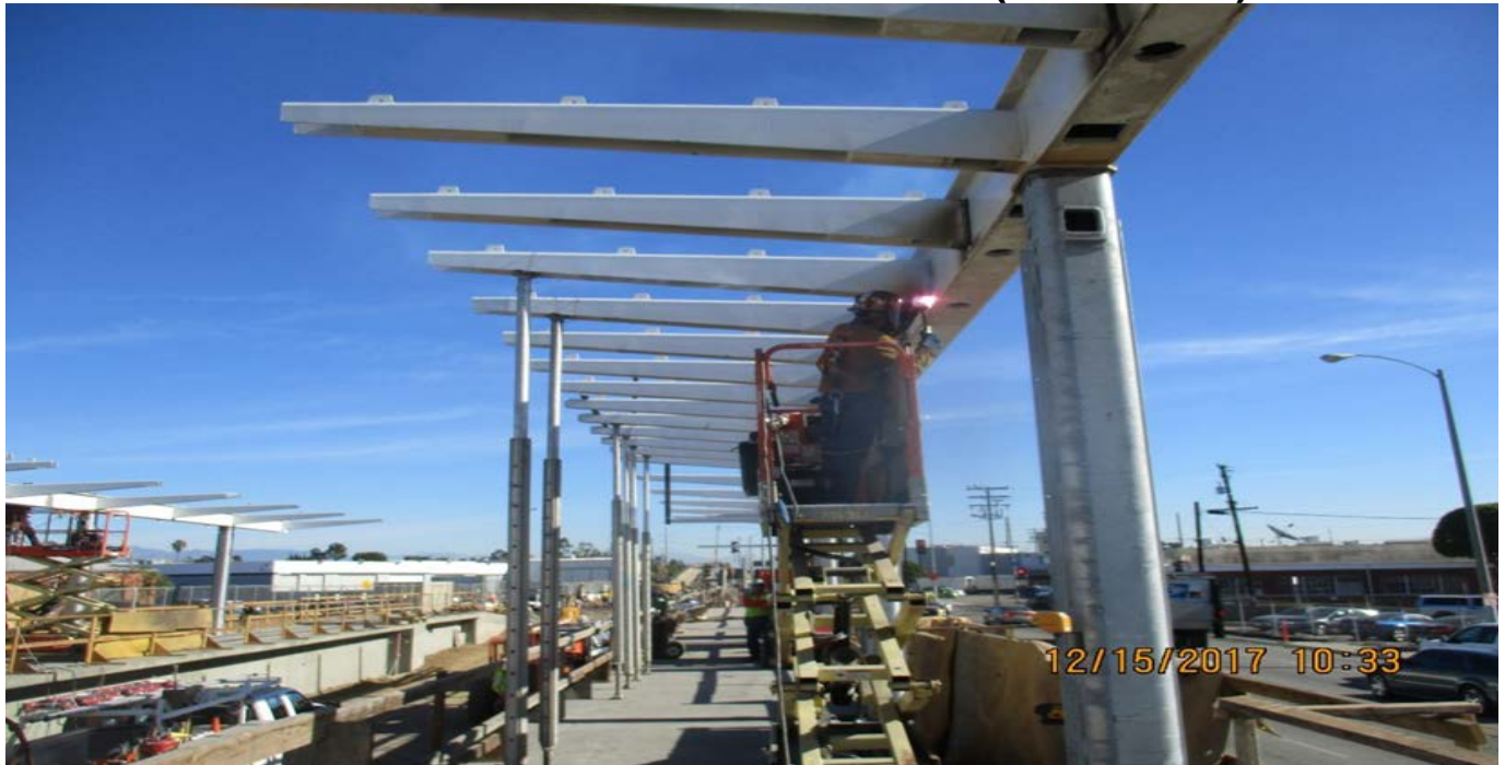
WESTCHESTER STATION – Crew continued splice welding of canopy frames and column to canopy girder FP.
