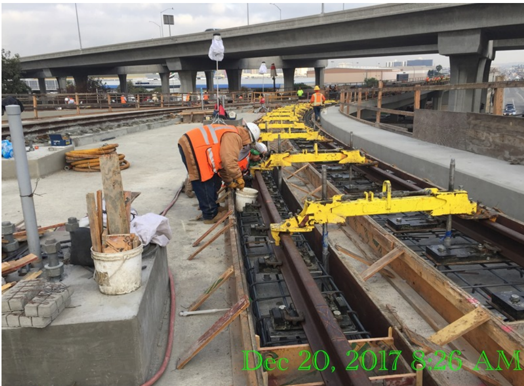
GREENLINE UNDERPASS – Crew continued installation of iron horse system and rail fasteners on track-4 NB.
