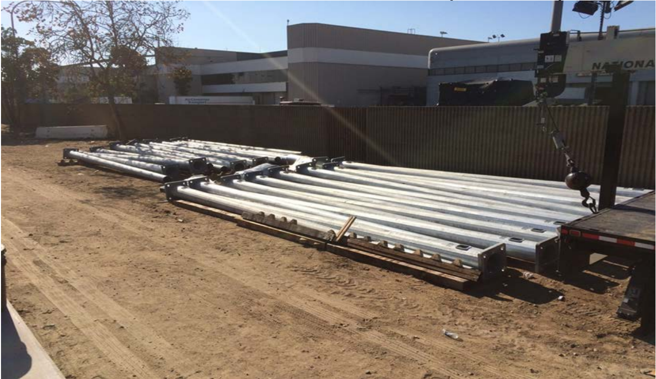
MSE 29L&R – OCS poles delivered and stock piled on the west side of the retaining wall.
