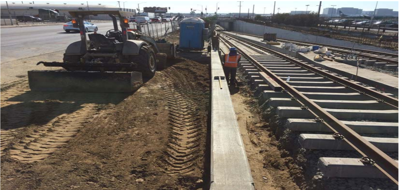
UG1 – Backfill and compaction on both sides of the retainer wall STA 59+50 to 60+00.
