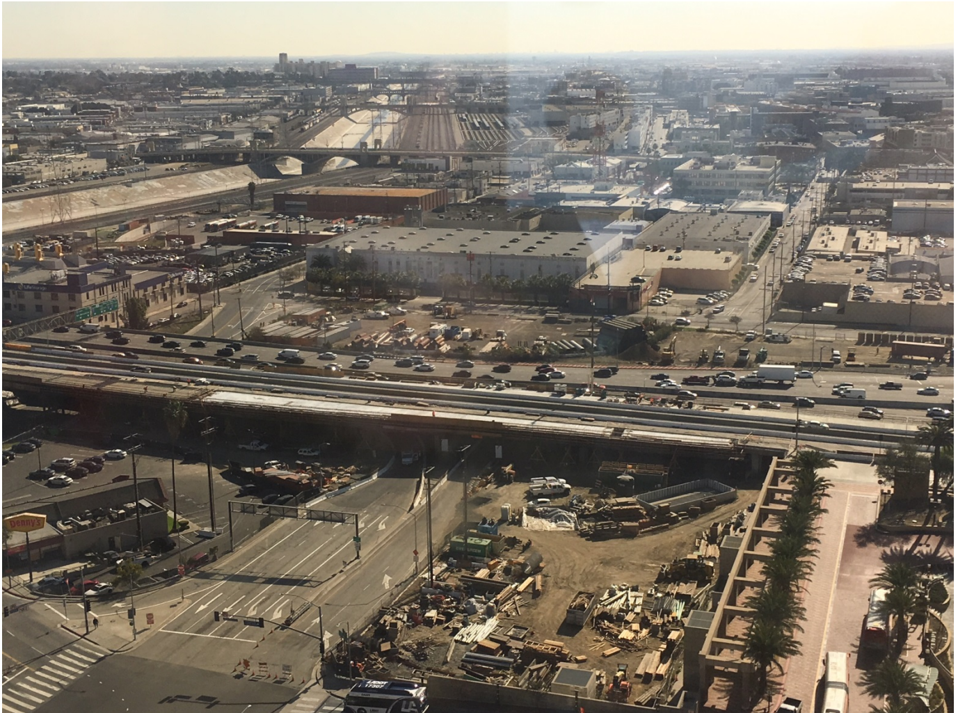
Photo taken from the south side of the Metro Gateway Building provides an aerial view of the jobsite.
