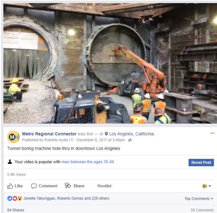
Live stream video of tunnel boring machine breakthrough at Grand Av Arts/Bunker Hill 18.3k people reached; 6.0k video views; 7.3k minutes viewed
