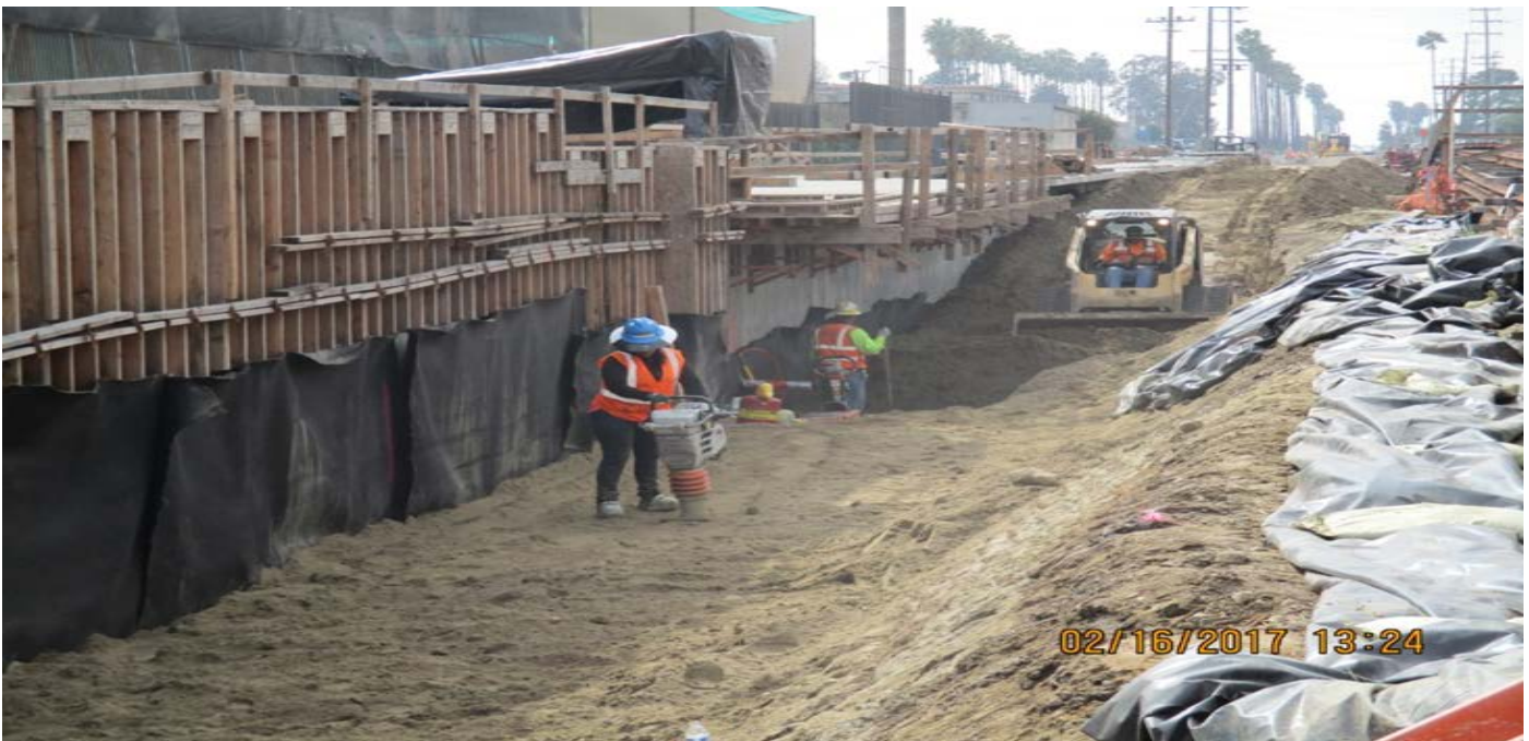
FAIRVIEW HEIGHTS STATION - Crews began backfilling and compaction testing along the outside perimeter of the TC&C room retaining walls.
