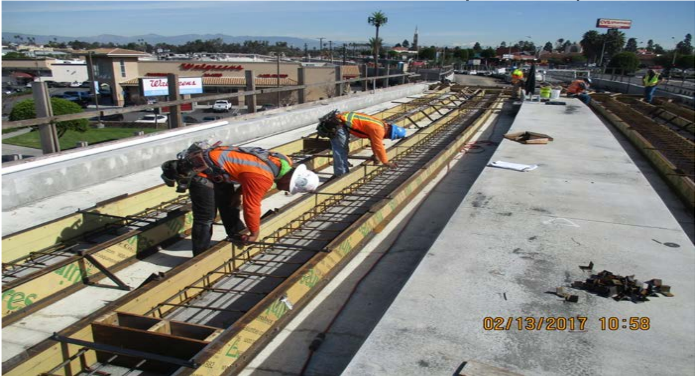
(AG-6) LA BREA BRIDGE – Reinforcement and formwork installations complete for the second pour plinth pads.
