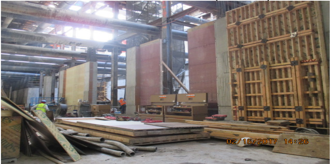
MARTIN LUTHER KING JR. STATION – Installation of formwork for lower interior walls.
