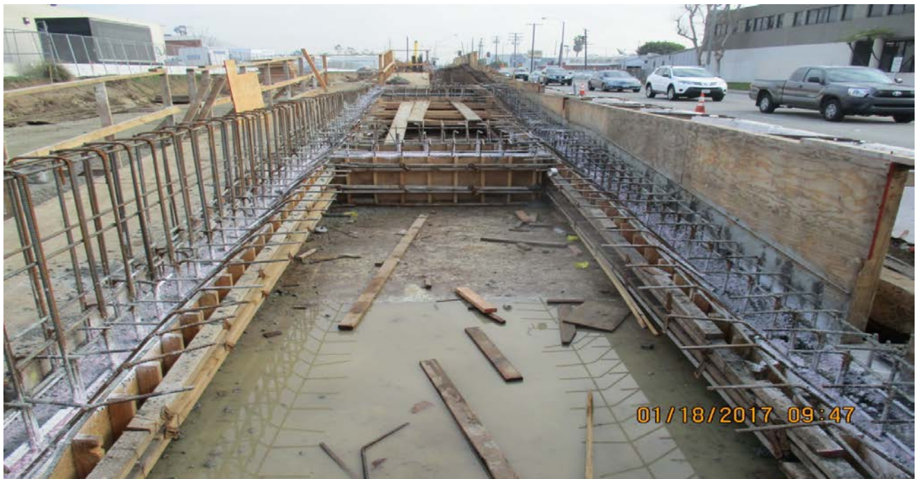
WESTCHESTER STATION – Concrete placement for the northbound platform's stem walls, shear walls and engaged columns.
