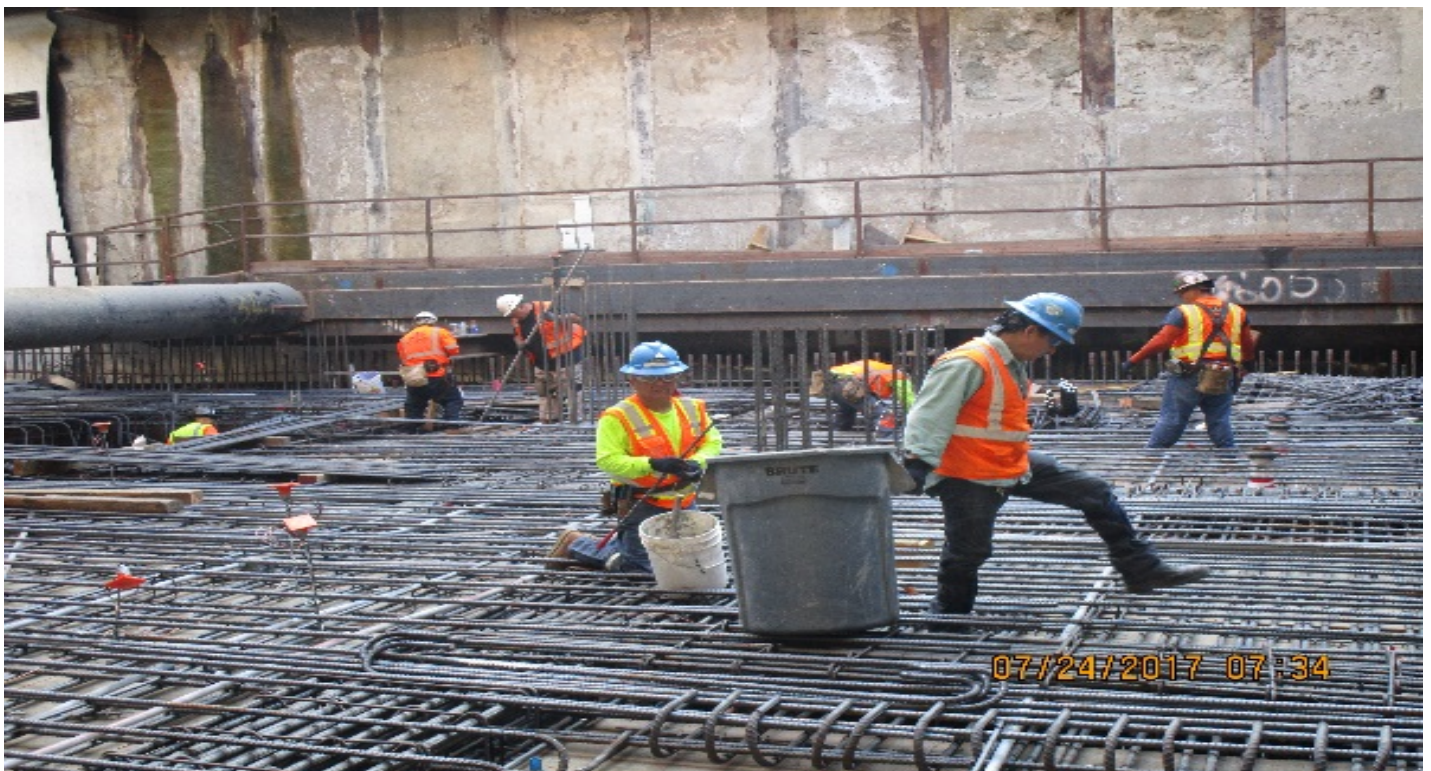
EXPOSITION/CRENSHAW STATION – Installation of formwork, rebar, and electrical components for Concourse Slab Phase 3.
