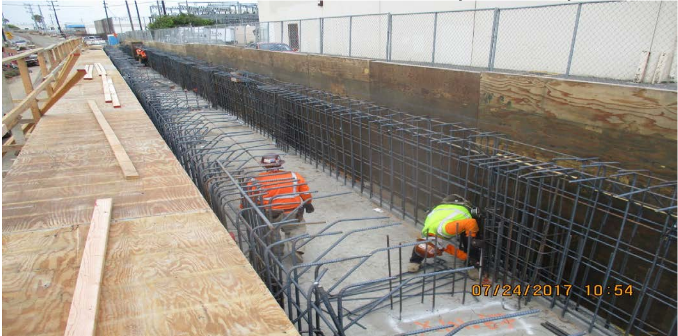
WESTCHESTER STATION – Crews continued exterior concrete finish work along the north bound station platform stem walls. Crews continued installing reinforcement and formwork for the south bound platform stem walls and center overhang.
