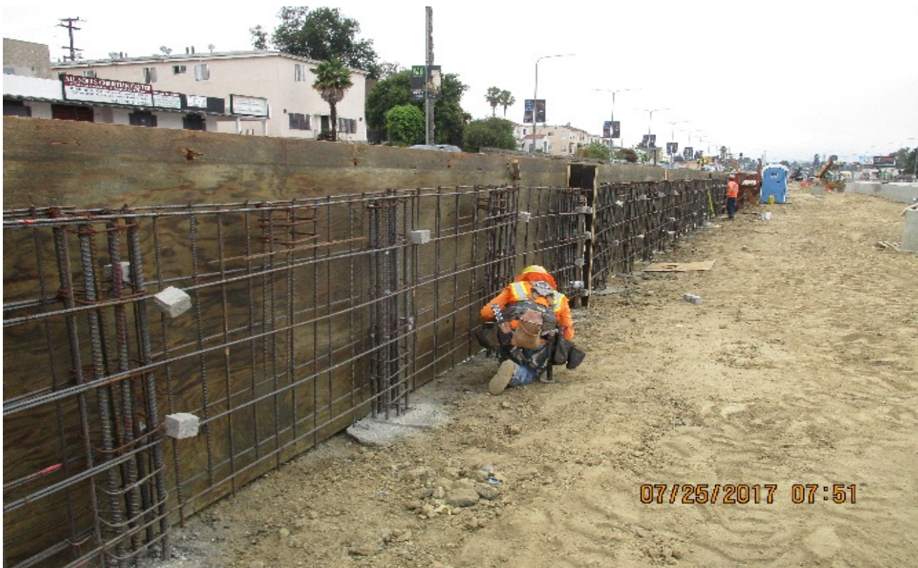
PARK MESA – Installation of formwork for ballast wall between 50th St. and 52nd St.
