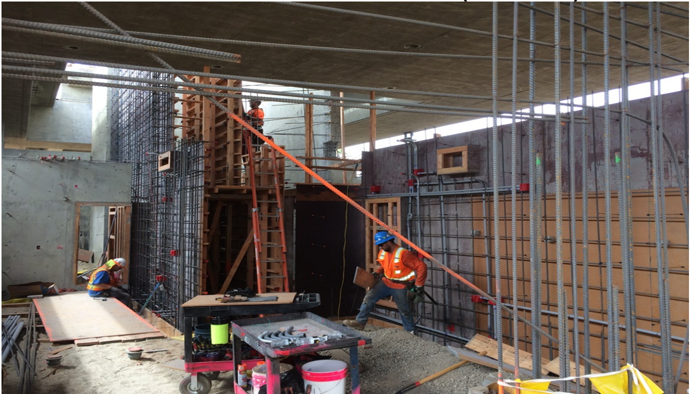
AVIATION/CENTURY BRIDGE – Construction of the plaza level service building walls, station elevator shaft and emergency stairway wall underway.
