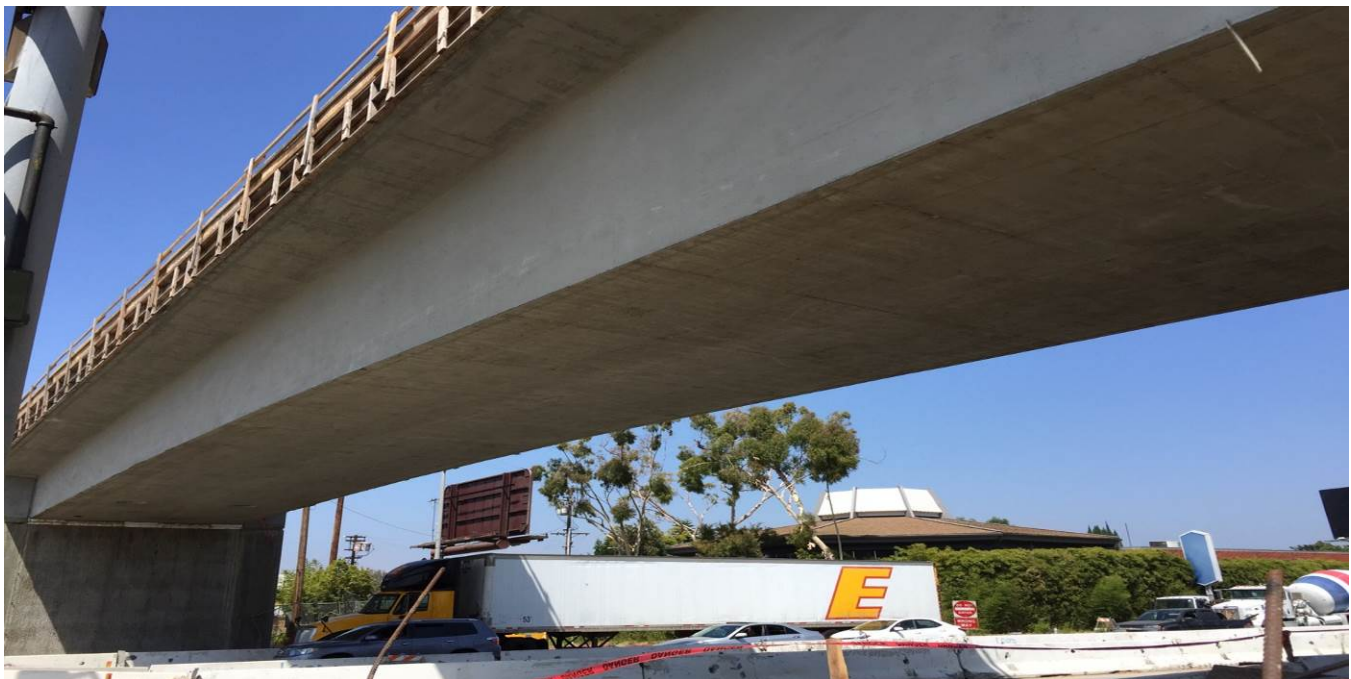
(AG-5) I-405 BRIDGE- Crews finished removing falsework from spans 1, 3 and 4. Crews continued stripping formwork and finish work along the exterior girder stems. Falsework removal from span 2 (over the I-405) will be completed under nightly freeway lane closures from 7/31 through 8/18.
