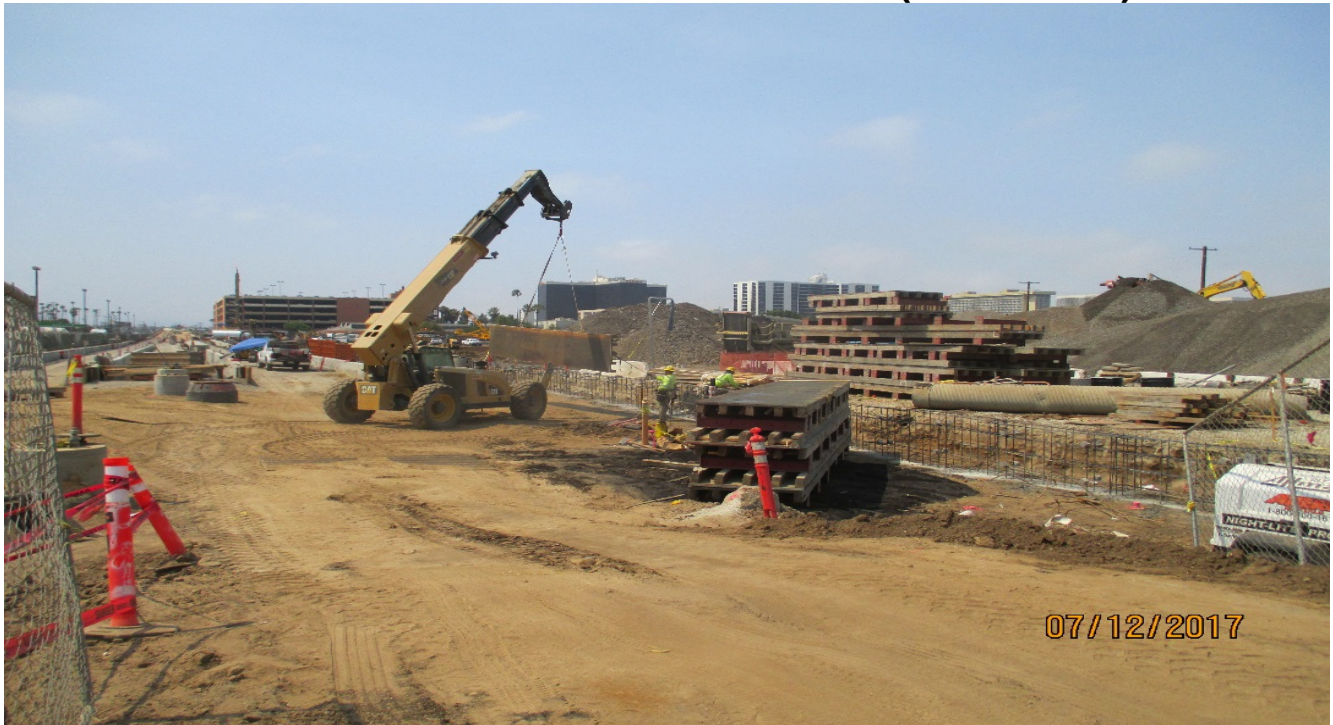
A1 GUIDEWAY- SB ballast wall construction underway for the north yard lead directly south of Arbor Vitae.
