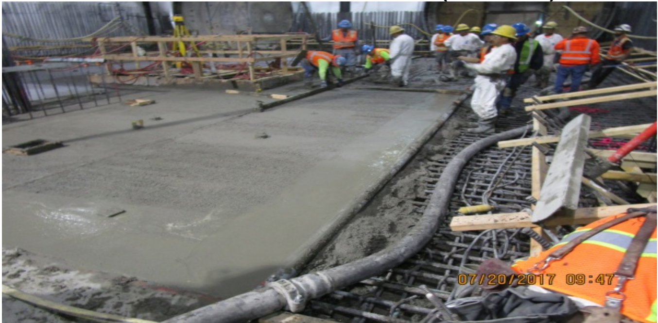
MARTIN LUTHER KING JR. STATION - Completed placement of final invert section S-1.
