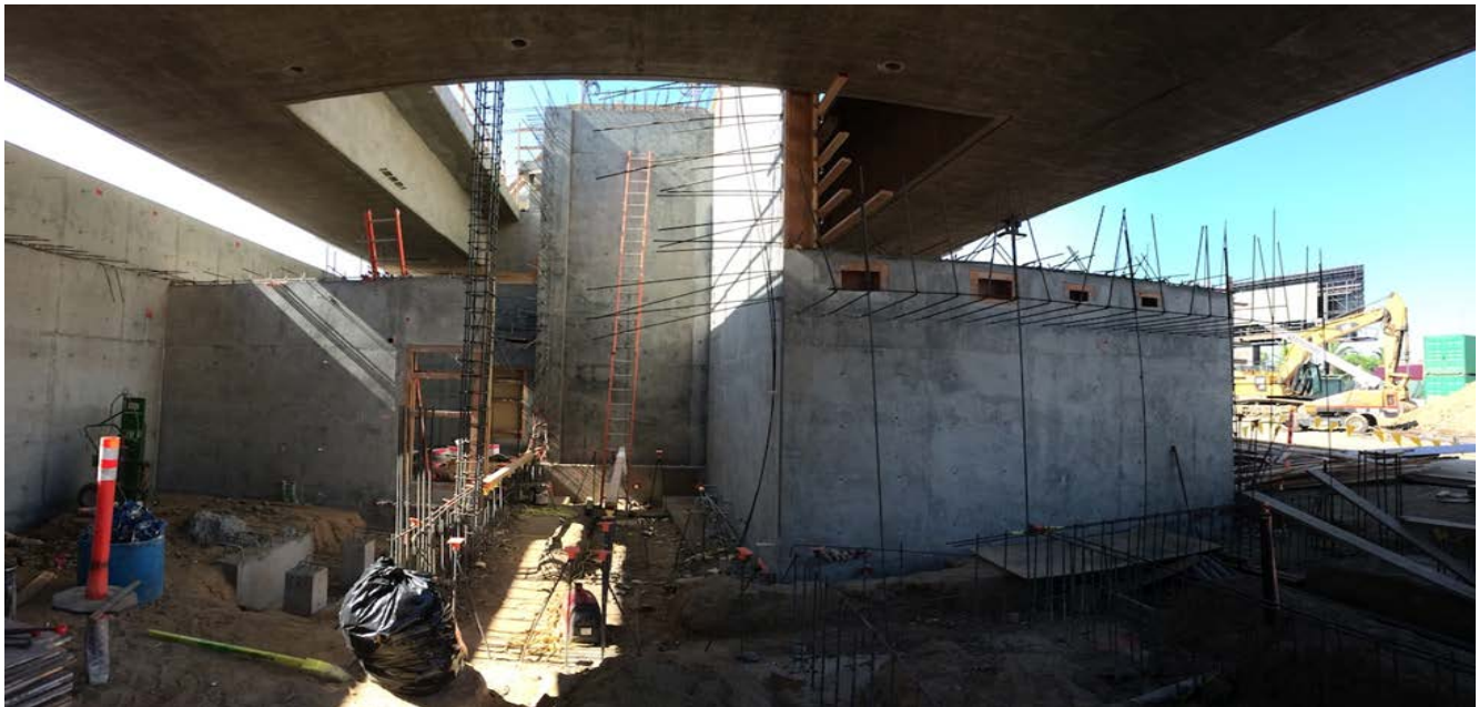
AVIATION/CENTURY BRIDGE – Construction of the plaza level service building and station elevator shaft underway.
