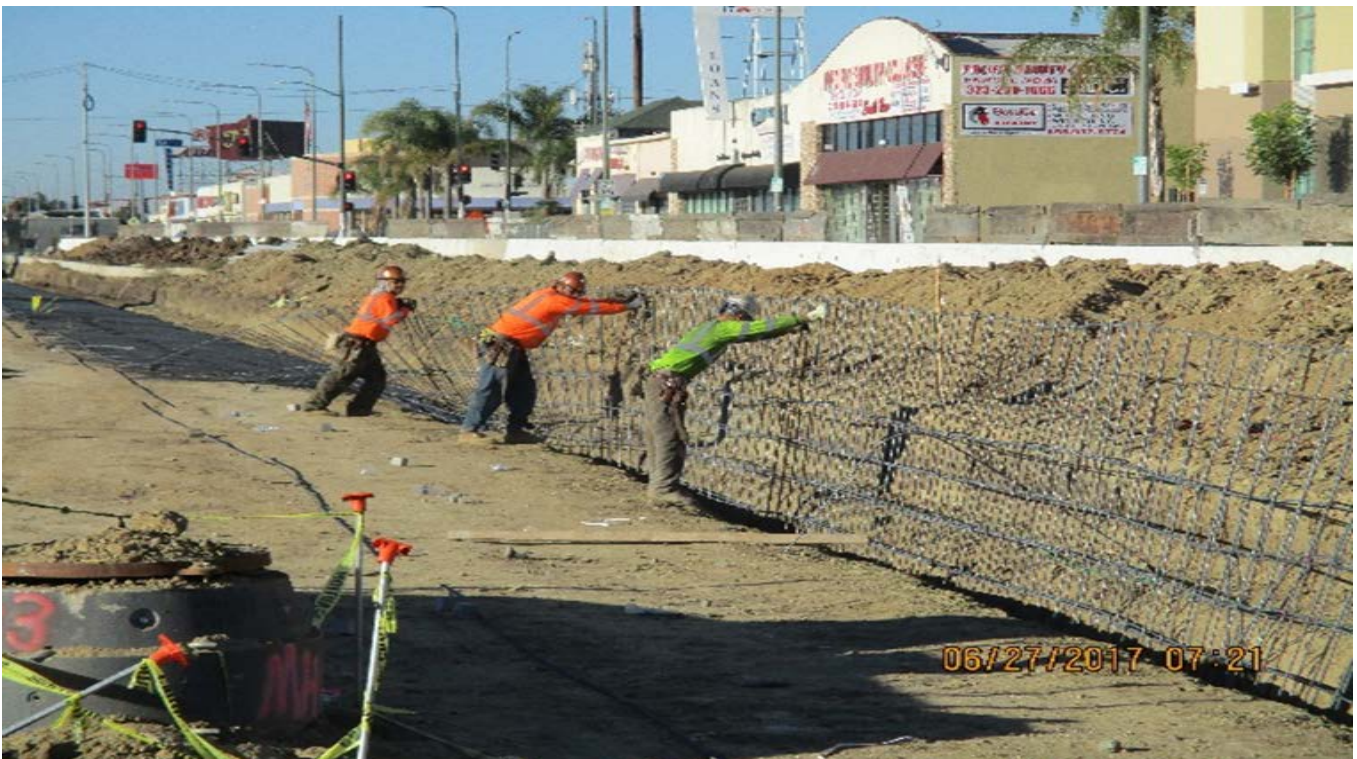
PARK MESA – Installation of ballast wall along west wall between 52nd St. and 54th St.
