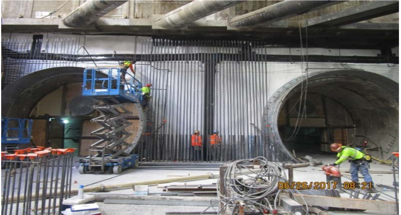
MARTIN LUTHER KING JR. STATION – Installation of rebar along south lower walls and installation of NB/SB Omega rings at south hammerhead.
