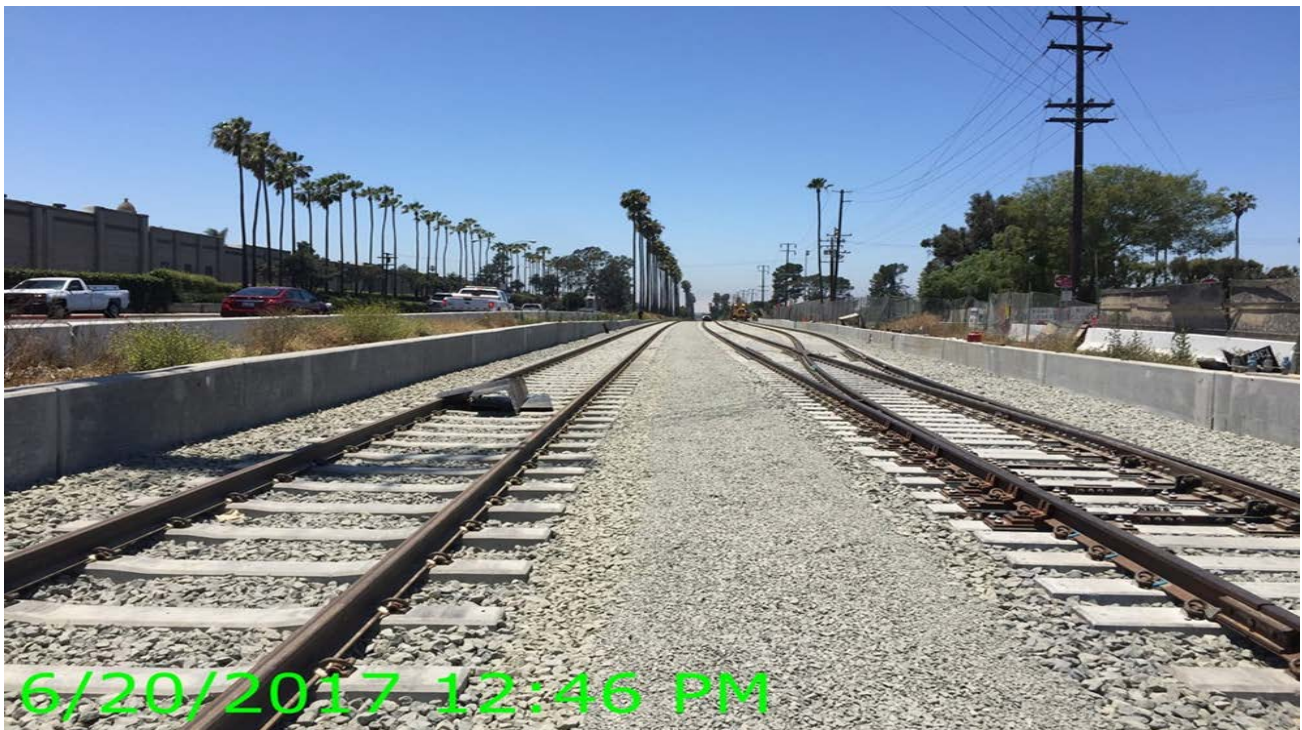
B1 GUIDEWAY – Ballasted trackwork between Centinela and High St. nearly complete with the exception of de-stressing. Siding track turnout to the right. Center walkway ballast has been placed.
