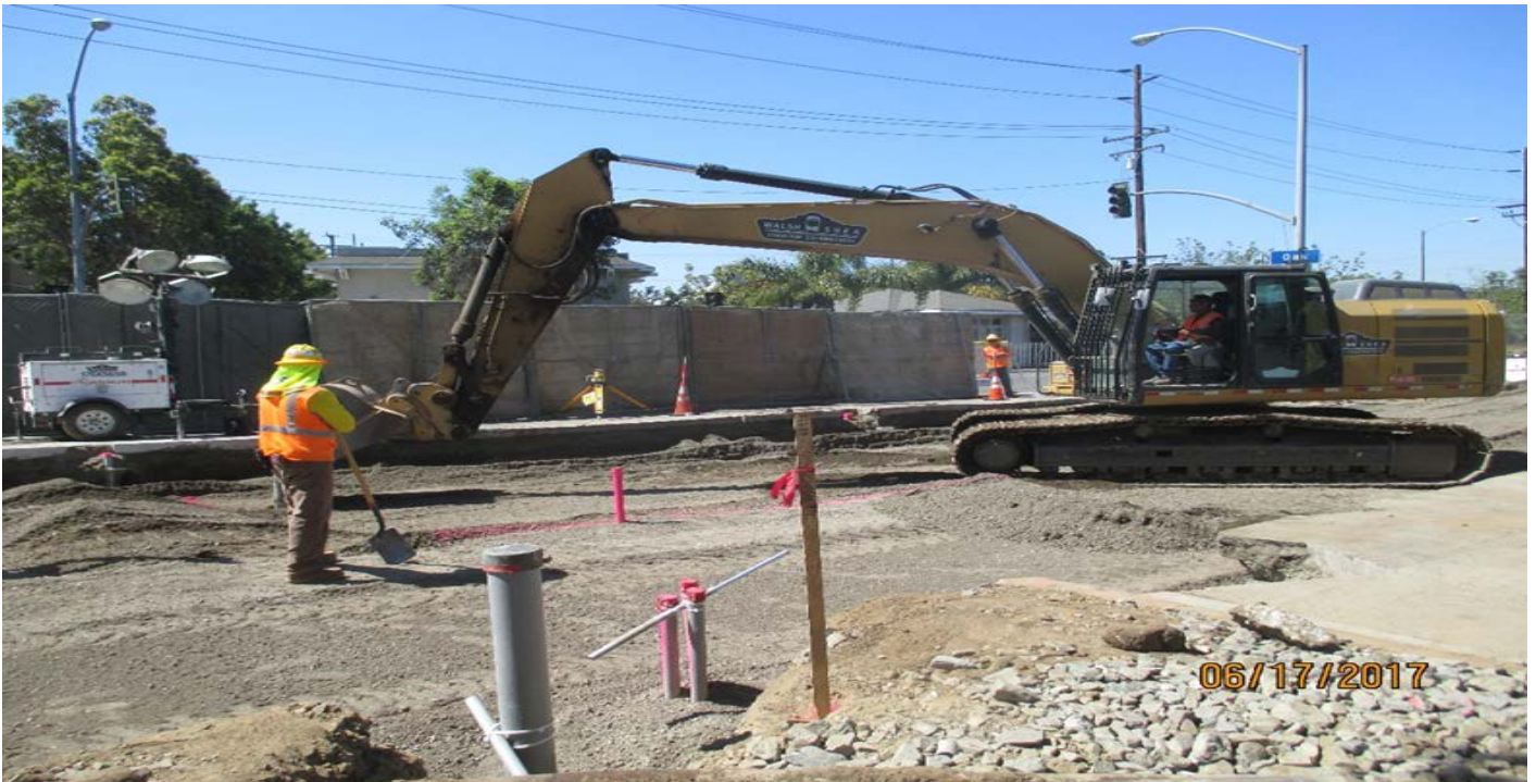
OAK ST. GRADE CROSSING - Crews finished the Oak Street grade crossing under a weekend closure.
