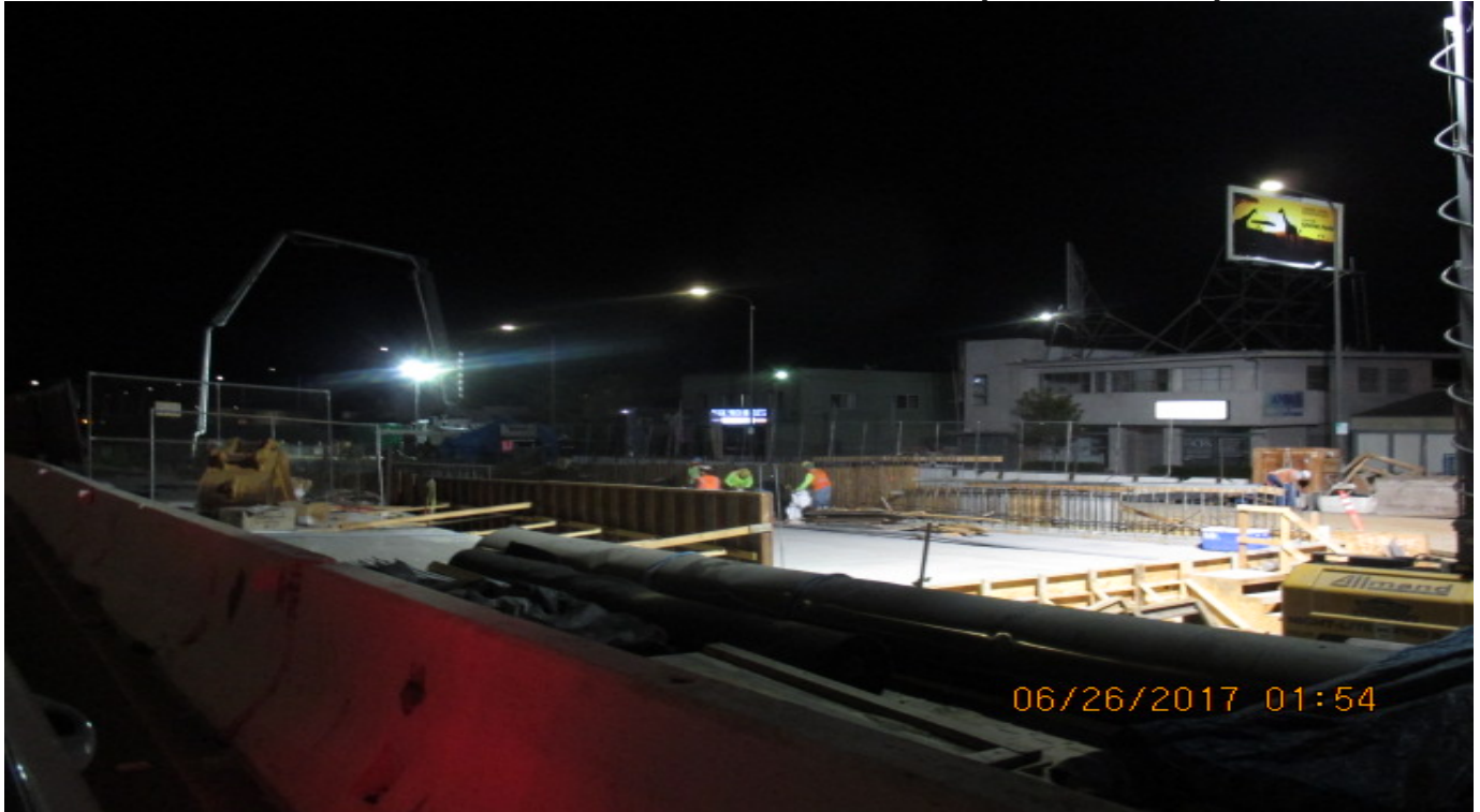
UG4 – Placement of invert sections I-2 and I-4; UG4 invert is now complete.
