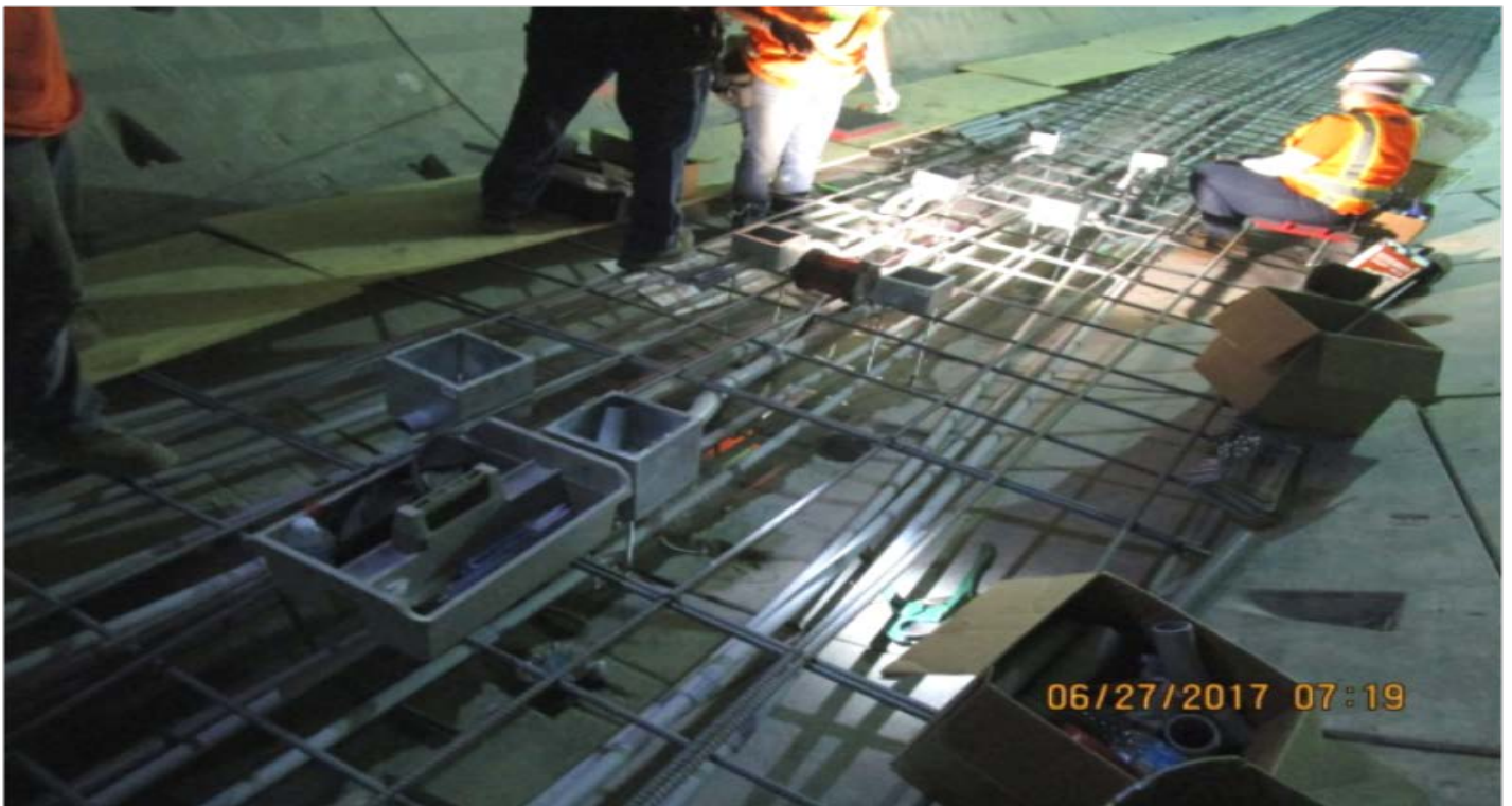
TUNNELING – Installation of electrical components/conduits for the NB tunnel invert between Expo and MLK.
