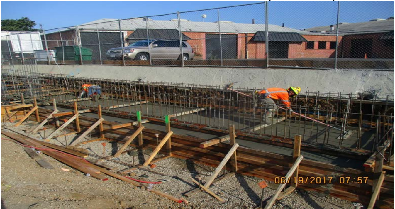
WESTCHESTER STATION – Crews continued with finish work for the north bound station platform. Crews placed concrete for the south bound platform footing.
