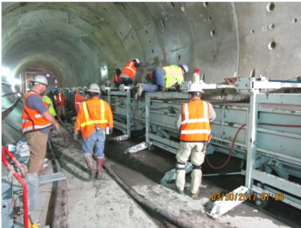
First Walkway placement in tunnel just south of MLK station – SB tunnel.
