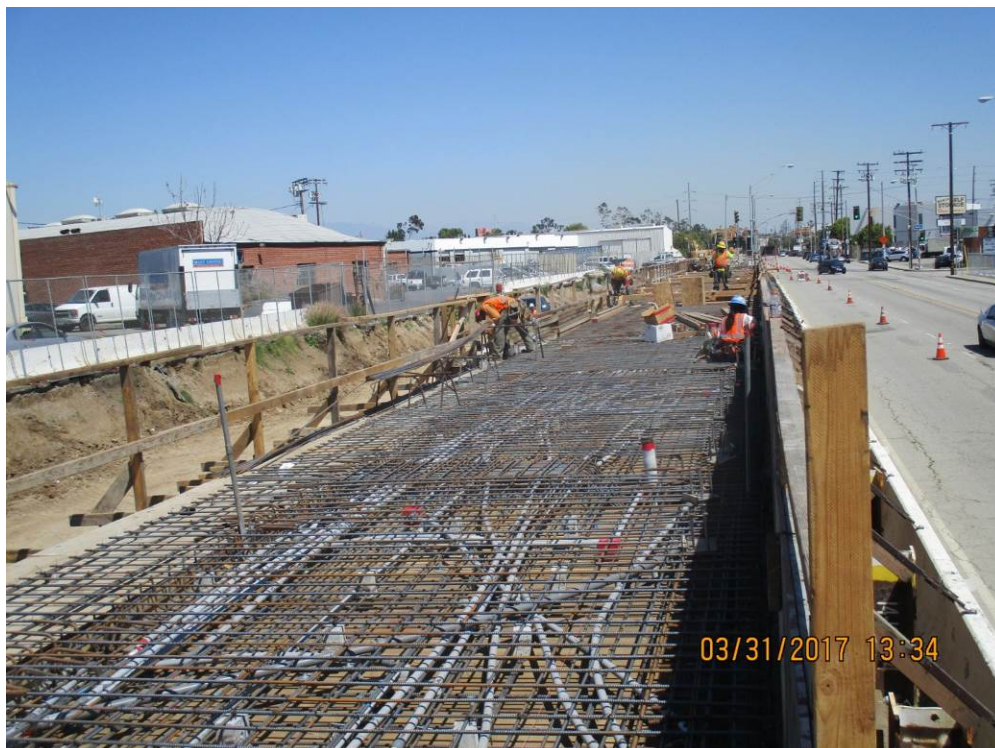
Deck reinforcement and conduit embed installations ongoing for Hindry Station NB platform (photo facing up-station).
