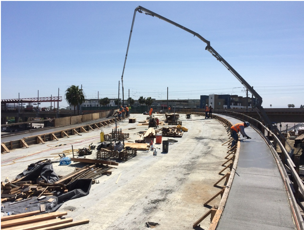
Contractor continues concrete placement for the multi-purpose emergency walkway/ductbank/parapet curbs for Green Line tie-in structure.
