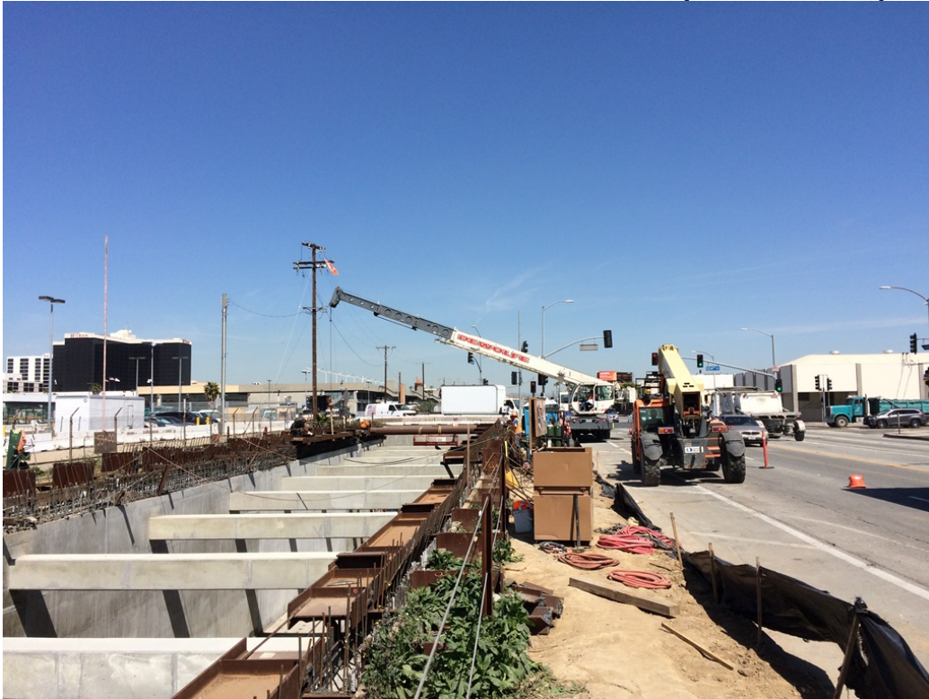
Tier 1 SOE strut removals nearly complete for tunnel in front of LAX runways.
