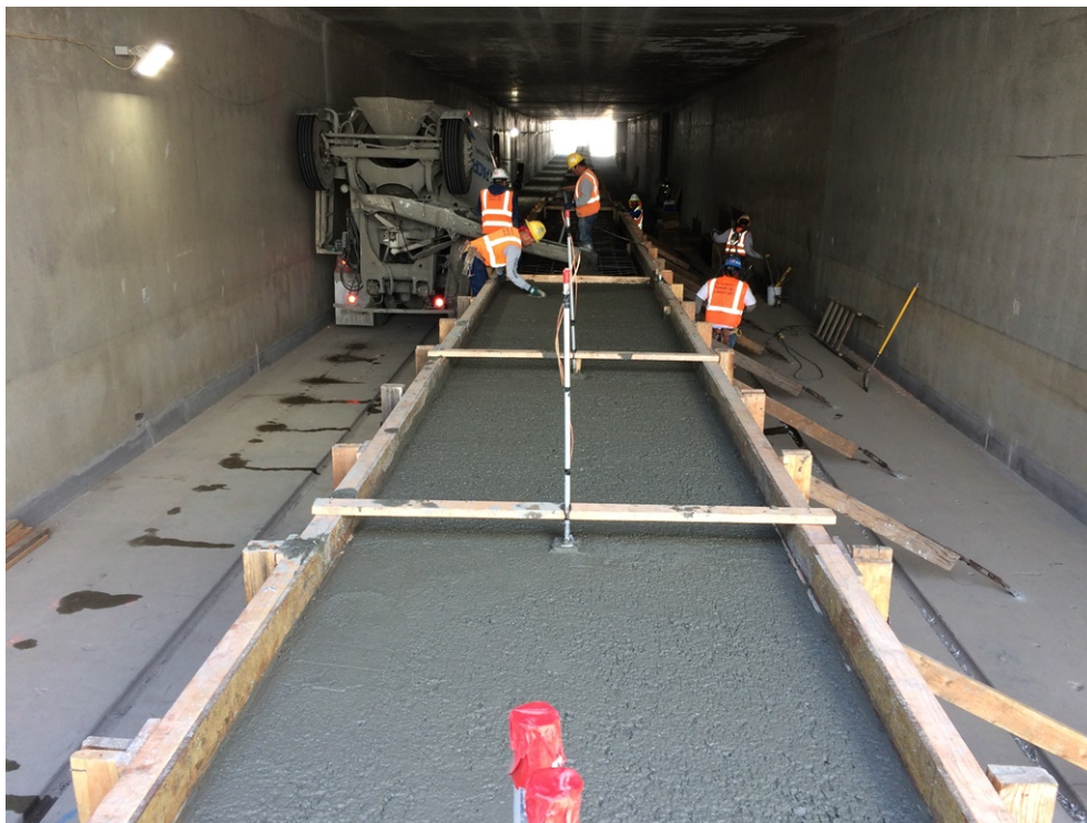
Contractor continues raised emergency walkway construction for tunnel in front of LAX runway.
