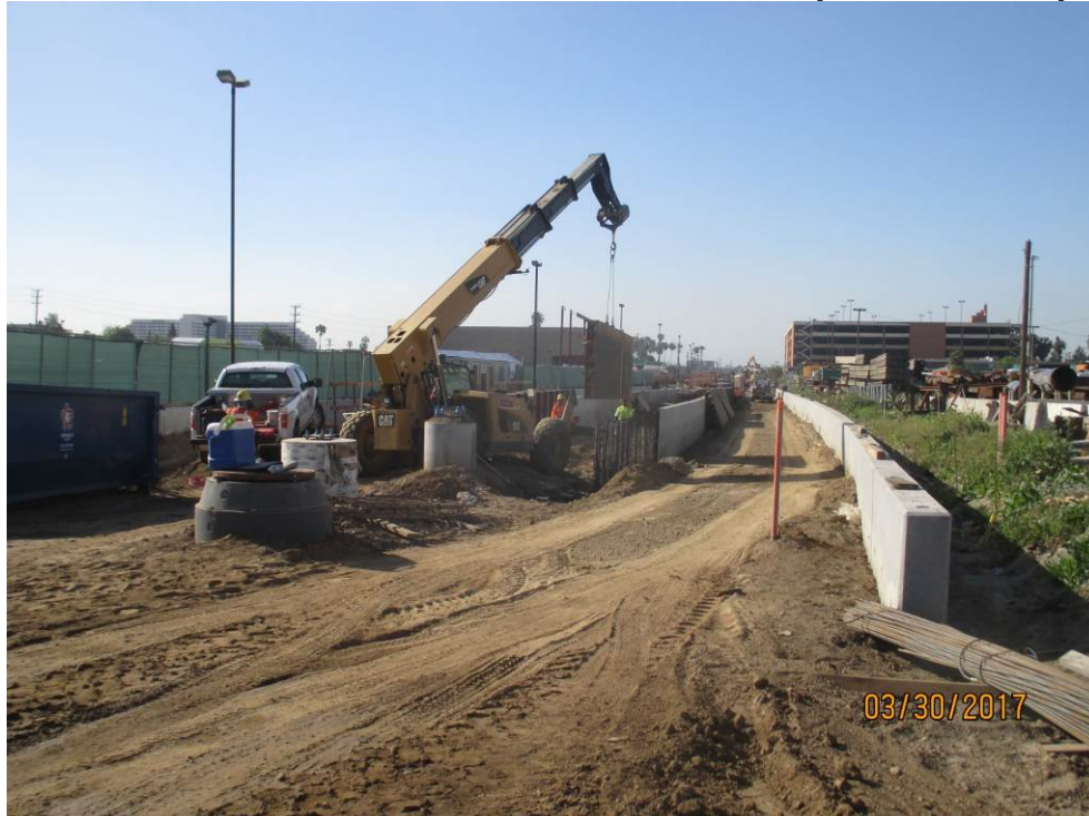
Contractor constructing the final remaining ballast walls for 96 th Street station accommodations effort.
