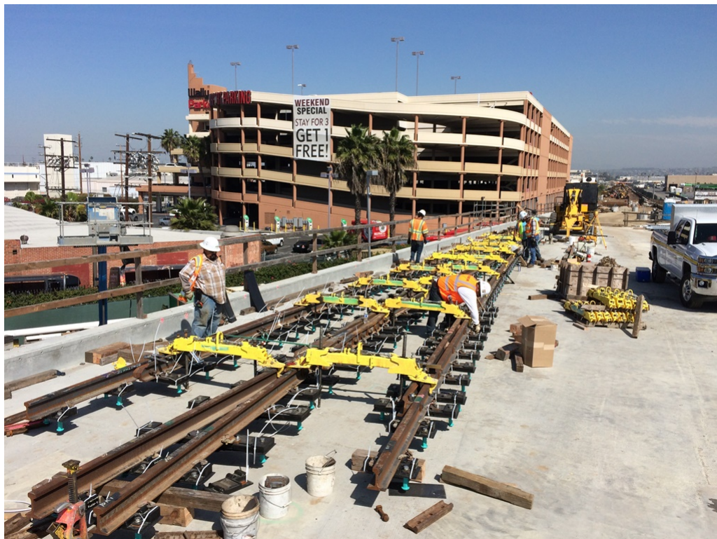
Iron horse assembly in preparation for top-down DF construction of the 10k and 10k1 crossovers.
