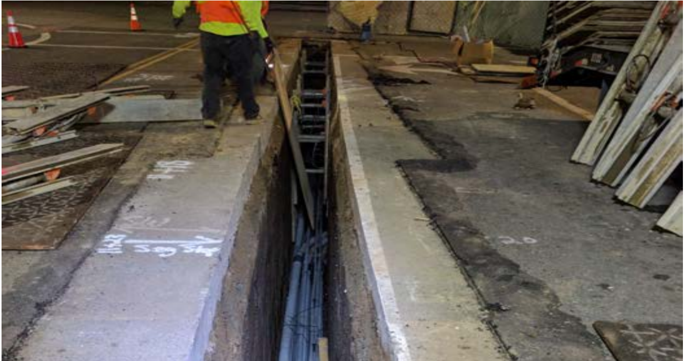
Century City Constellation Joint Trench
