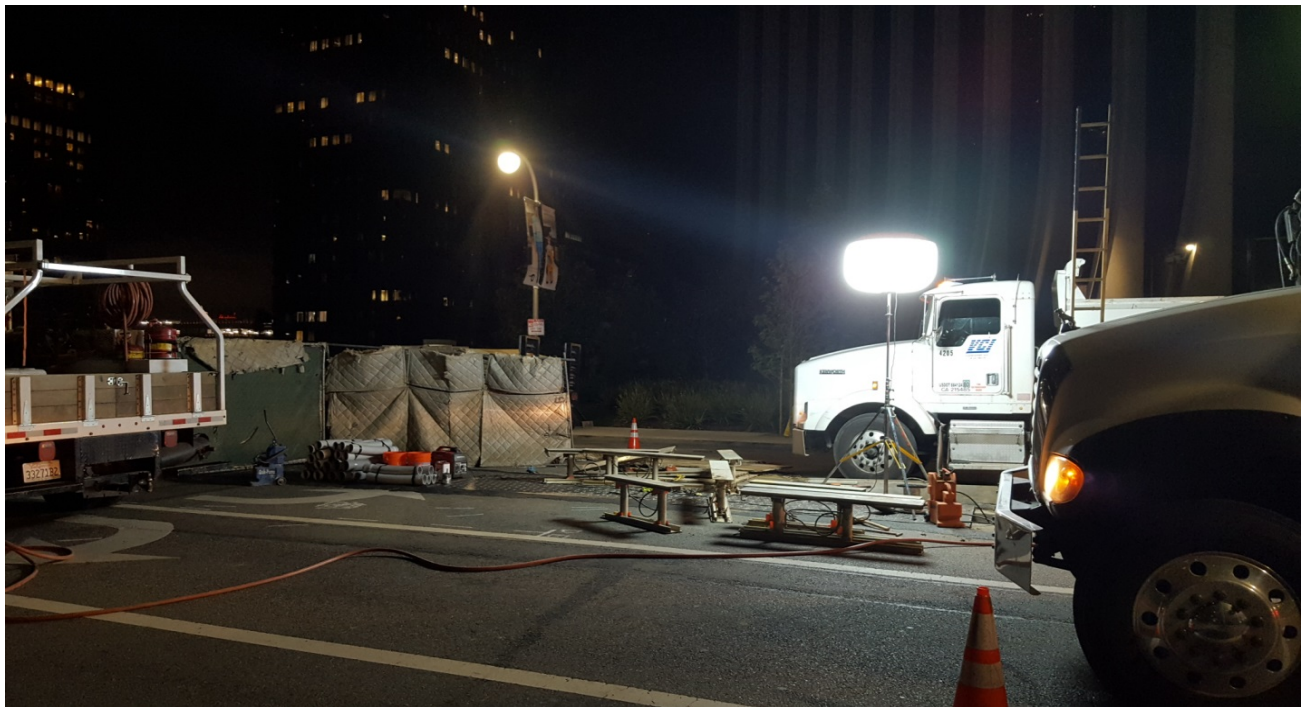
Century City Constellation Joint Trench
