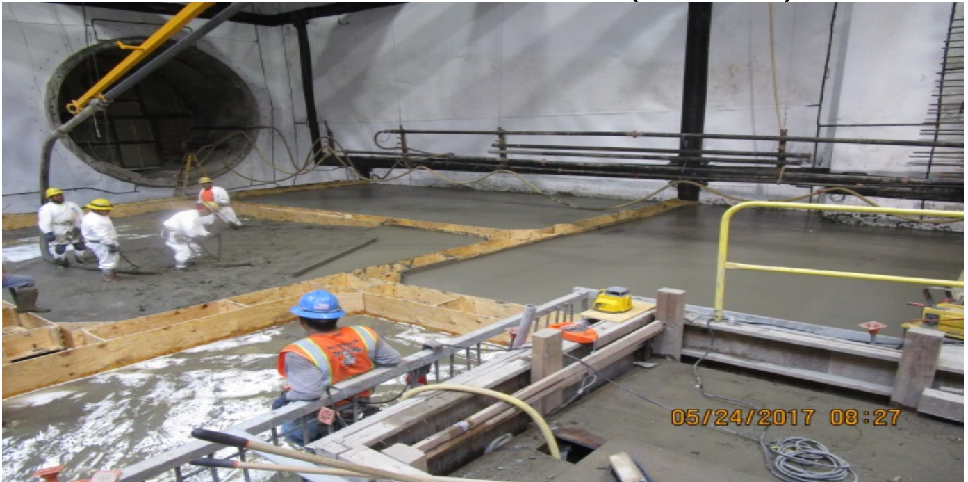
MARTIN LUTHER KING JR. STATION Placement of protection slab at north hammerhead.
