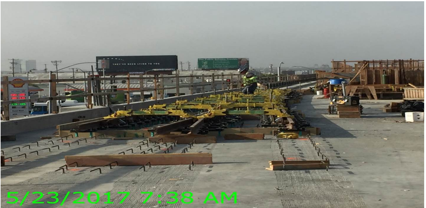
AVIATION/CENTURY BRIDGE – Top down construction of the 10K1 crossover utilizing the Iron Horse system underway at Aviation Century.
