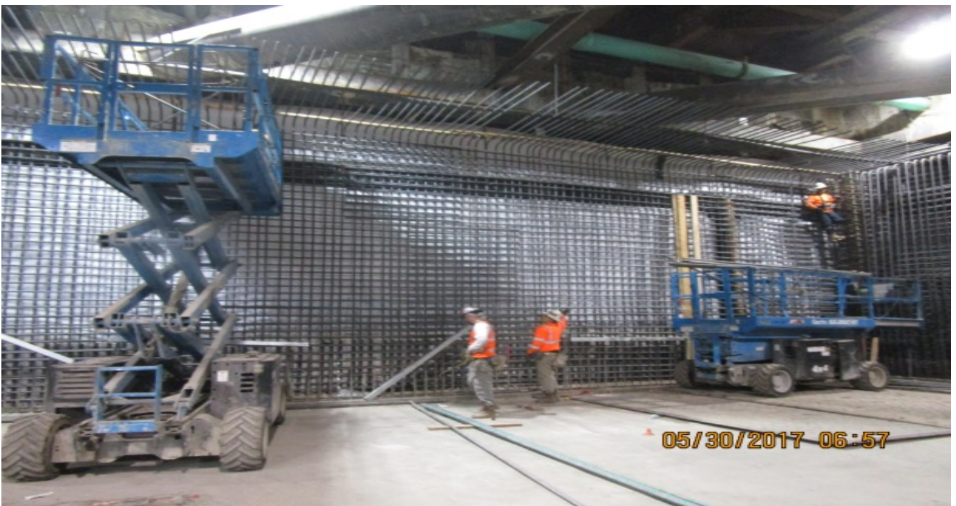
EXPOSITION/CRENSHAW STATION – Installation of rebar for concourse level wall sections G-22 and G-23.
