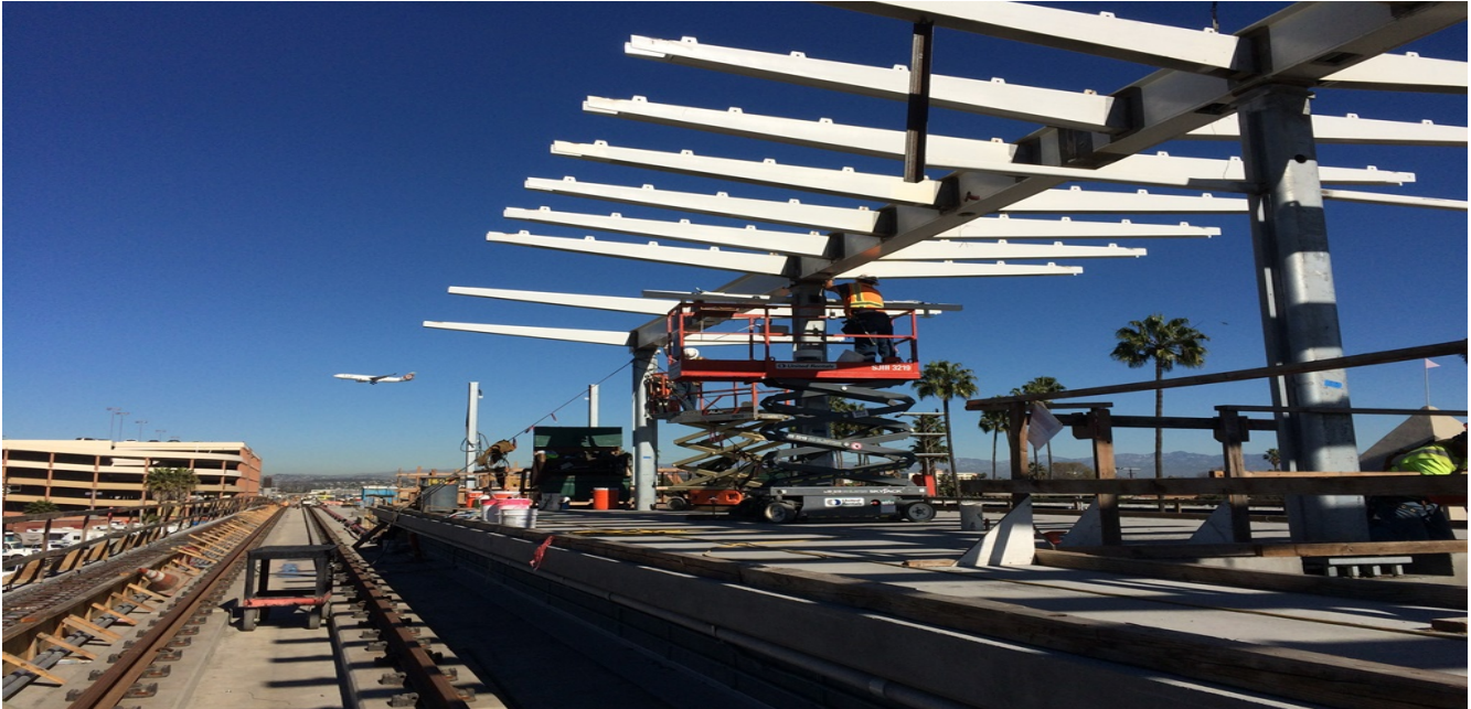
AVIATION/CENTURY BRIDGE – Steel flex conduit and junction box installation in the platform canopy beam assembly.
