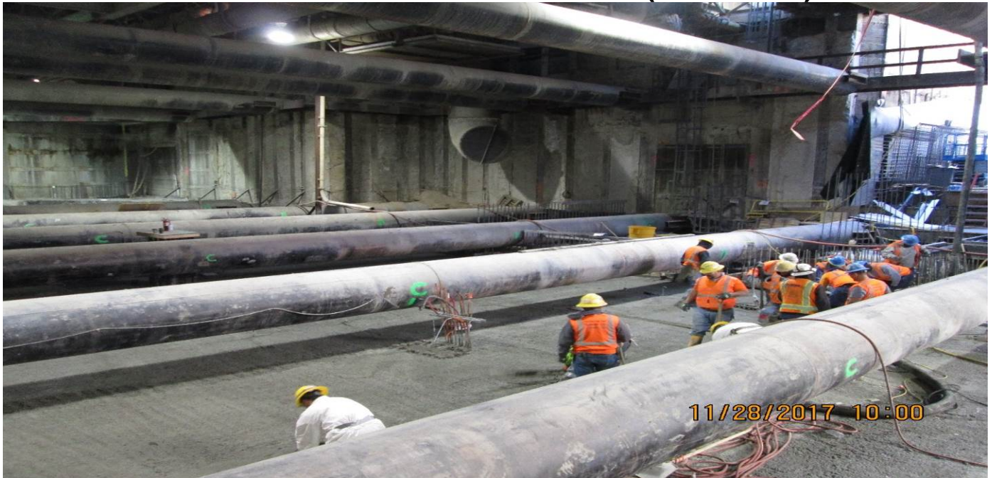
MARTIN LUTHER KING JR. STATION – Placement of concrete for concourse deck section C-2.
