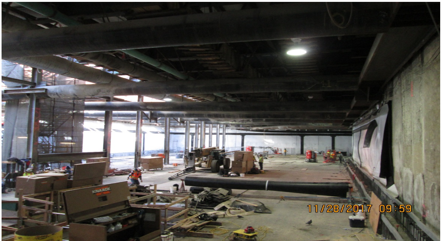
MARTIN LUTHER KING JR. STATION Installation of waterproofing along the north and east concourse level walls.
