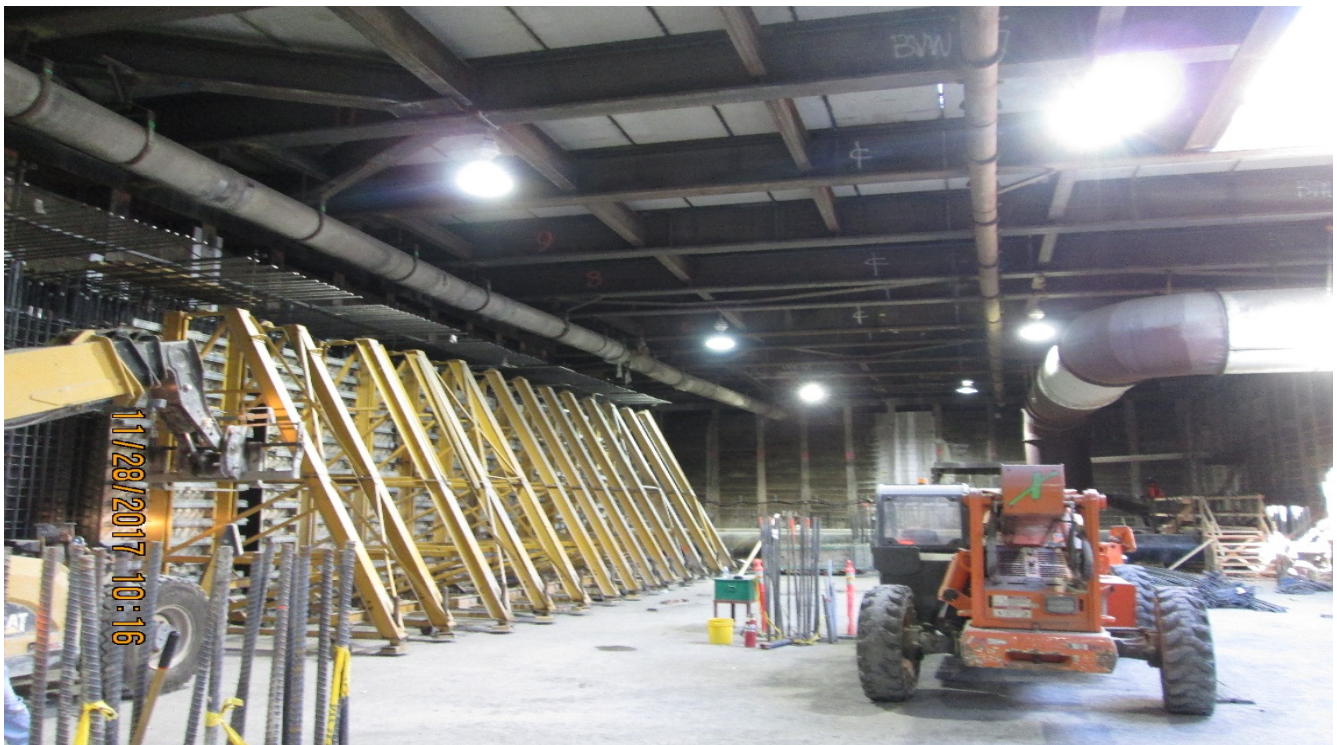
LEIMERT PARK STATION – Removing and installing formwork for west concourse level walls.
