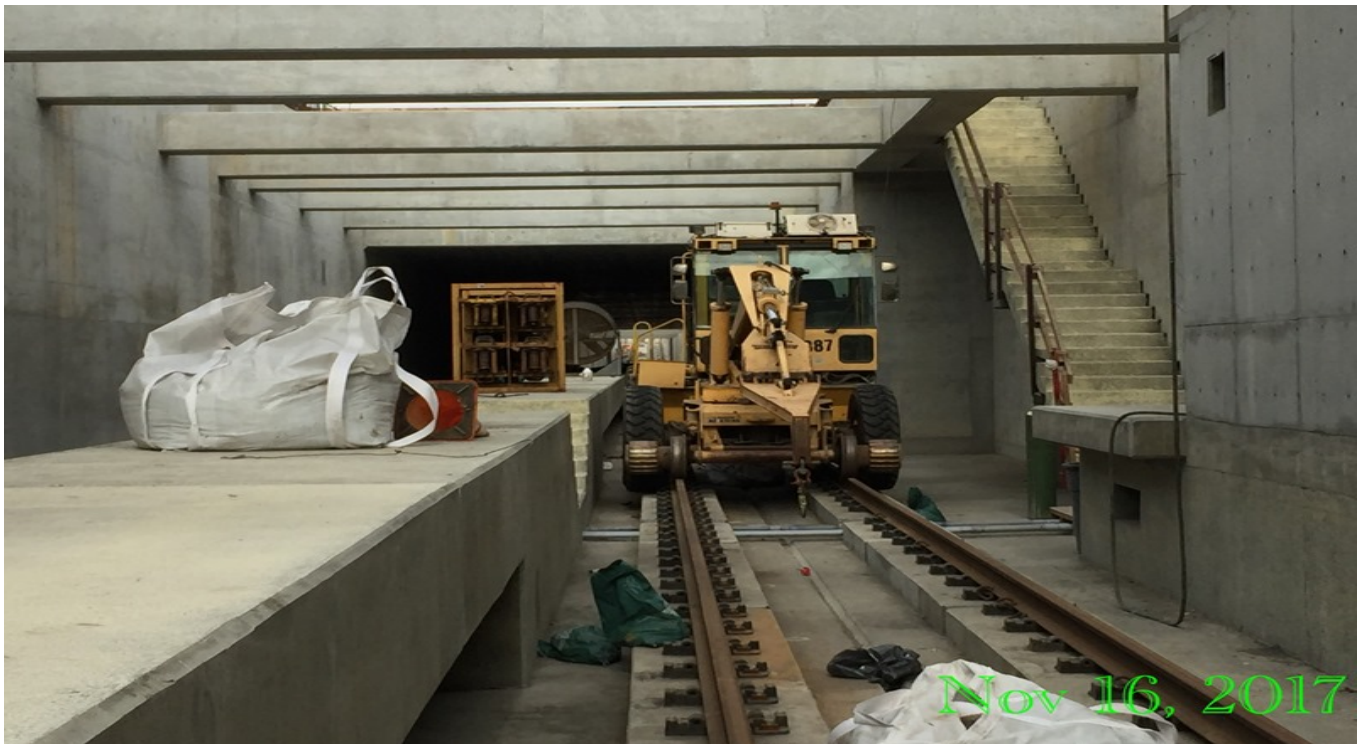
UG1 – Crew continued moving 115# R.E running rail on track-4 NB inside UG-1.
