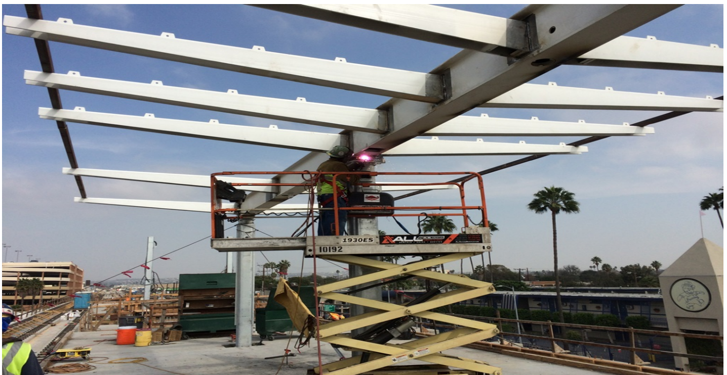
AVIATION/CENTURY BRIDGE -Full penetration weld between the canopy main beam and column in progress.
