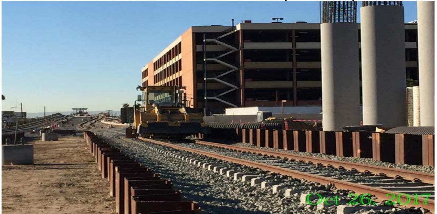
MSE 75L&R – Crew tamping, regulating and surfacing top ballast on track-3 SB from Vitae Street to Century Bridge.
