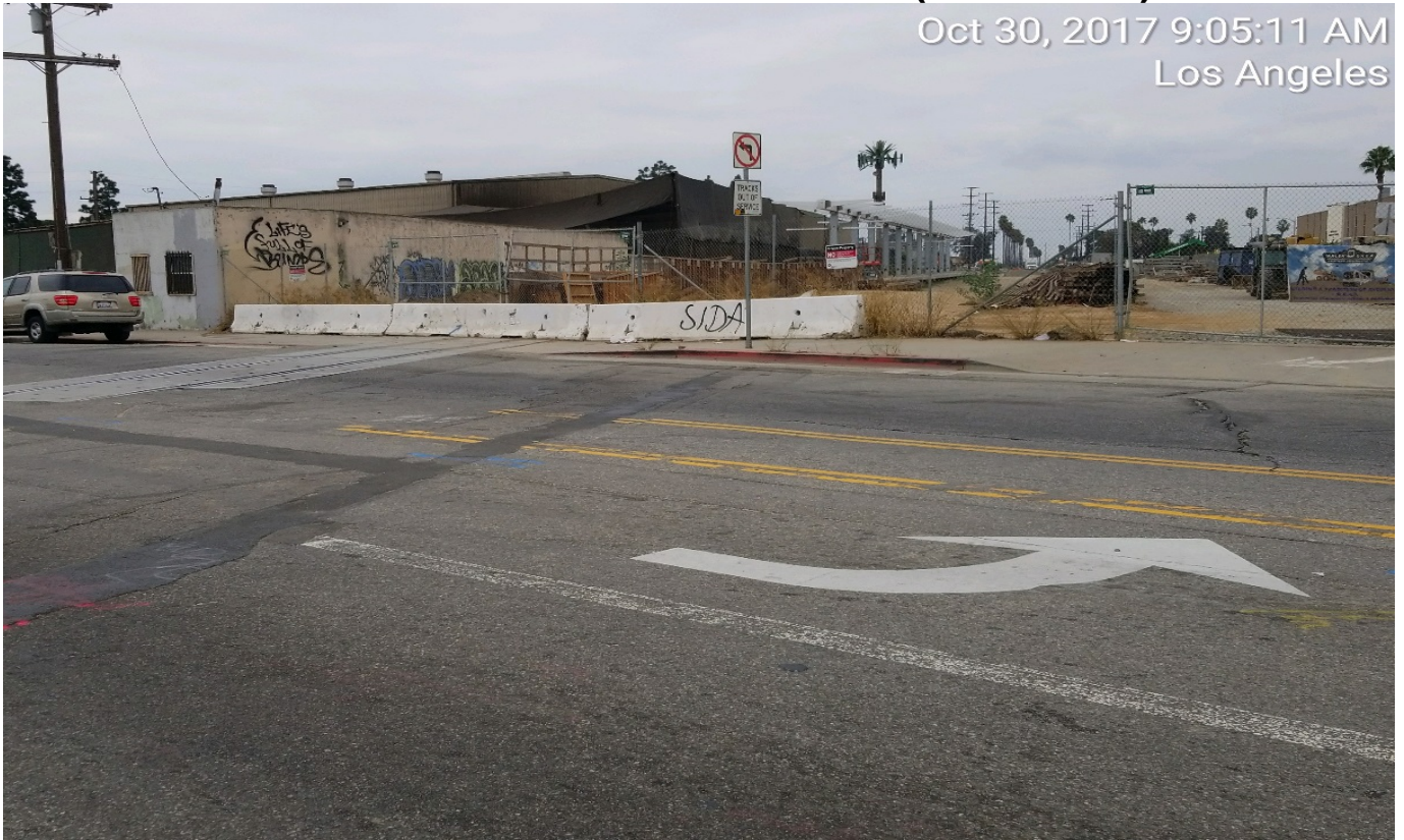
WEST STATION- Canopy erection complete. Outrigger welding underway. Painting of structural steel and installation of canopy catwalks, gutters and glass to follow.
