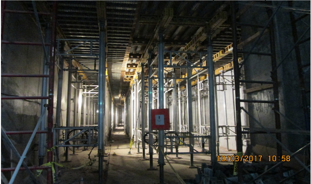
UG4 – Installing false work for roof sections R-28 thru R-25, south of Vernon portal.
