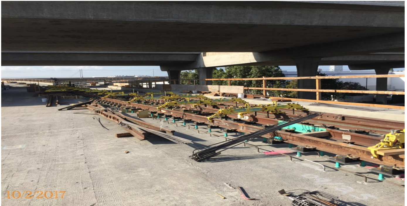
GREENLINE UNDERPASS – Bridge superstructure complete including approach slabs and joint seals. Special track work underway.
