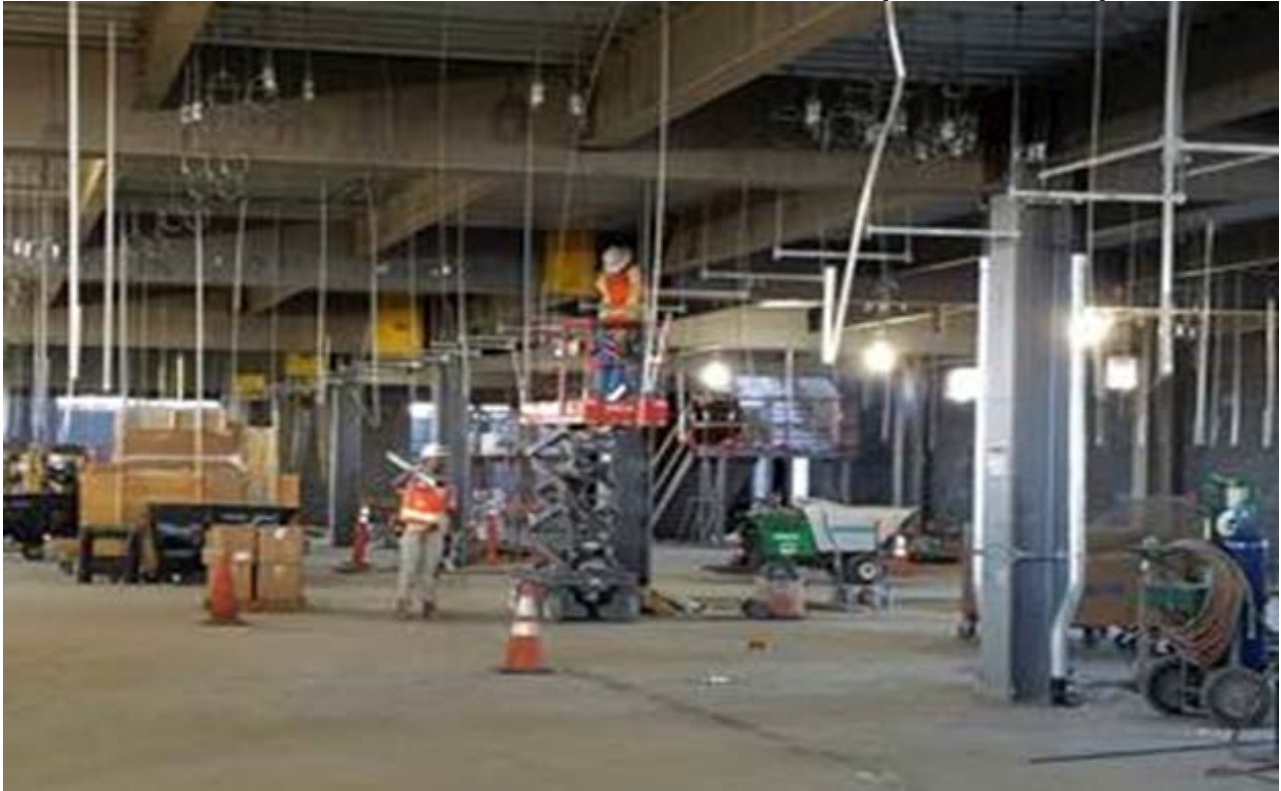
Southwestern Yard - Main shop interior electrical, plumbing and mechanical.
