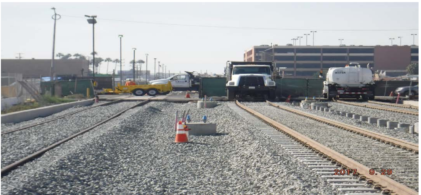
ARBOR VITAE GRADE CROSSING – Crews completed the Arbor Vitae grade crossing on 09.17.17.
