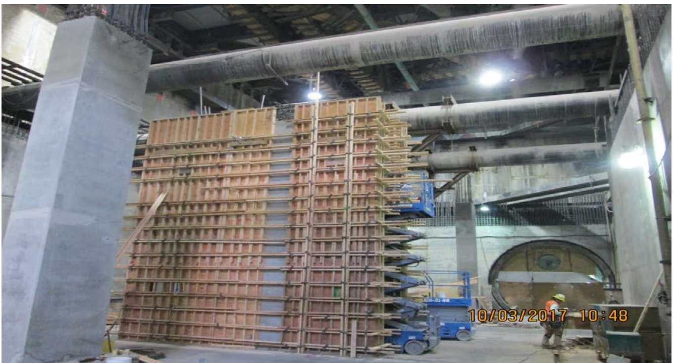
MARTIN LUTHER KING JR. STATION – Installing formwork for south emergency exit stair 1.
