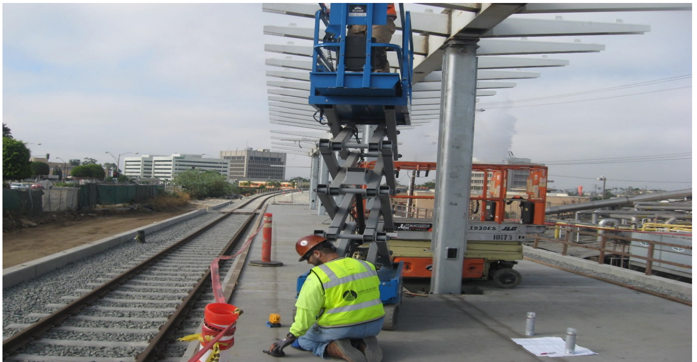
LA BREA AT GRADE STATION - Crews completed canopy outrigger welding and electrical and plumbing installations. Painting of structural steel and installation of canopy catwalks, gutters and glass panels to follow.
