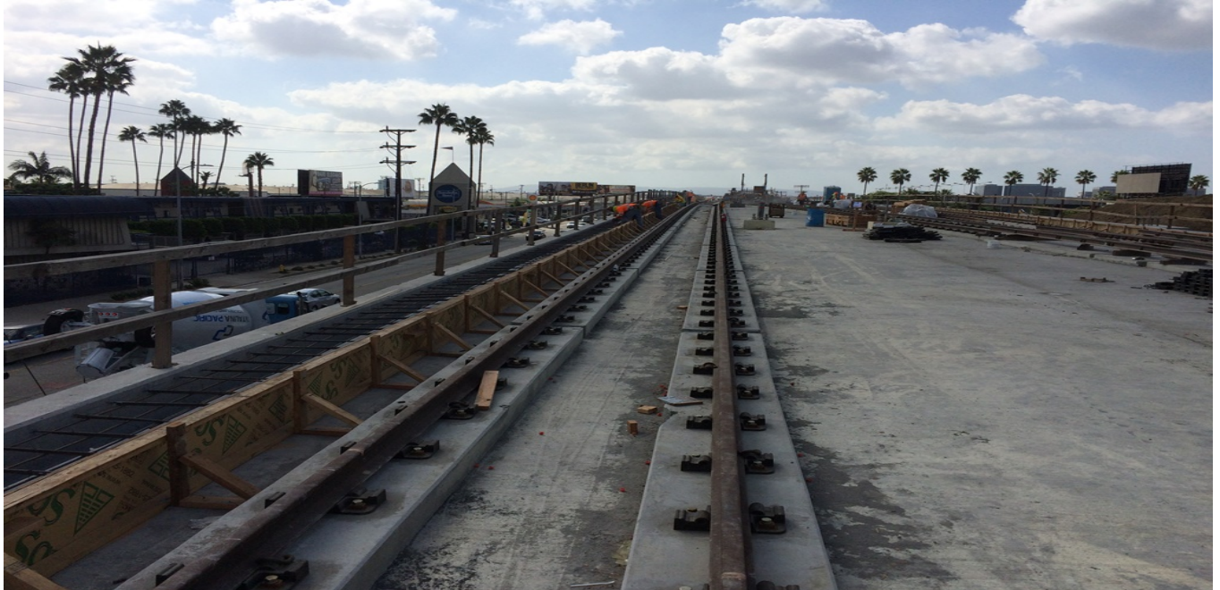
AVIATION/CENTURY BRIDGE – Northbound emergency walkway duct bank on the bridge deck.
