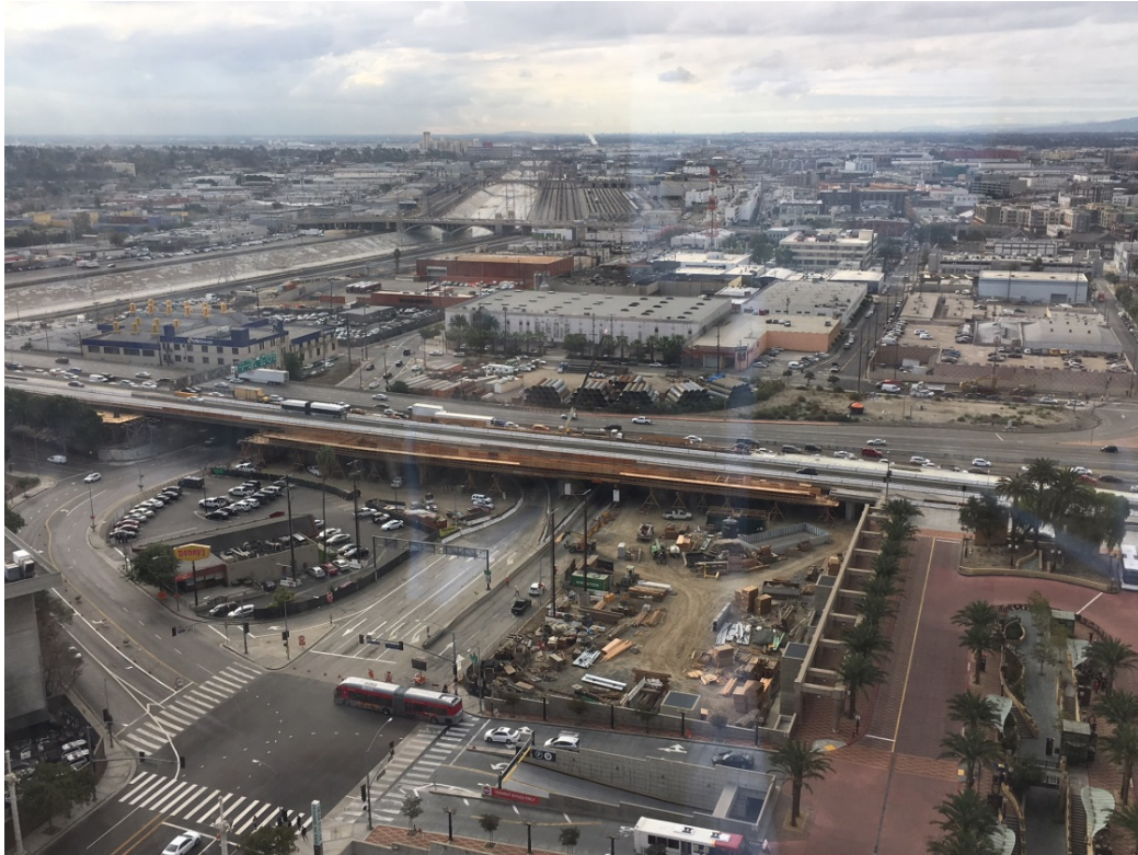
Photo provides an aerial view of the jobsite from the south side of the Metro Gateway Building.
