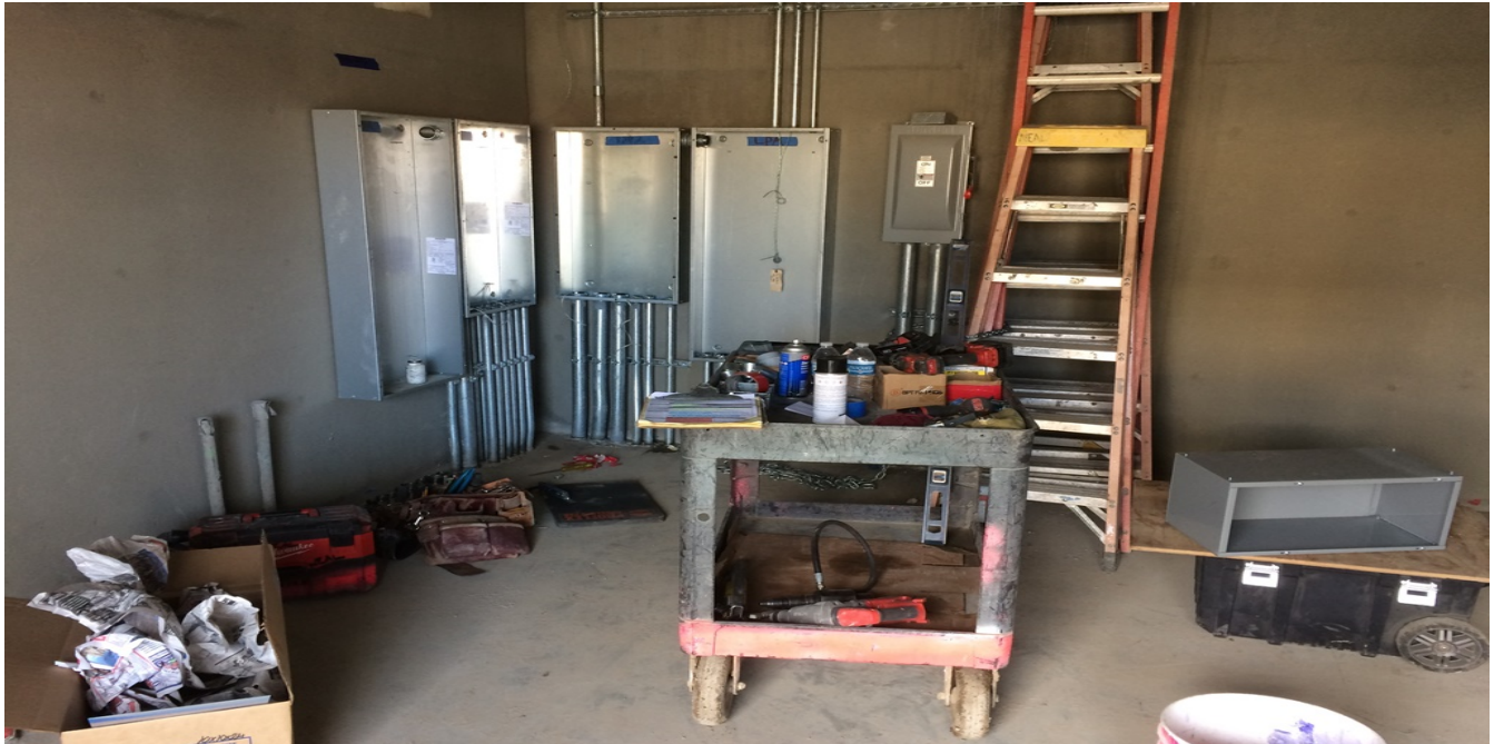
AVIATION/CENTURY BRIDGE – Panels PPA, PPC, LCPA and LPA installed in the Service Building Electrical Room.
