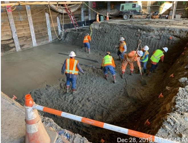
Dec 28, 2018 5:19:44 AM West Cable Room mud slab at Track Level at Central in future Little Tokyo/Arts District Station
