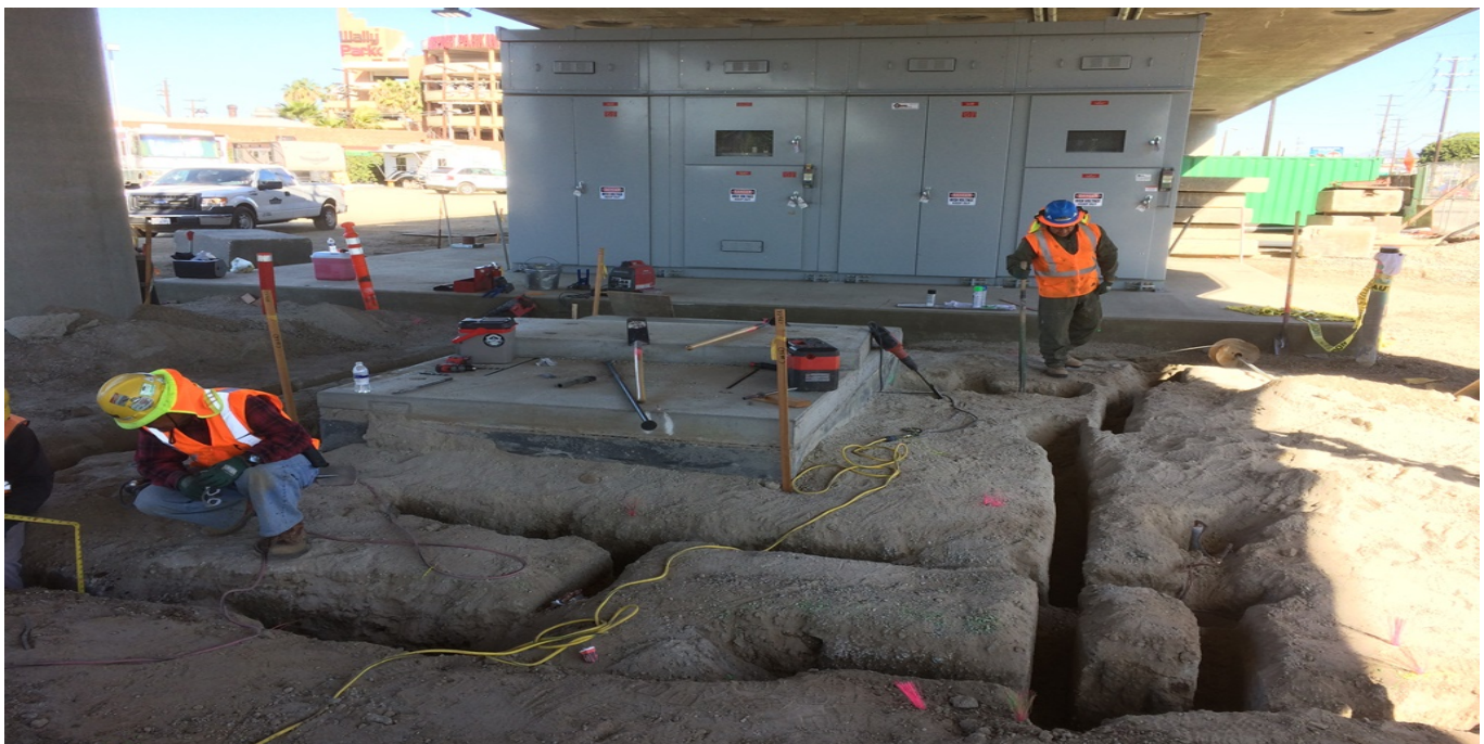
TPSS - TPSS 2. Trench excavation and installation of copper cable for the grounding grid around the DWP Disconnect Switch and Pullbox.
