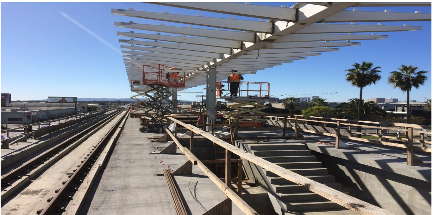
AVIATION/CENTURY STATION – Painting the exposed steel on the platform canopy columns and beams.
