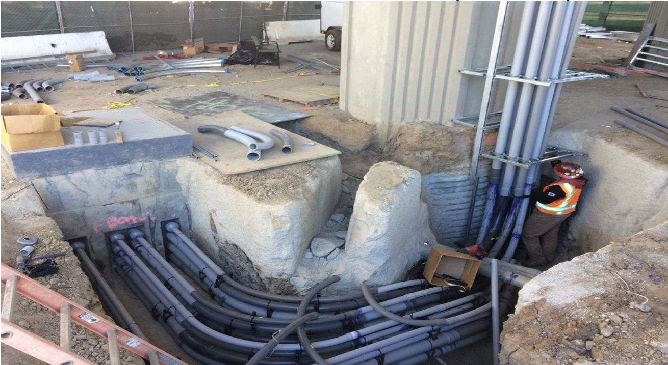
TPSS - TPSS 1. Ductbank and riser conduit installation from MH-COM-013B to the Bent 3W column.
