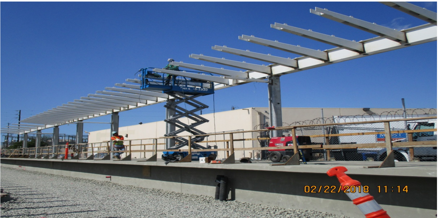
WESTCHESTER STATION -Removal and placement of steel tabs at NB and SB outriggers.
