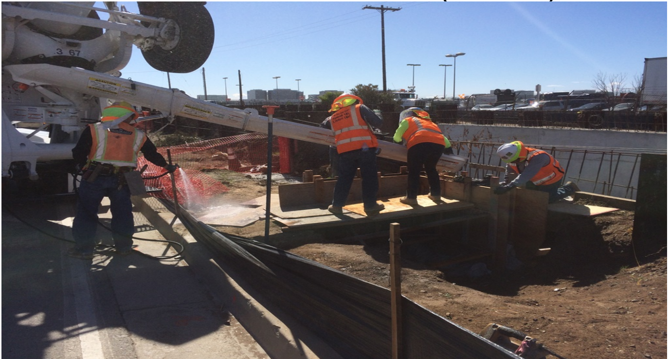
UG1 – Concrete placement at the storm drain line P-200A Headwall NB STA.
