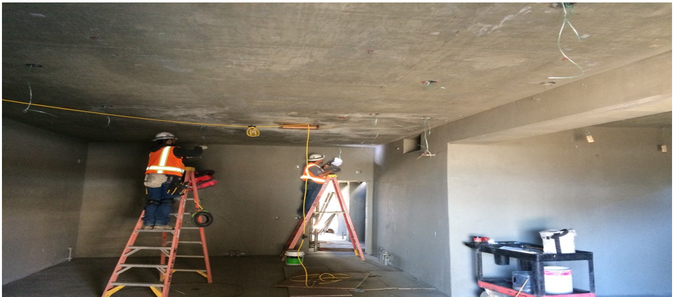
Aviation/Century Bridge – Pulling string and labeling conduit in the service building TC&C.
