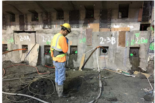
Second post grouting at second level underpinning panel tie-backs related to Historic Broadway Station
