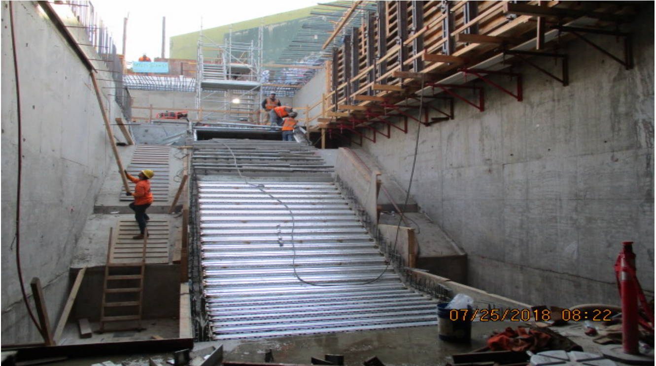
LEIMERT PARK STATION – Installation of anchors for the metal ceiling system above the platform.
