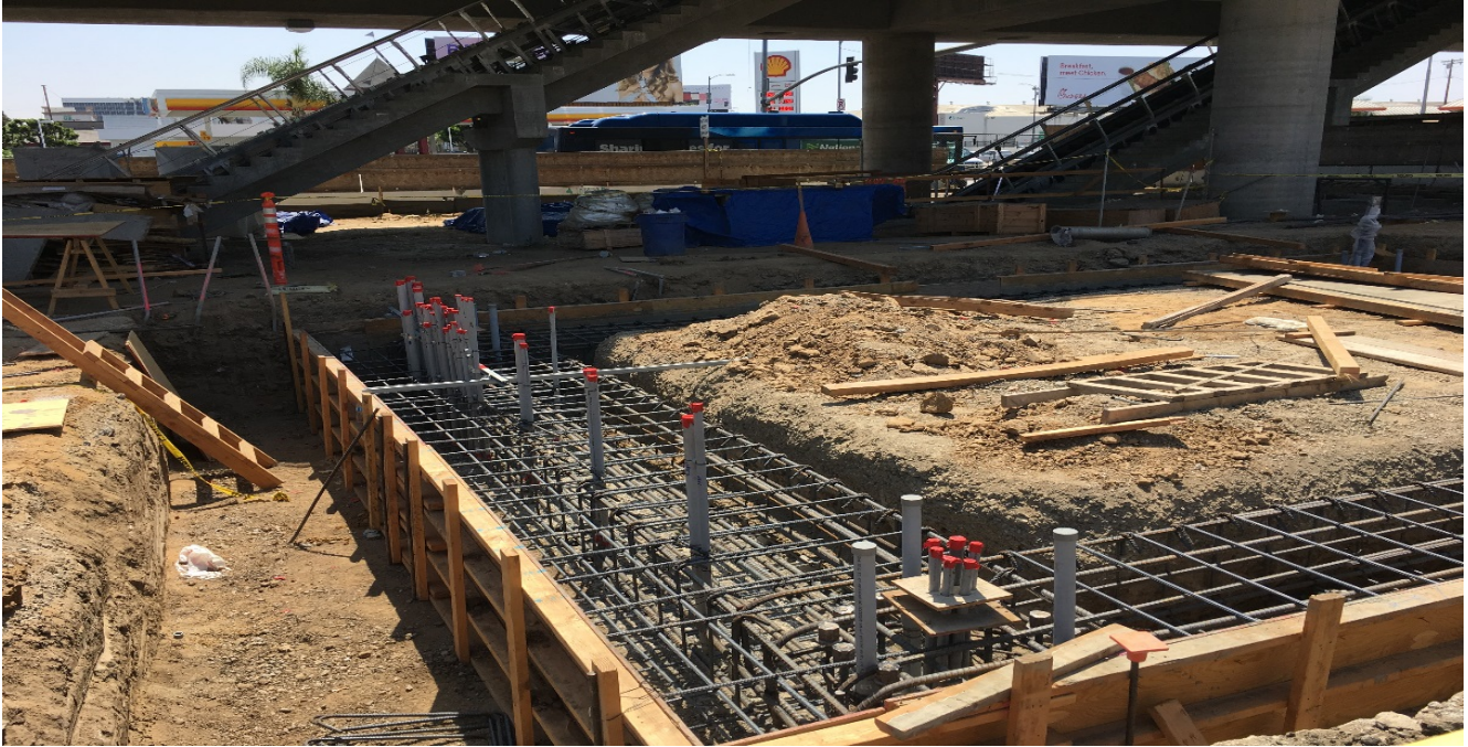
AVIATION/CENTURY STATION - All PVS Stubs have been raised above the pour line for the forms for the TVM's.
