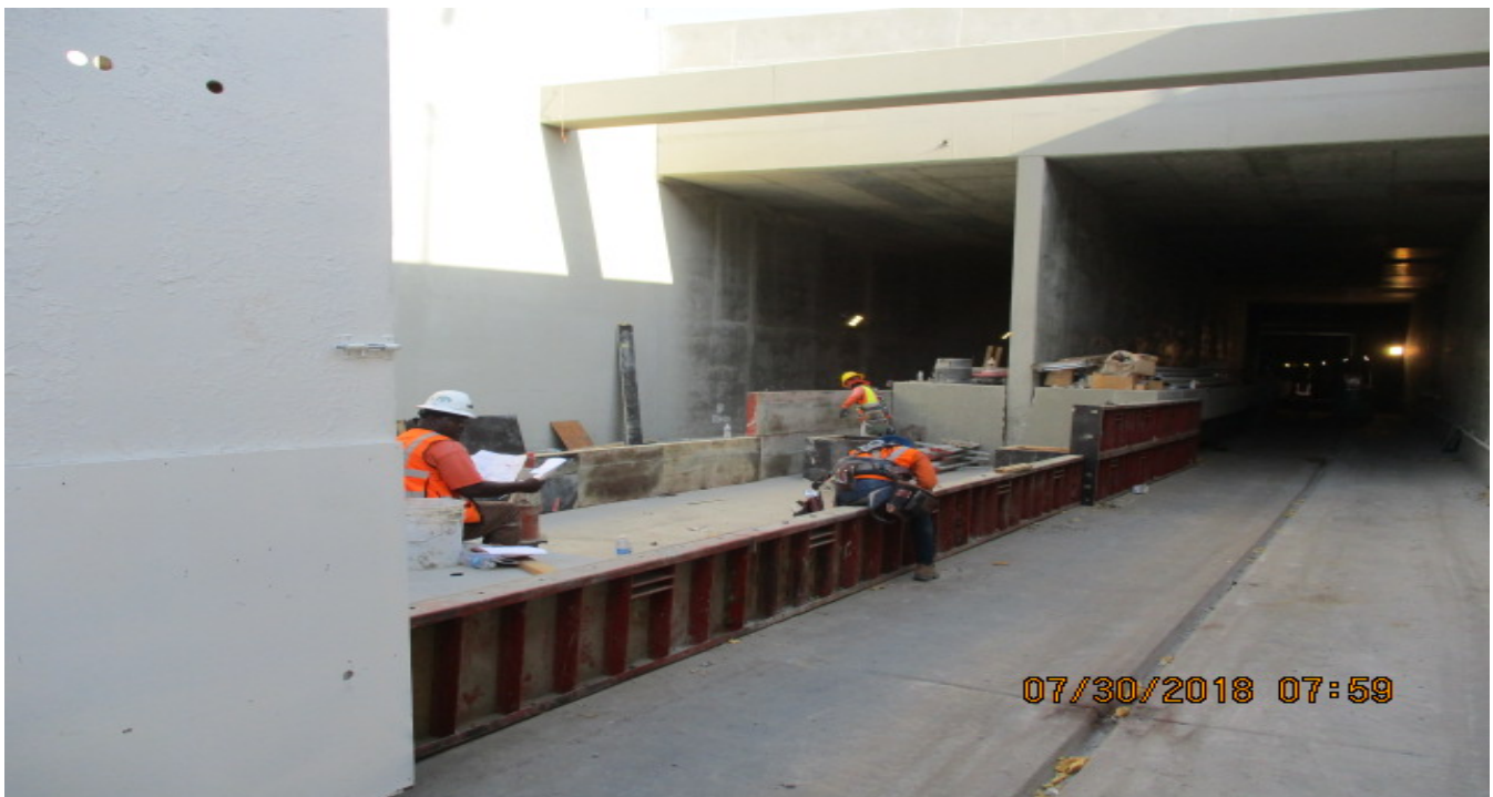
UG4 – Formwork for the remaining section of the emergency walkway at the south portal
