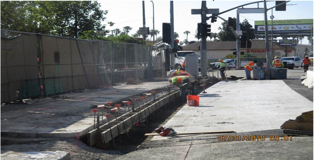
UG4/VERNON RESTORATION – Formwork for east curb and gutter between 43rd street and Vernon.
