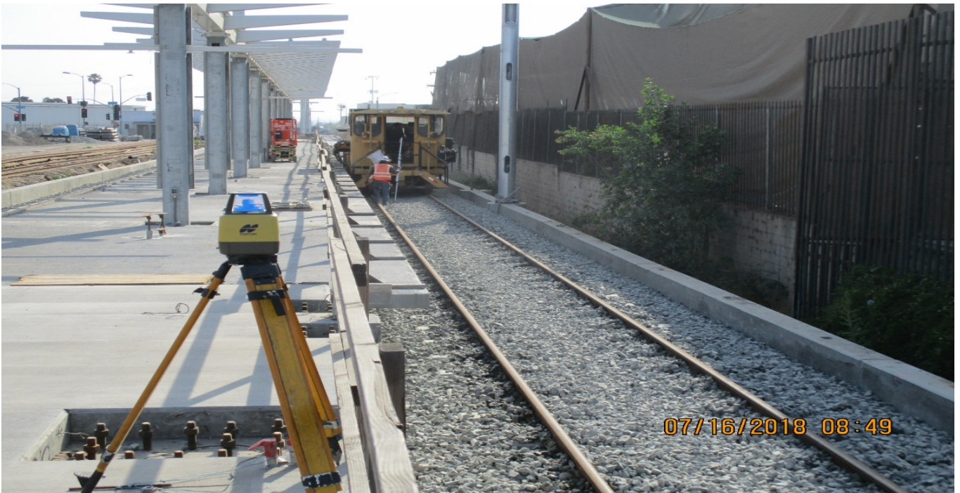
FAIRVIEW HEIGHTS STATION - Track 4 tamping and ballast regulating at the Fairview Heights Station.
