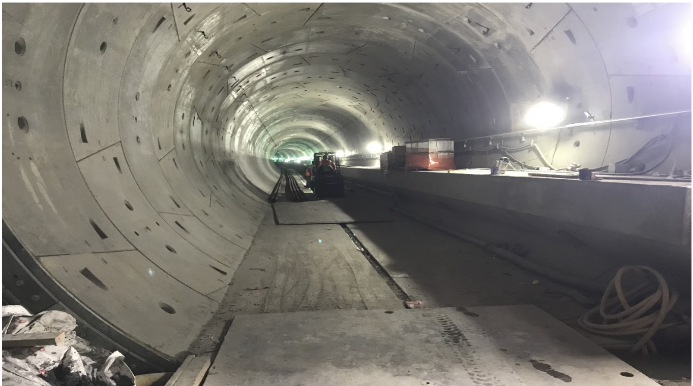
TUNNEL – SB tunnel to Vernon station at the south end of MLK station.
