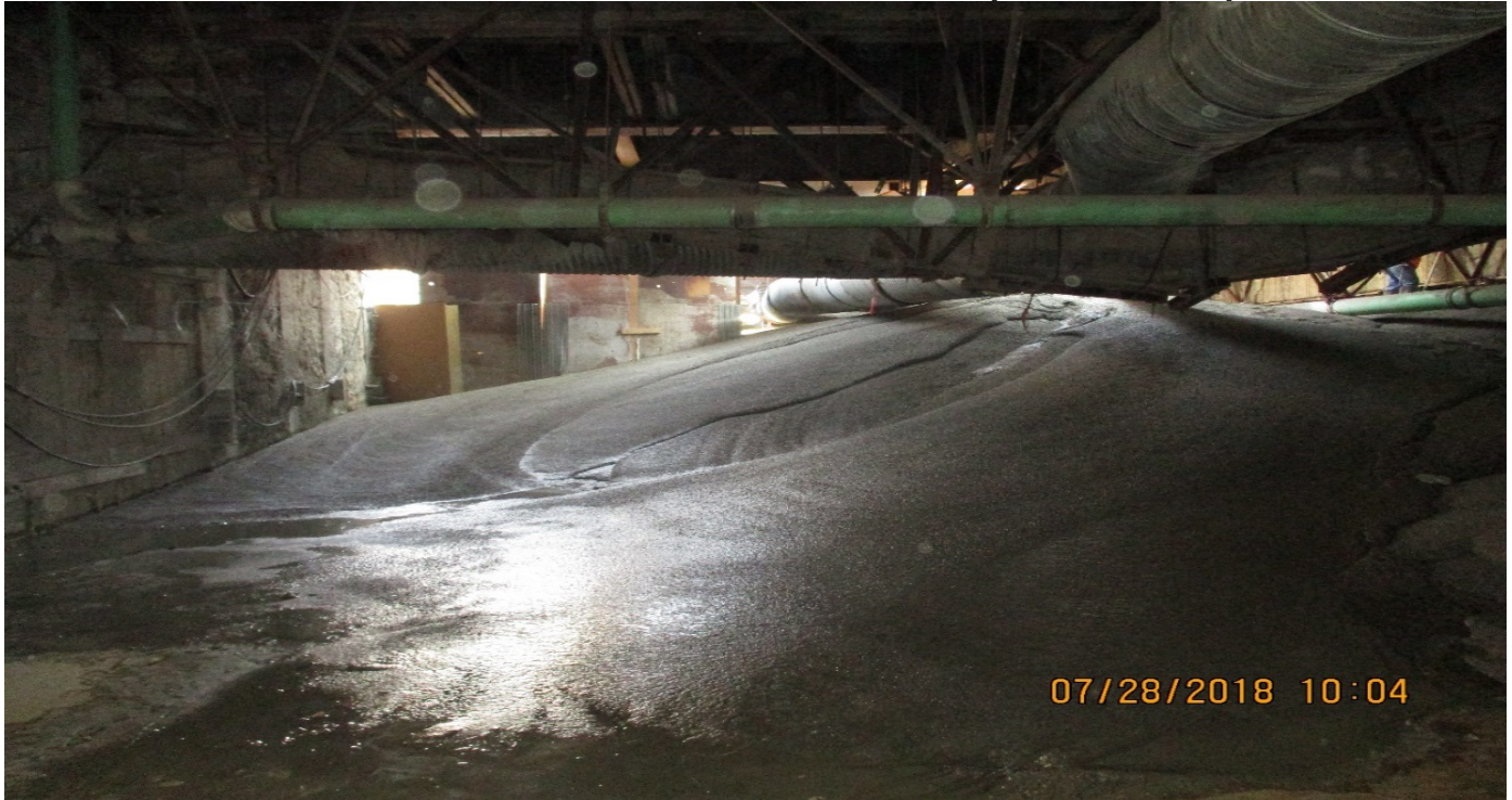
MARTIN LUTHER KING JR. STATION- Slurry backfill underneath utilities at the roof.
