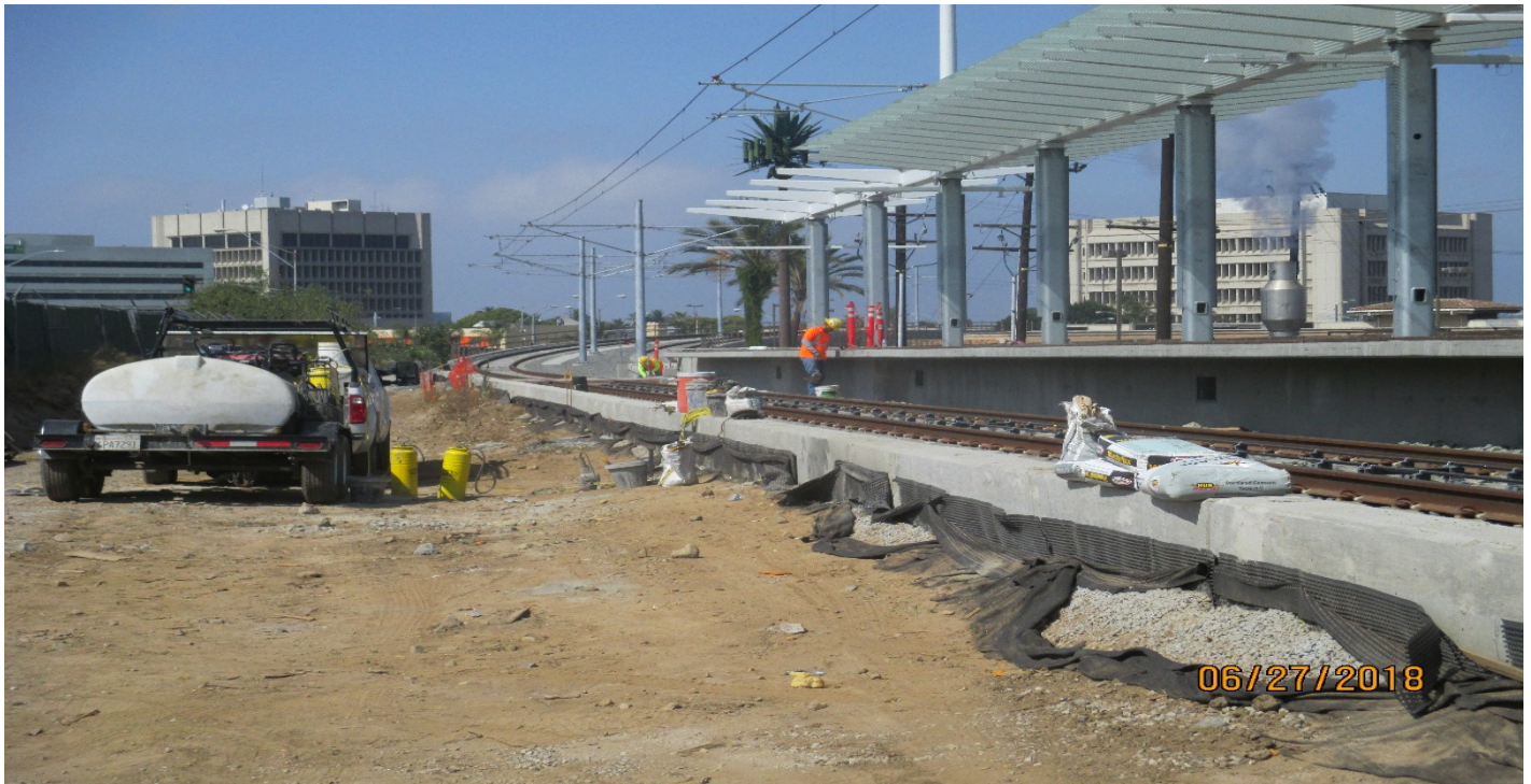
LA BREA AT- GRADE STATION – Working on the concrete finish for the La Brea Station platform.
