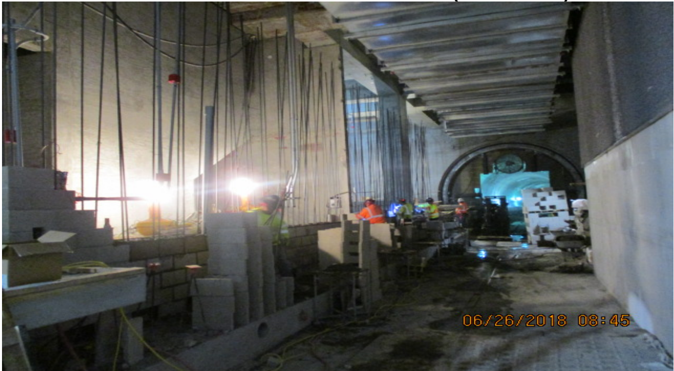
LEIMERT PARK STATION – Installation of platform level CMU walls at the north back of house.
