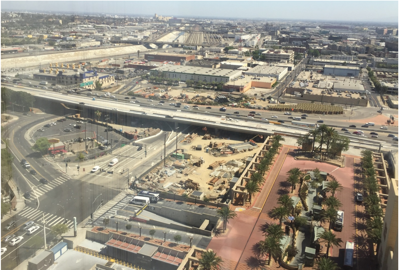
Photo taken from the south side of the Metro Gateway Building provides an aerial view of the jobsite.
