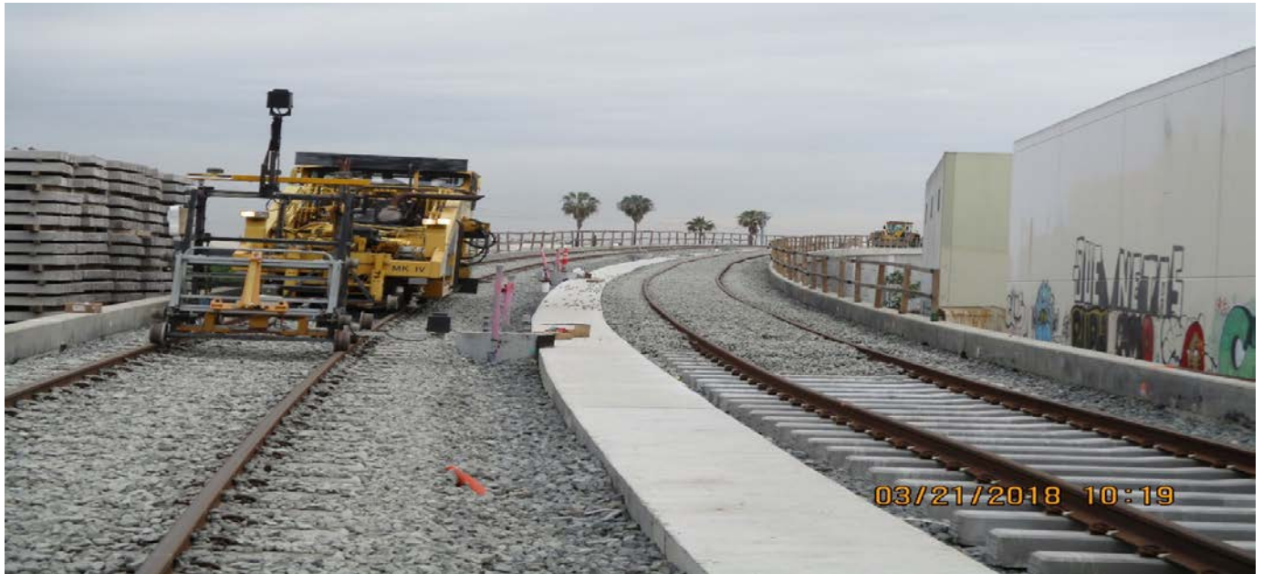
(AG-4) MANCHESTER BRIDGE – Tamping of SB track and flooding of ballast rock along NB track.
