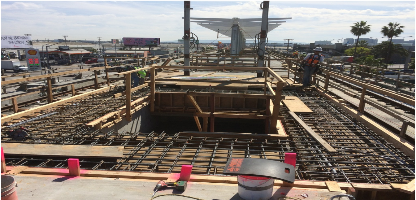
AVIATION/CENTURY STATION – Station platform overhang formwork installation at the Service Building Exit Corridor staircase.
