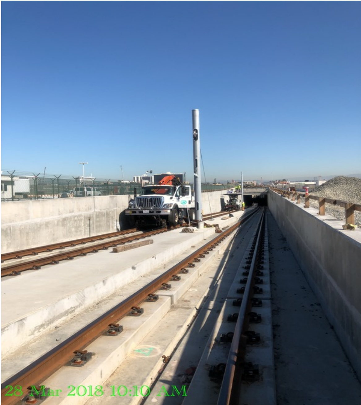
UG1 – Installation of counter weight balance and down guy cable inside the OCS pole Str. 1028 and 1029.
