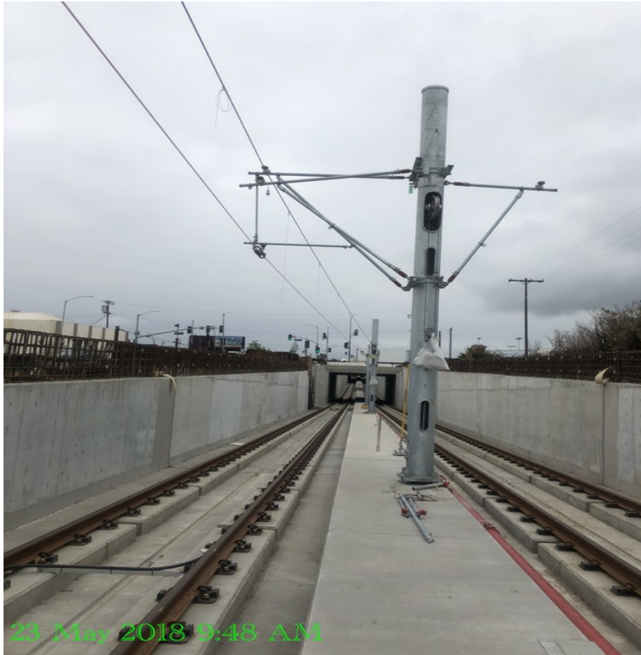
UG1 – track work and overhead catenary system.
