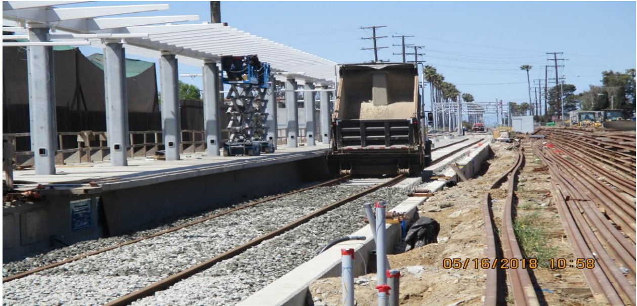
FAIRVIEW HEIGHTS STATION- top ballast rock speading along southbound track.
