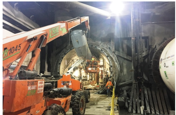
Wilshire/La Brea Station – Hanging Ventilation
