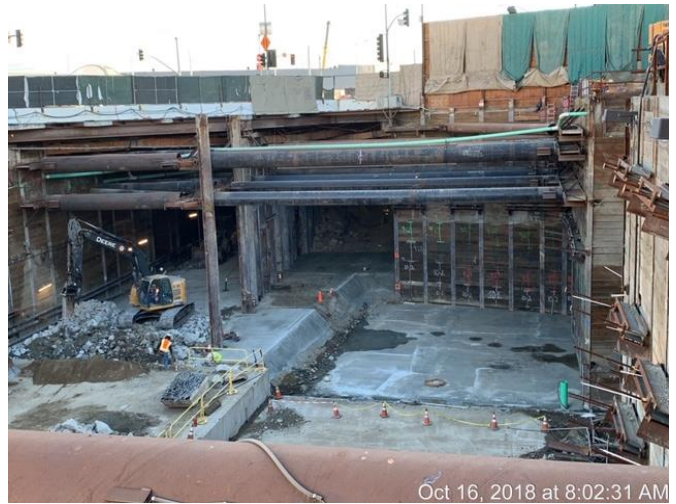
Installation of mud slab at track level in the future Little Tokyo/Arts District Station
