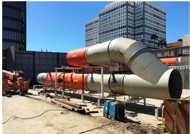
Ventilation Ducts at Wilshire/La Cienega Station
