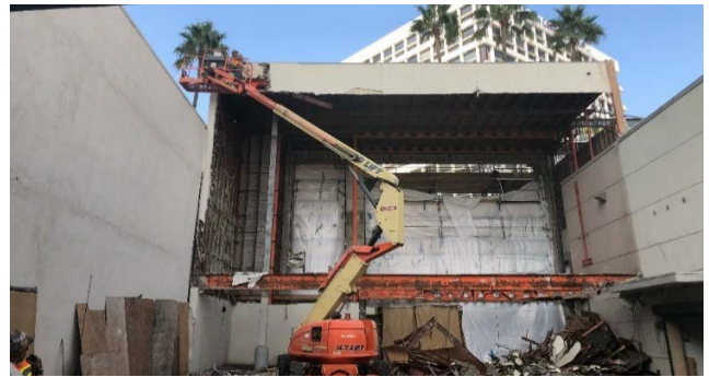
Roof Wall Removal of Former Ace Gallery in Beverly Hills at Future Station Entrance
