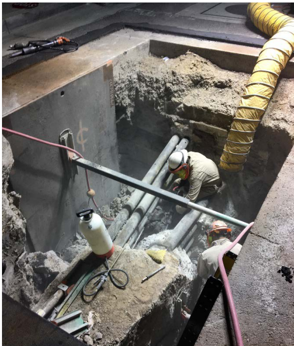
DWP Power Ductbank in Century City
