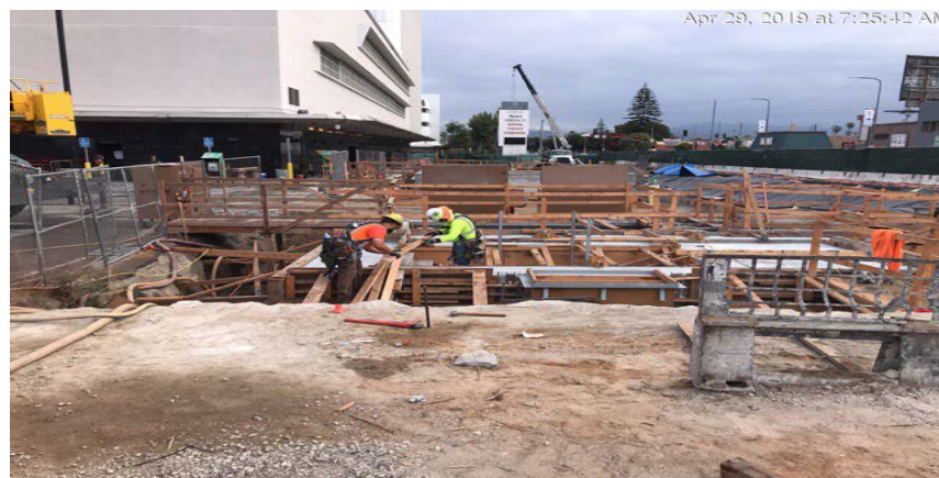
Construction of the ramp and entrance to Emergency Exit 2 south for Martin Luther King Jr. Station.
