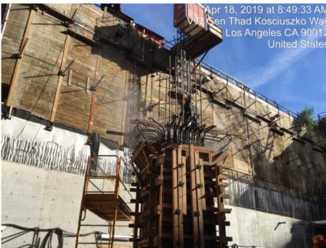
Concrete placement at Concourse Level column at Grand Av Arts/Bunker Hill Station
