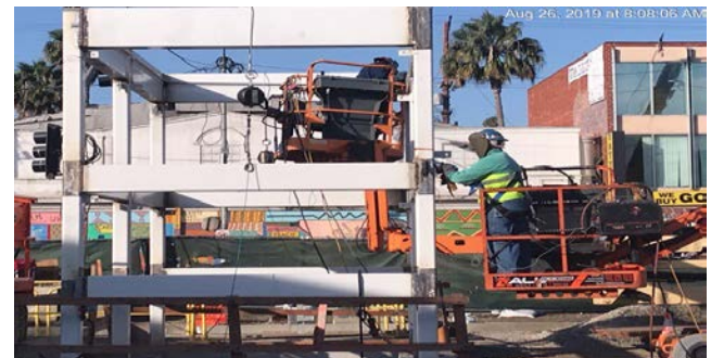
LEIMERT PARK STATION – Continued installation of entrance canopy steel for Elevator 1 and 2 at street level.
