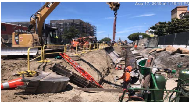
UG STRUCTURE #3 - Continued removal of beams northbound/southbound piles at 63 rd and Crenshaw Blvd.
