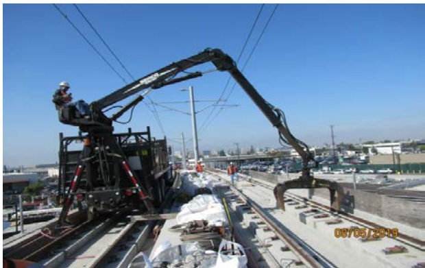
MANCHESTER BRIDGE – Grapple truck moving rail into place for plinth repair work.
