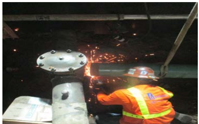
Southern California Gas Welding Connection Joint at the Intersection of Veteran Ave. and Wilshire Blvd.
