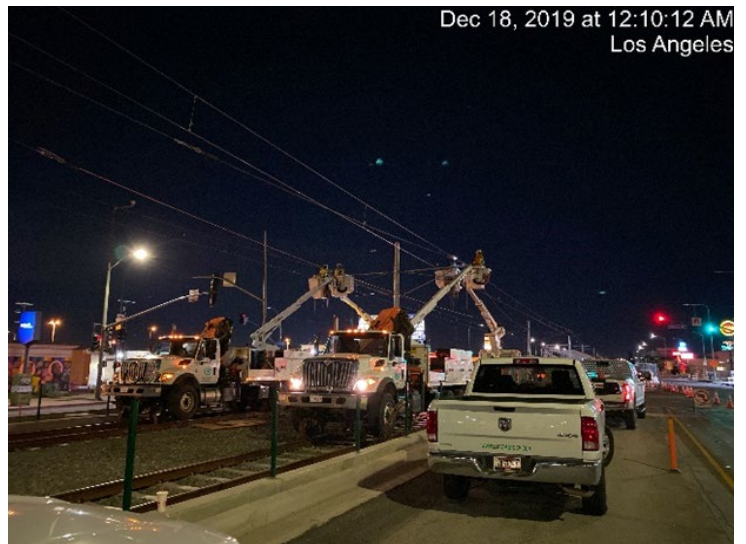
12 PARK MESA – adjusting overhead contact system wire, installing overhead contact rail at Slauson Ave and Crenshaw Blvd.
