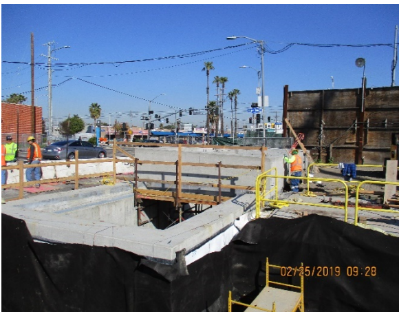
Expo Station - north plaza ventilation shaft room
