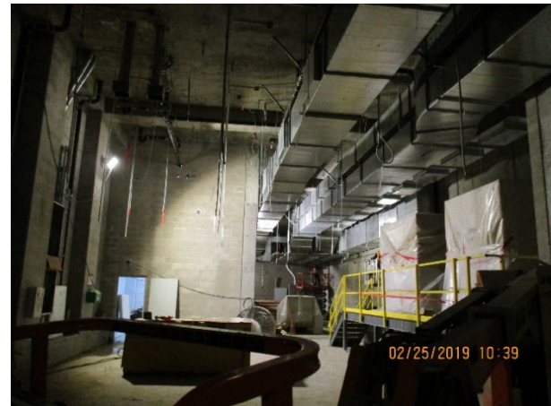
Martin Luther King Jr. Station - Traction Power
